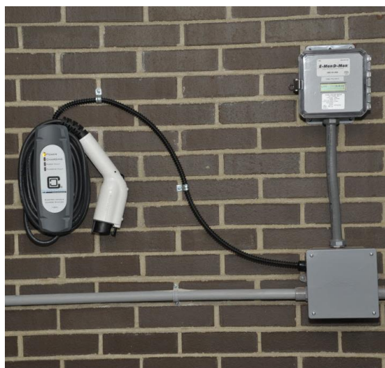
Wall-mounted Level 1 EVSE used for workplace charging (New York Power Authority Photo)
