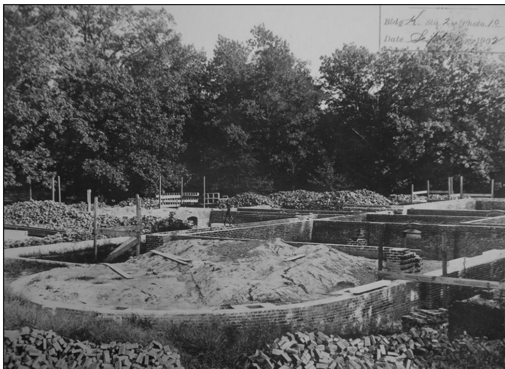
Figure 6.4. Foundation for Building K under construction, September 1902. (National Archives RG 48 Entry 300 Box 6)
