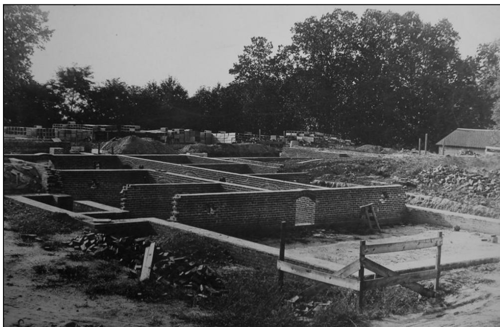
Figure 6.5. Foundation for Building J under construction, September 1902. (National Archives RG 48 Entry 300 Box 6)
