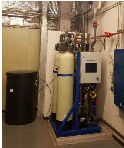
Figure 3: PWS system installed at the Lloyd D. George U.S. Courthouse
