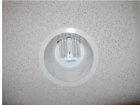
Dallas, TX and Philadelphia, PA 8" aperture Horizontally oriented 2-lamp, 4' on-center
