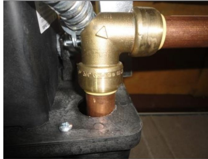
Copper pipe replaces PVC but booster condensate pumps not monitored
