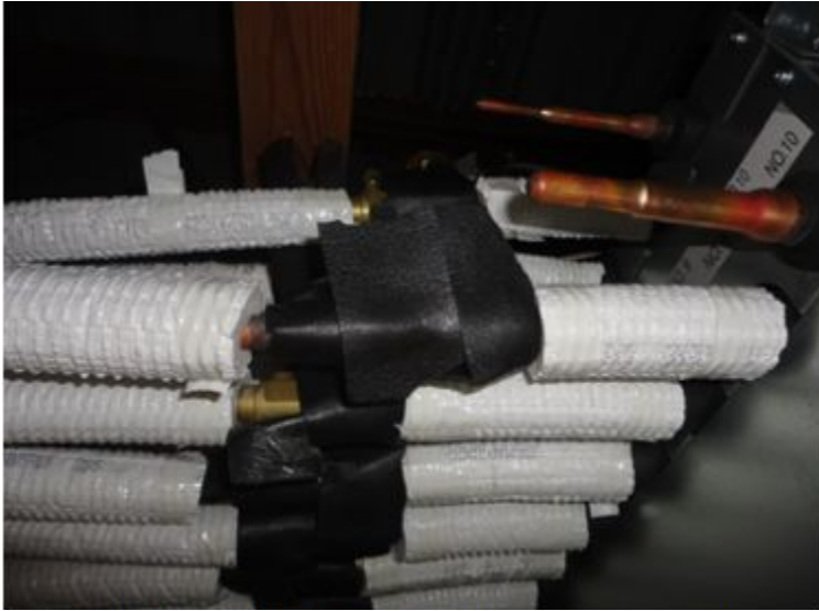
Note lack of continuous insulation
