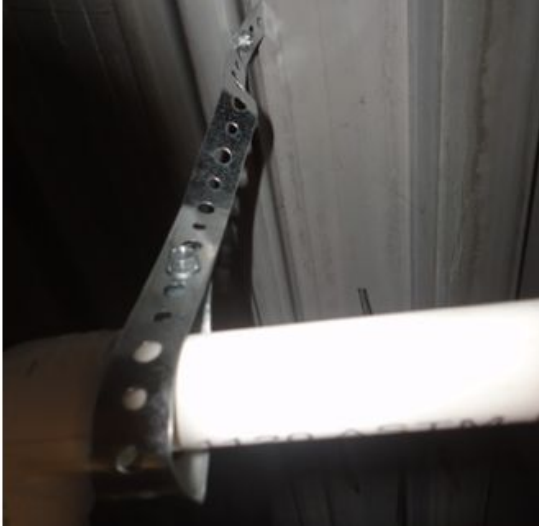
PVC pipe condensate installed with loosely installed metal strap
