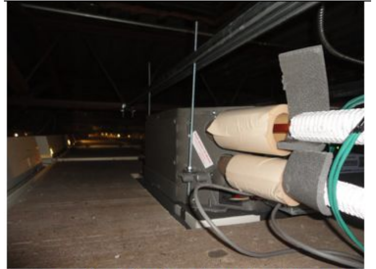
Lack of continuous insulation on refrigerant line
