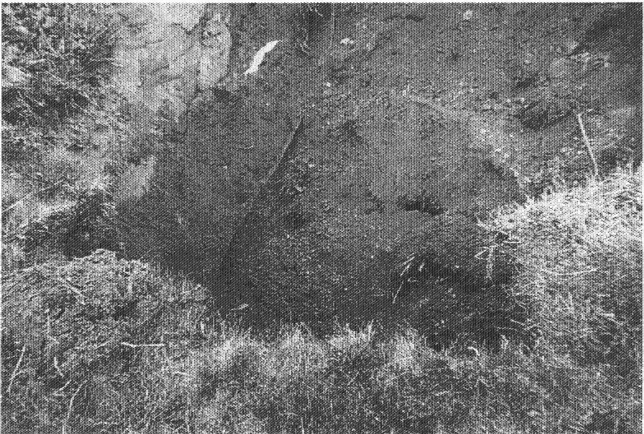
Photograph No.: 4 Contract No.: DACW31-95-D-0097 Earth Tech Job No.: 21574 Project Name: Pedricktown U.S. Army Reserve Center D.O. 0015 Photographer: D. Mothershead Date: 5/13/97 Description: Excavation after removal of UST No. 235-1 at Building No. 235. Direction: North.
