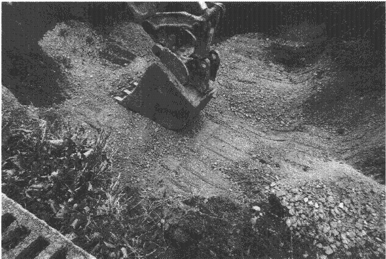
Photograph No.: 6 Contract No.: DACW31-95-D-0097 Project Name: Pedricktown U.S. Army Reserve Center Photographer: D. Mothershead Description: Backfilling of tank excavation at Building No. 235.
