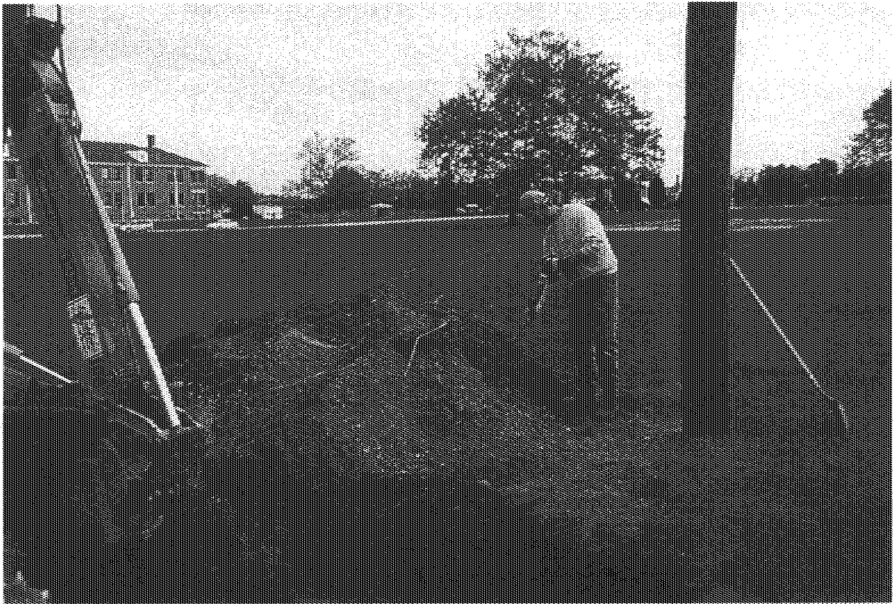
Photograph No.: 5 Contract No.: DACW31-95-D-0097 Project Name: Pedricktown U.S. Army Reserve Center Photographer: D. Mothershead Description: Screening of excavated soil at Building No. 235.
