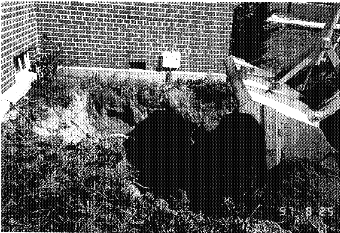
Photograph No.: 3 Contract No.: DACW31-95-D-0097 Location: Pedricktown U.S. Army Reserve Center (Bldg 276S) Photographer: B. Rayfield Description: Excavation was backfilled with clean excavated soil.
