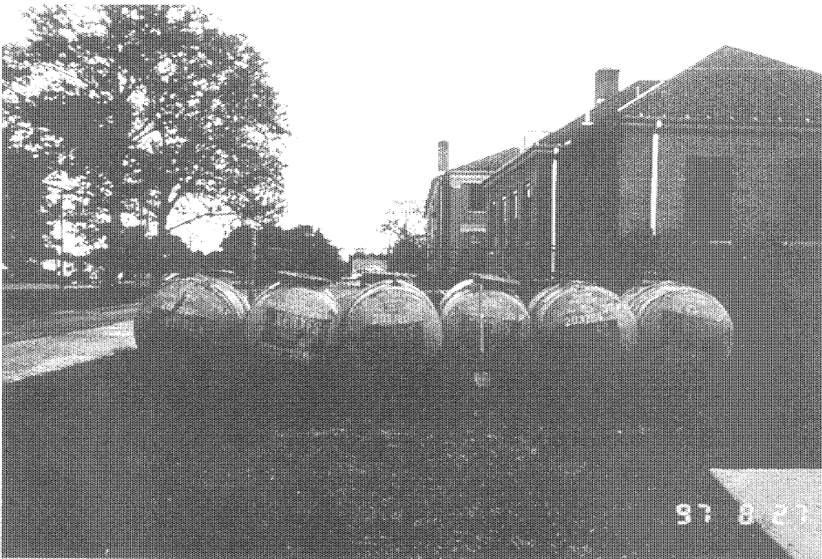
Photograph No.: 2 Contract No.: DACW31-95-D-0097 Location: Pedricktown U.S. Army Reserve Center (Bldg 278S) Photographer: B. Rayfield Description: Tank removed and staged for cleaning.
