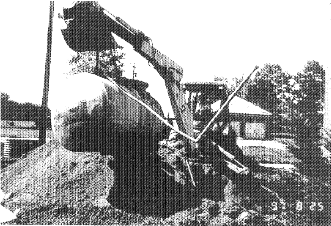
Photograph No.: 2 Contract No.: DACW31-95-D-0097 Location: Pedricktown U.S. Army Reserve Center (Bldg 276S) Photographer: B. Rayfield Description: 550-gallon UST and associated piping were removed from excavation.
