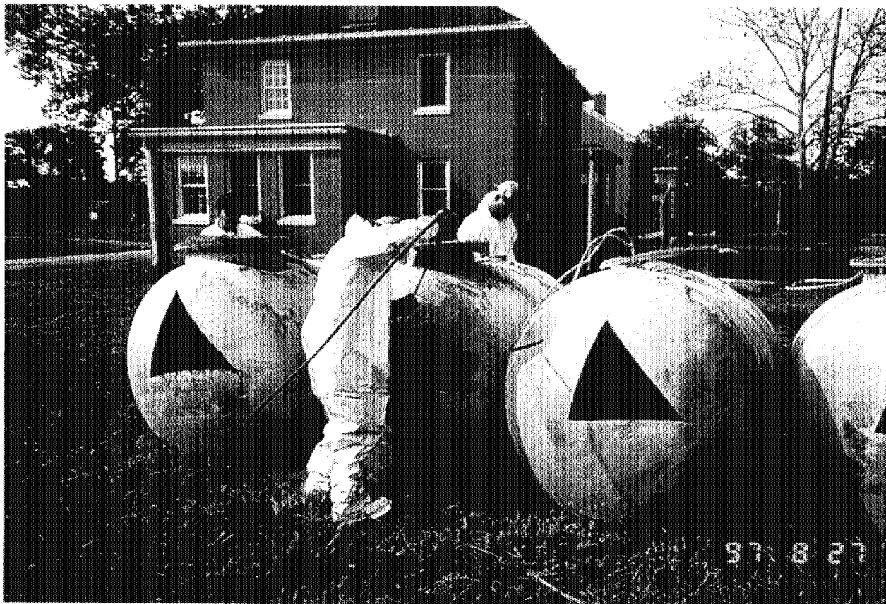
Photograph No.: 4 Contract No.: DACW31-95-D-0097 Location: Pedricktown U.S. Army Reserve Center (Bldg 276S) Photographer: B. Rayfield Description: Tanks cleaned using pressure washer.
