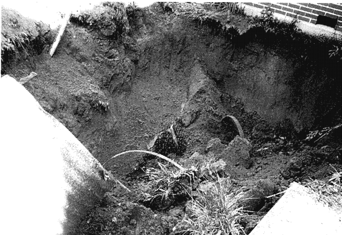
Photograph No.: 3 Contract No.: DACW31-95-D-0097 Location: Pedricktown U.S. Army Reserve Center (Bldg 276N) Photographer: B. Rayfield Description: Bottom of UST 276N excavation.
