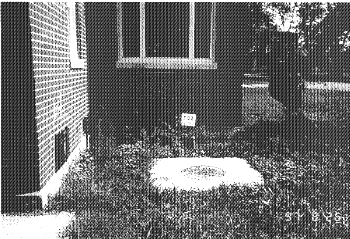
Photograph No.: 1 Contract No.: DACW31-95-D-0097 Location: Pedricktown U.S. Army Reserve Center (Bldg 278S) Photographer: B. Rayfield Description: Building 278S prior to excavation activities.
