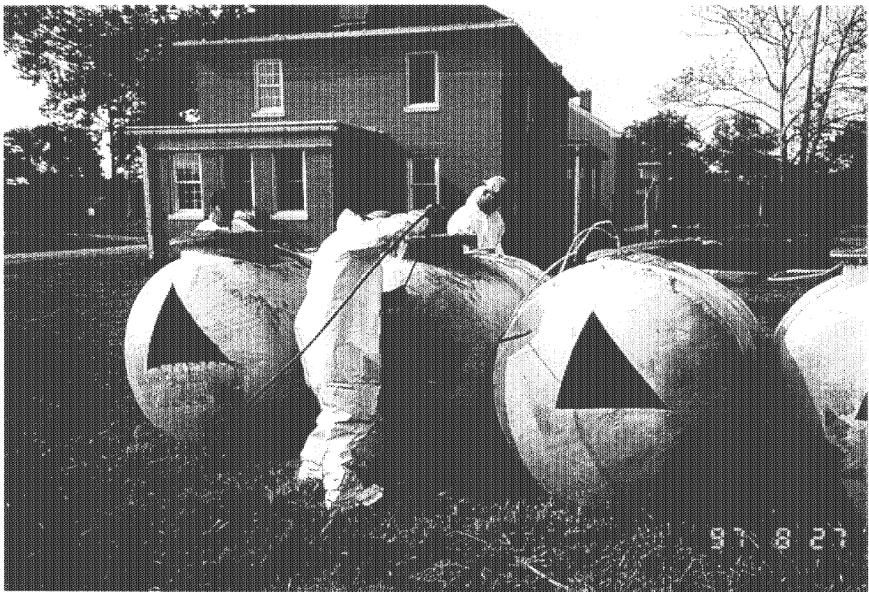
Photograph No.: 3 Contract No.: DACW31-95-D-0097 Location: Pedricktown U.S. Army Reserve Center (Bldg 278S) Photographer: B. Rayfield Description: Tanks cleaned using pressure washer.
