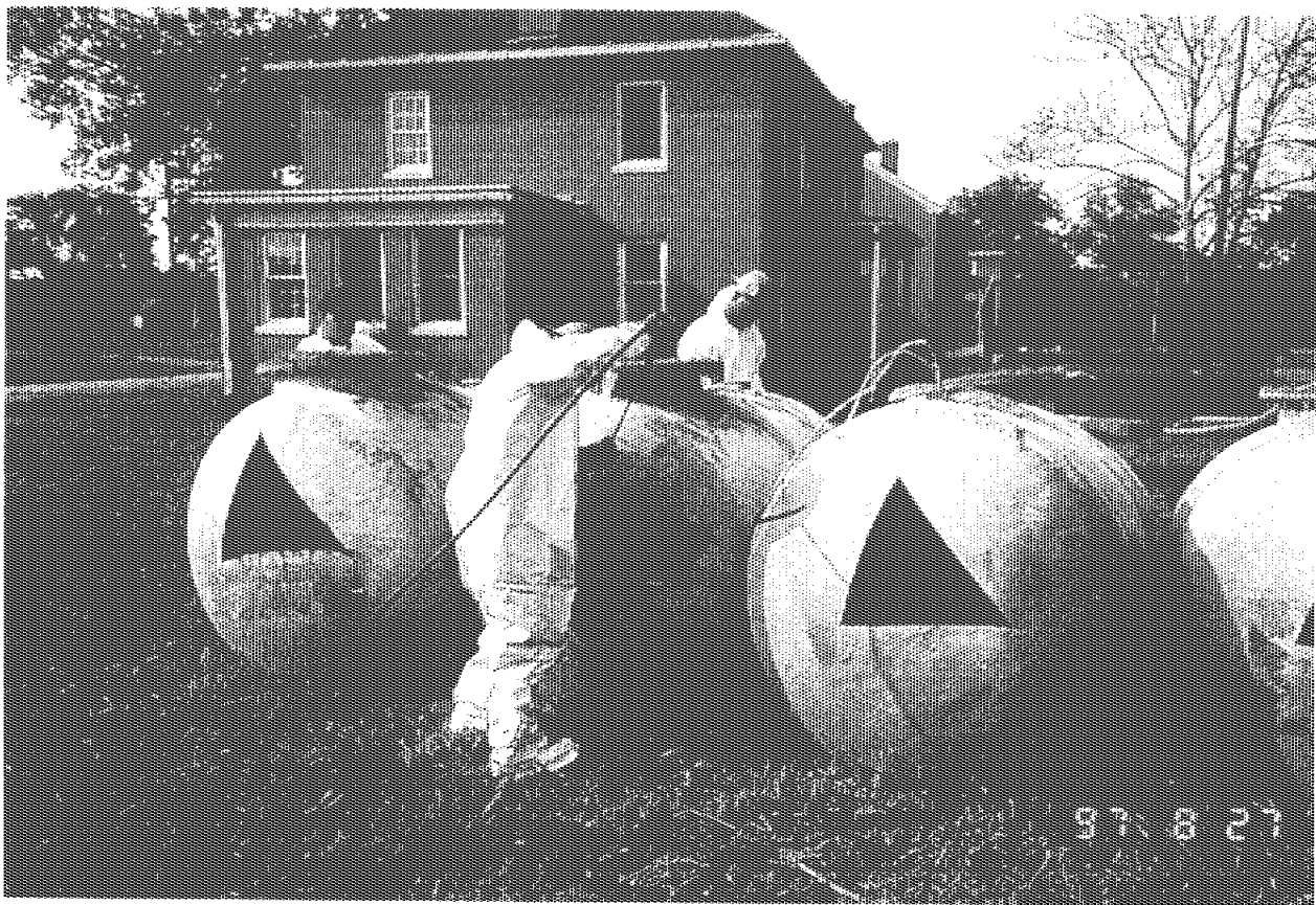
Photograph No.: 3 Contract No.: DACW31-95-D-0097 Location: Pedricktown U.S. Army Reserve Center (Bldg 2775) Photographer: B. Rayfield Description: Tanks cleaned using pressure washer.
