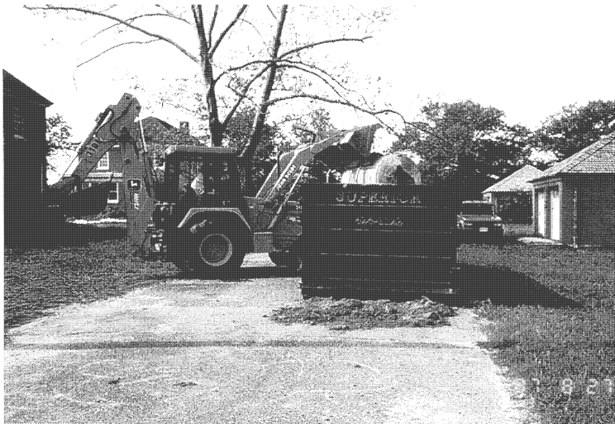
Photograph No.: 5 Contract No.: DACW31-95-D-0097 Location: Pedricktown U.S. Army Reserve Center (Bldg 278S) Photographer: B. Rayfield Description: Tank was loaded into rolloff box for disposal.
