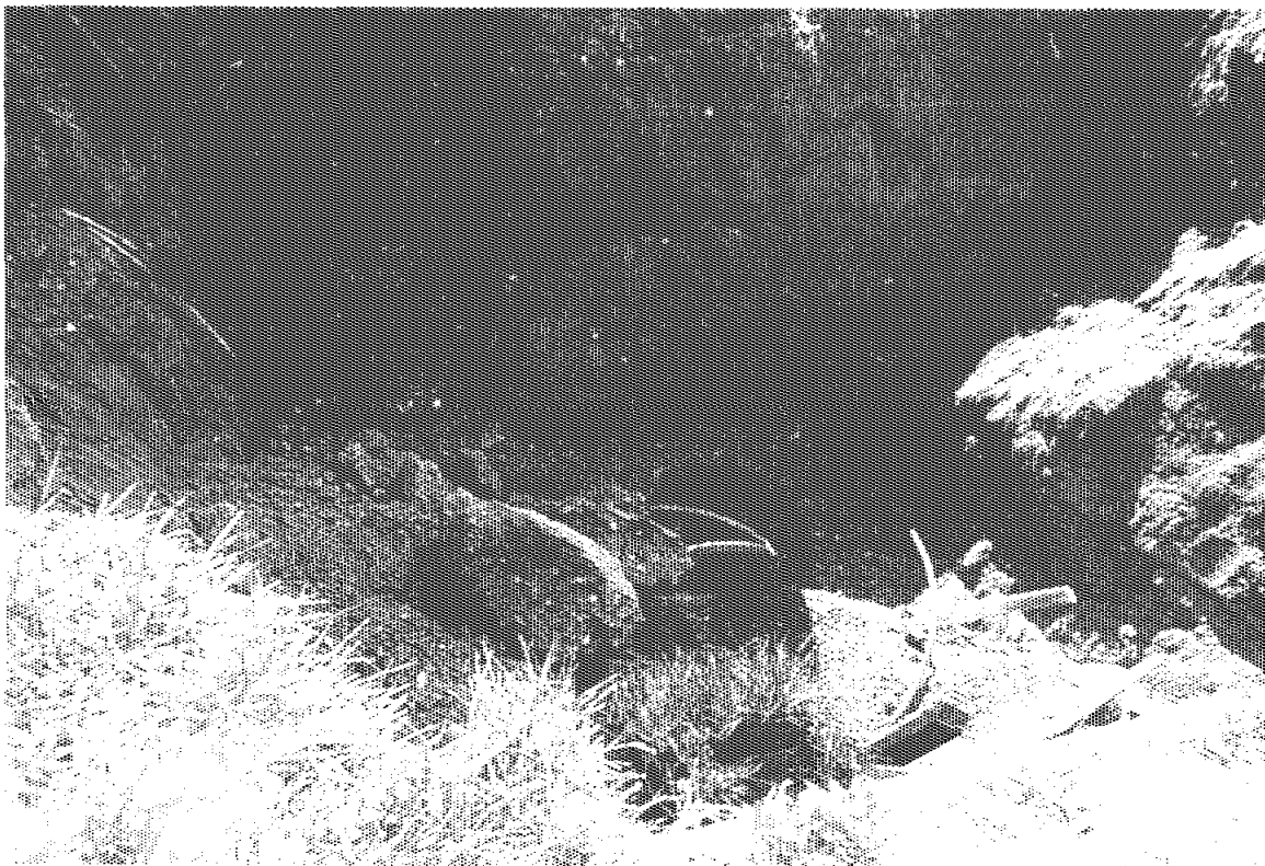
Photograph No.: 2 Contract No.: DACW31-95-D-0097 Location: Pedricktown U.S. Army Reserve Center (Bldg 277S) Photographer: B. Rayfield Description: Excavation after tank removal.
