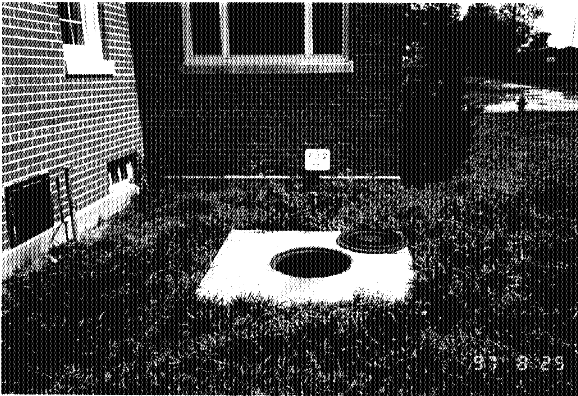
Photograph No.: 1 Contract No.: DACW31-95-D-0097 Location: Pedricktown U.S. Army Reserve Center (Bldg 276S) Photographer: B. Rayfield Description: Building 276S prior to excavation activities.
