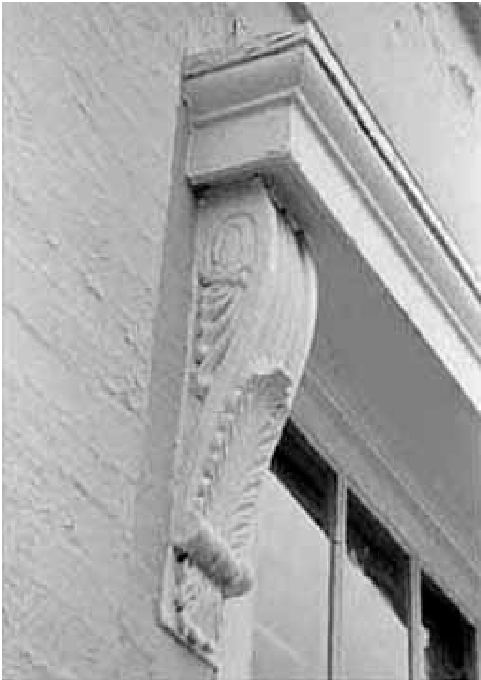
Figure 70 Old Naval Observatory (1844) Detail of bracketed window hood. This decorative detail was repeated in later additions.
