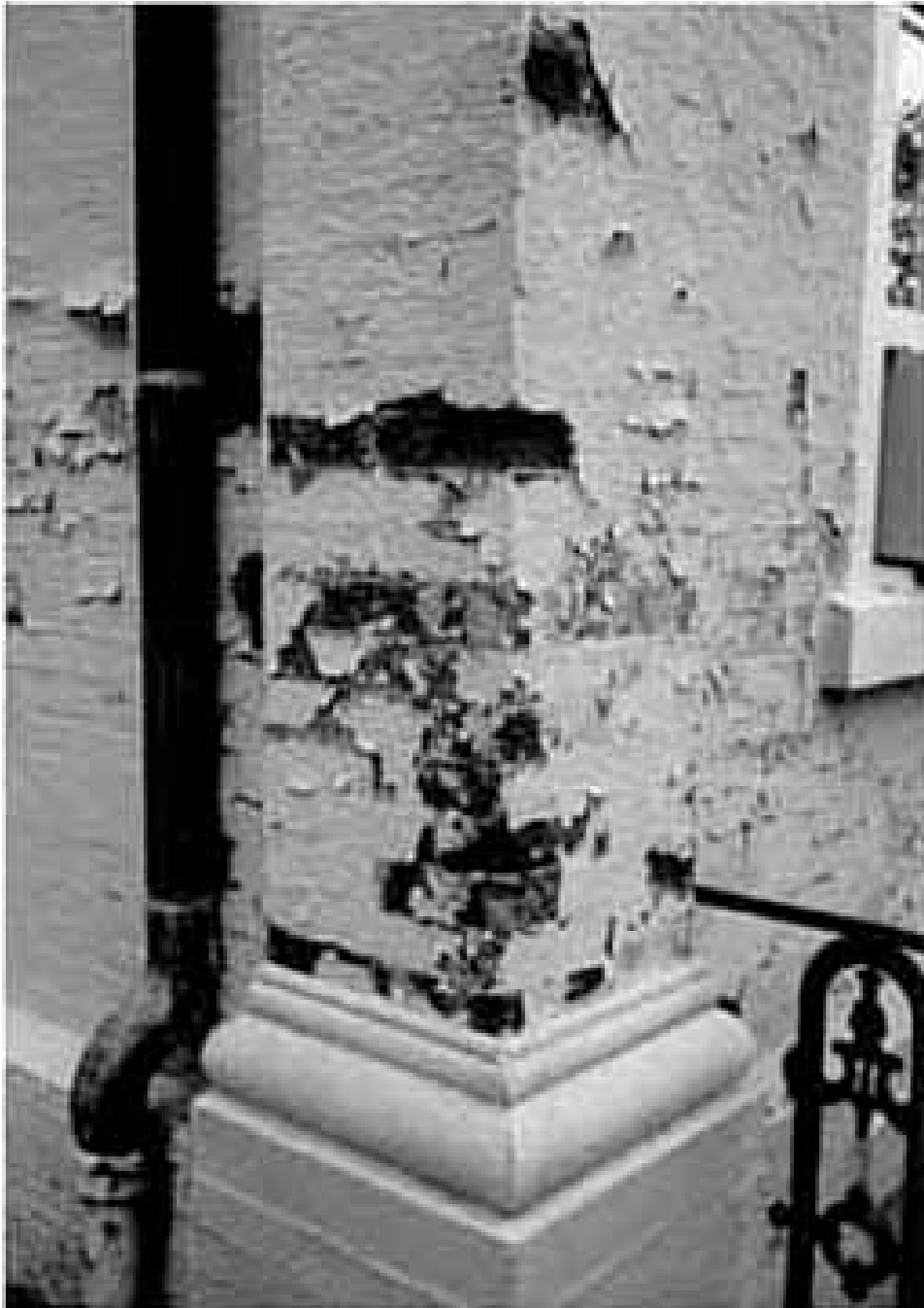
Figure 68 Old Naval Observatory (1844) Severe masonry deterioration on brick pier at northeast corner.
