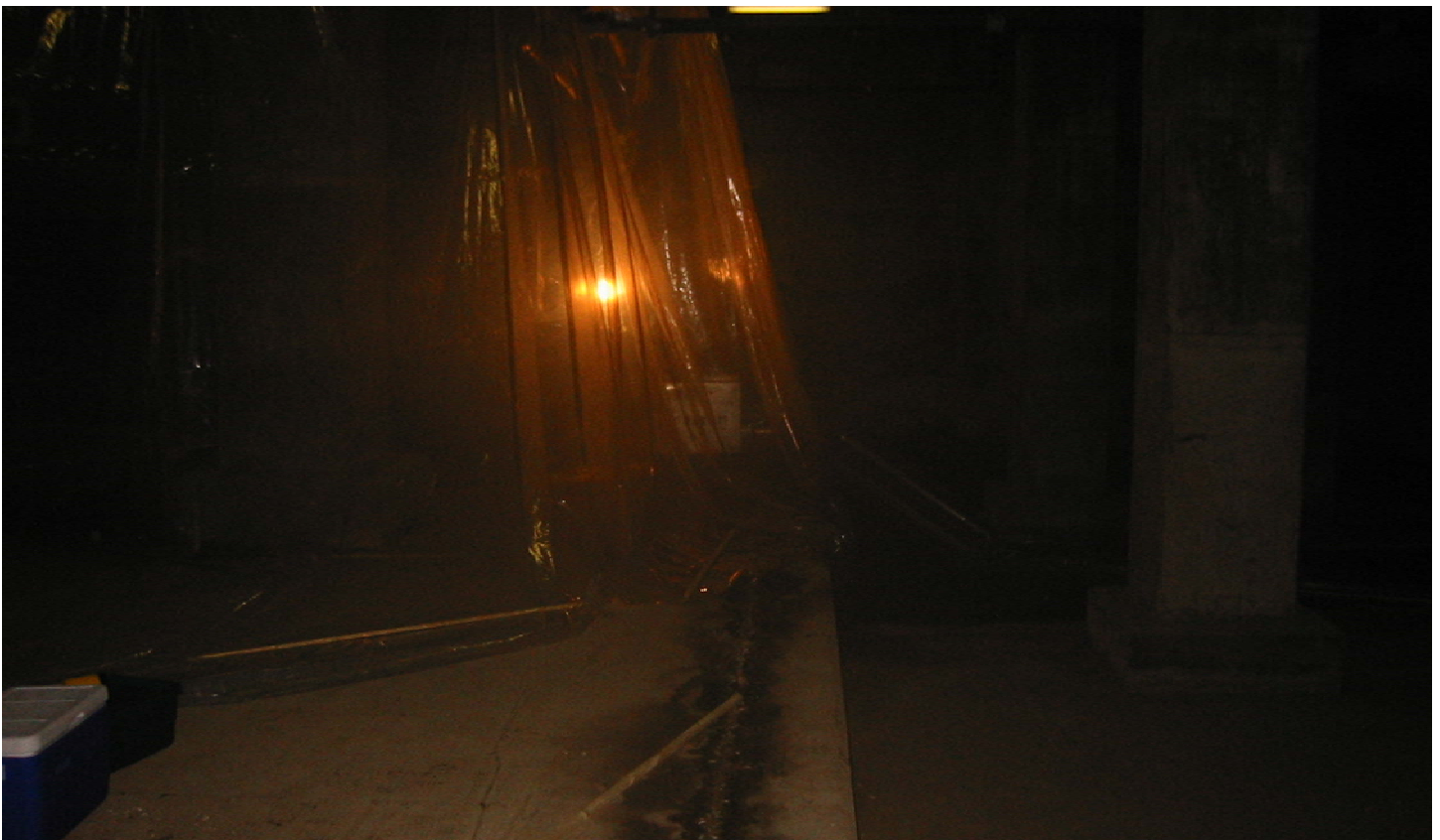
Photograph 8. Building 105 SAFR. Containment ledge drops off to floor with sump, September 2002.
