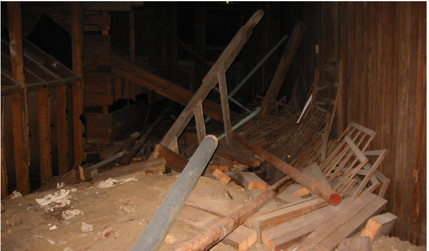
Photograph 3. Building 105A SAFR. Debris behind Bullet Pit, September 2002.
