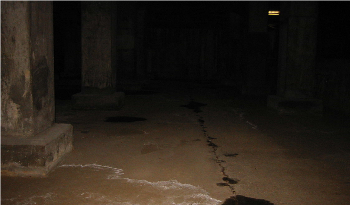
Photograph 5. Building 105 SAFR. Typical staining on floor, September 2002.
