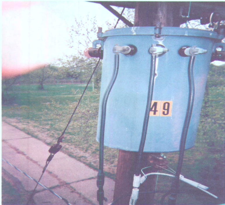
Transformer # 49, Building 286 Northwest
