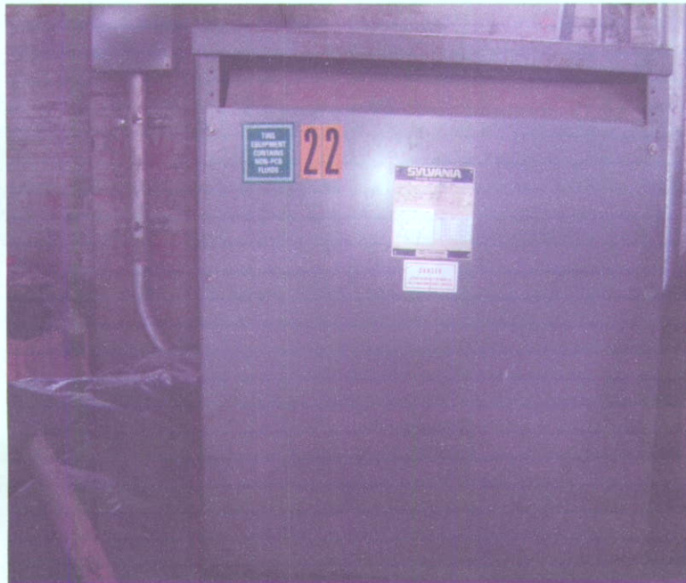
Transformer #22, Building 506 inside
