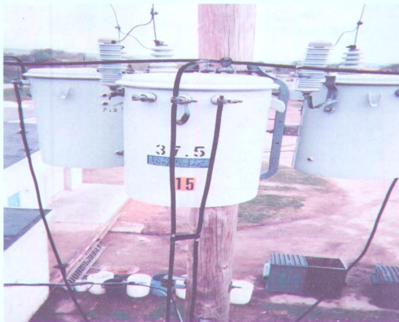
Transformer #15, Building 322 East
