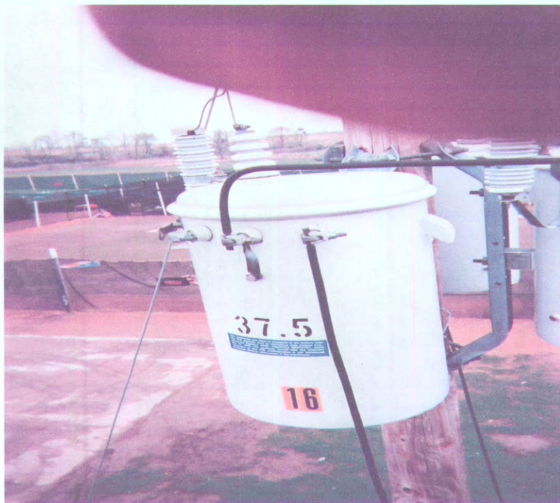
Transformer #16, Building 322 East
