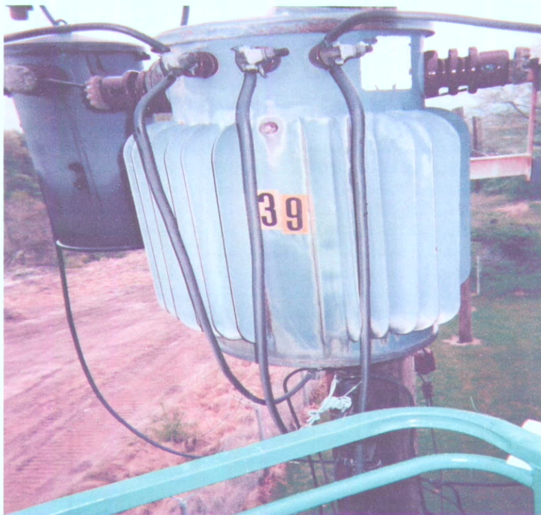
Transformer #39, Building 269 Southeast
