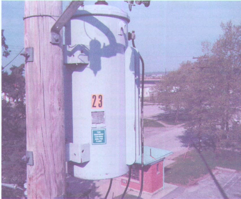
Transformer #23, Building 171 Southeast
