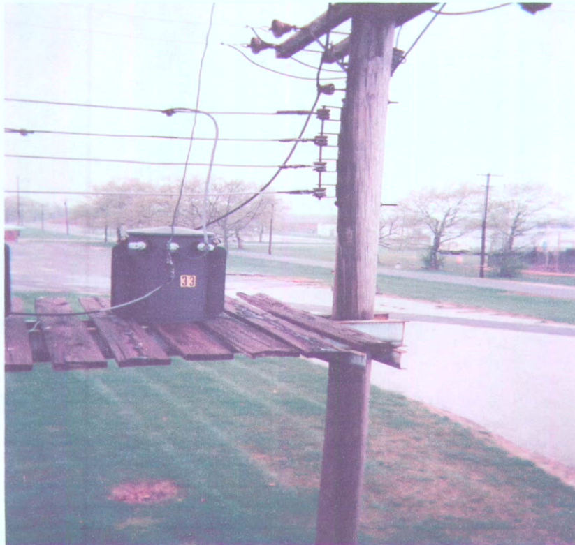
Transformer # 33, Building 173 North
