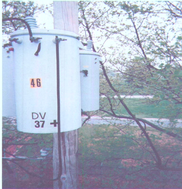
Transformer # 46, Building 285 West
