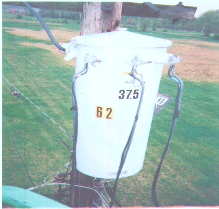
Transformer #62, Building 474 Southwest
