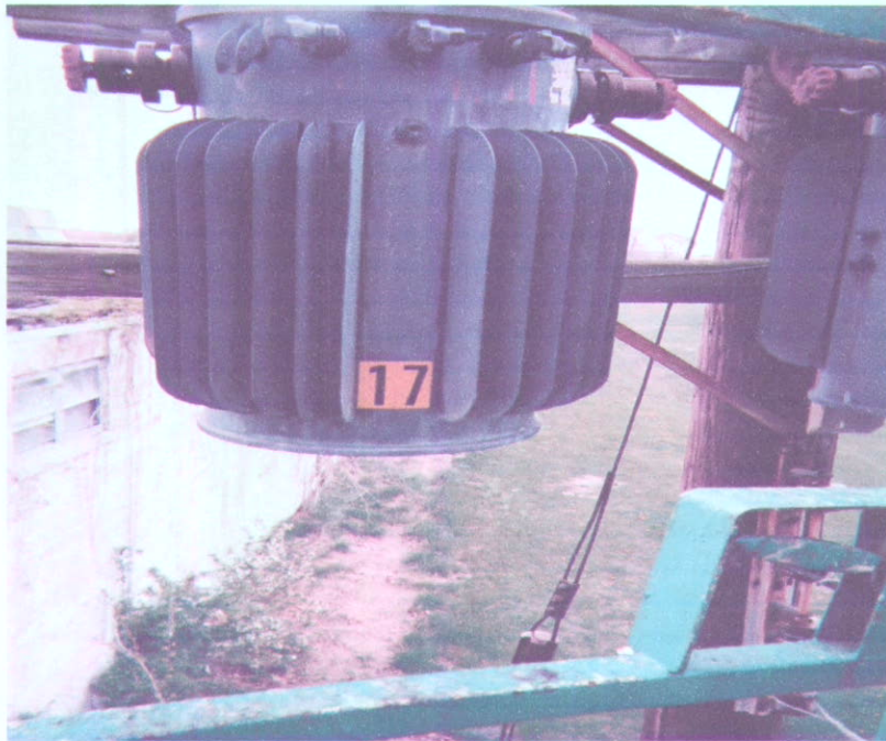
Transformer #17, Building 351 South
