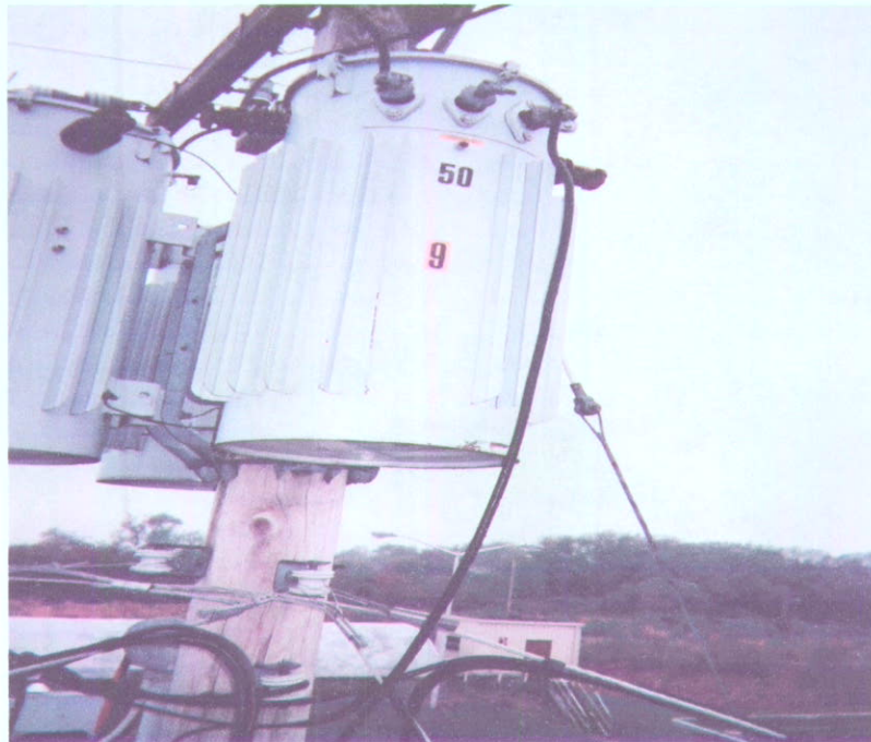
Transformer #9, Building 506 South
