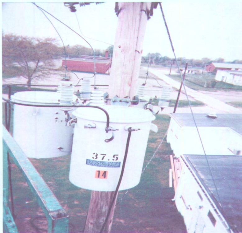
Transformer #14, Building 322 East
