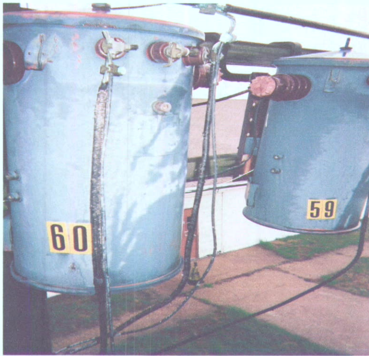
Transformer #60, Building 464 Southeast
