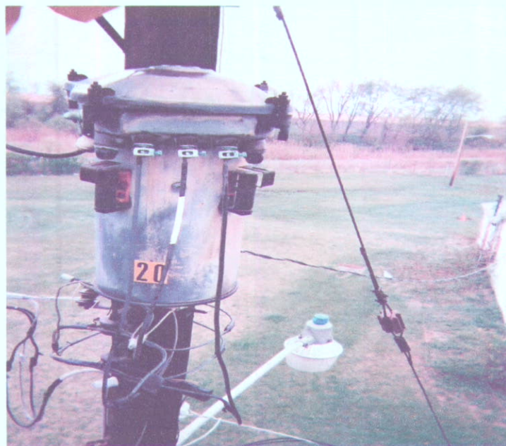
Transformer # 20, Building 380 Southwest
