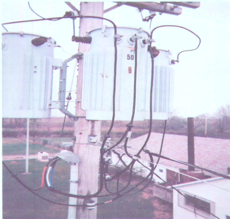
Transformer #8, Building 506 South
