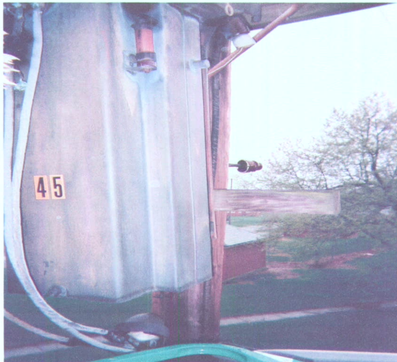
Transformer # 45, Building 273 West
