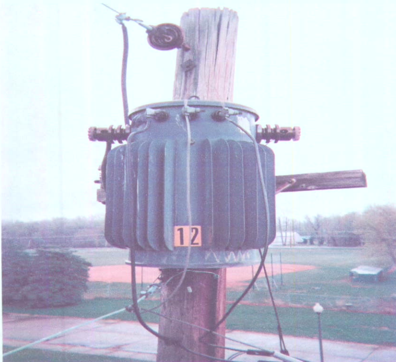
Transformer #12, Building 184 North
