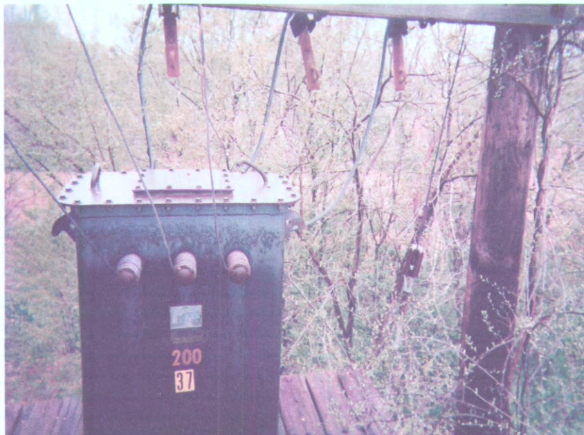
Transformer #37, Building 229 West
