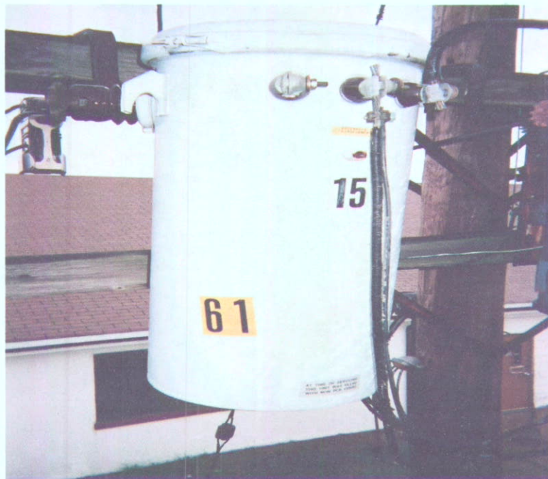
Transformer #61, Building 464 Southeast
