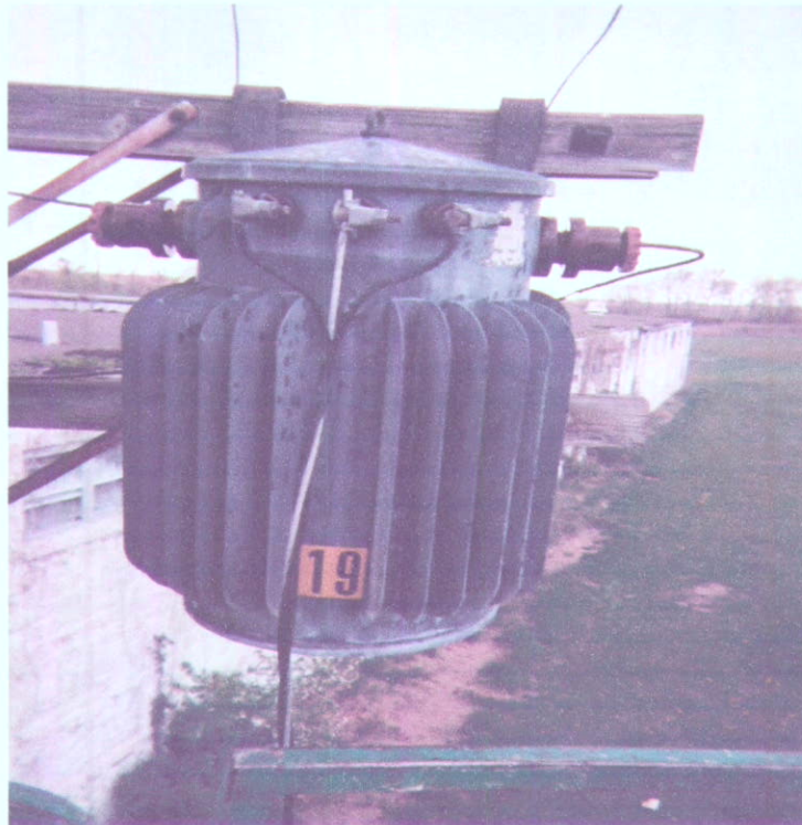
Transformer #19, Building 351 South
