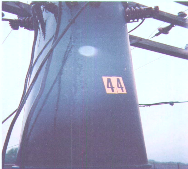
Transformer # 44, Building 273 North
