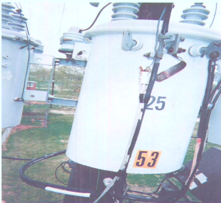
Transformer # 53, Building 404 Southeast
