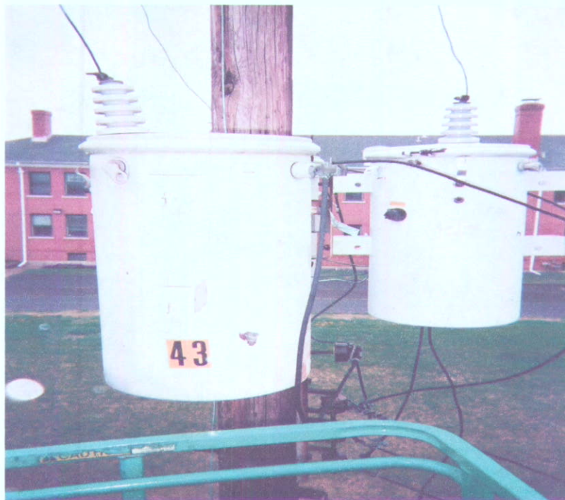
Transformer #43, Building 273 North
