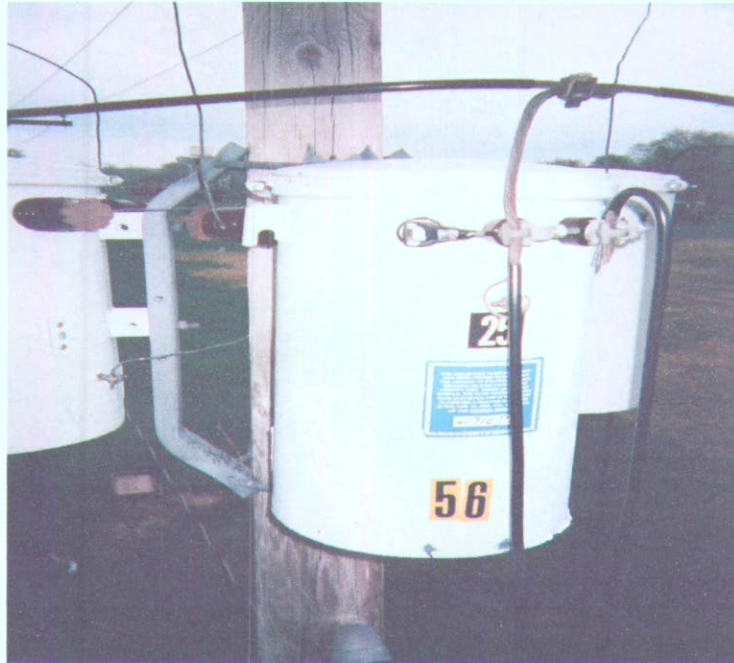
Transformer #56, Building 464 Southwest
