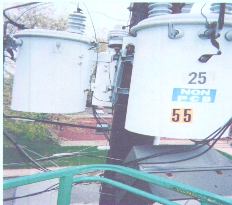
Transformer # 55, Building 404 South
