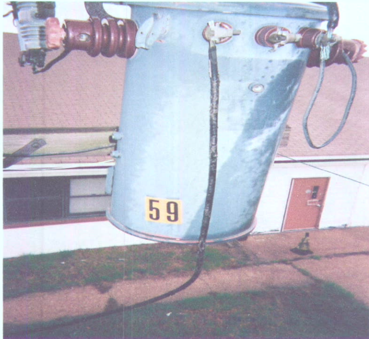
Transformer #59, Building 464 Southeast
