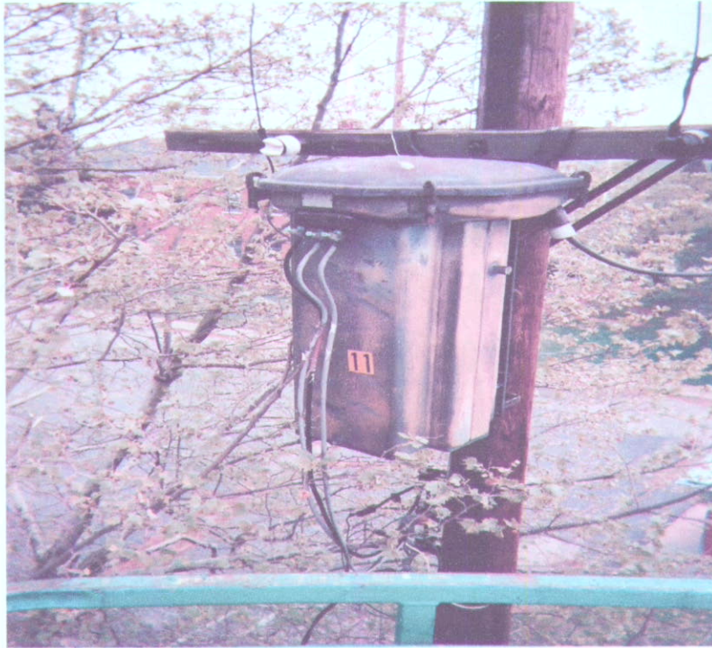
Transformer #11, Building 190 Northwest
