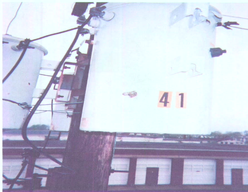
Transformer #41, Building 273 North
