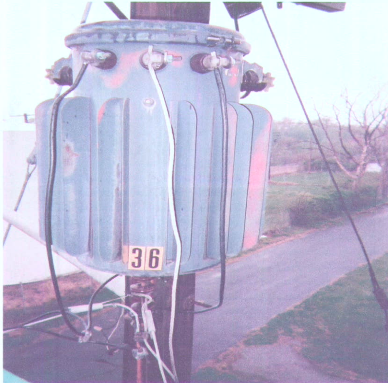
Transformer #36, Building 229 North
