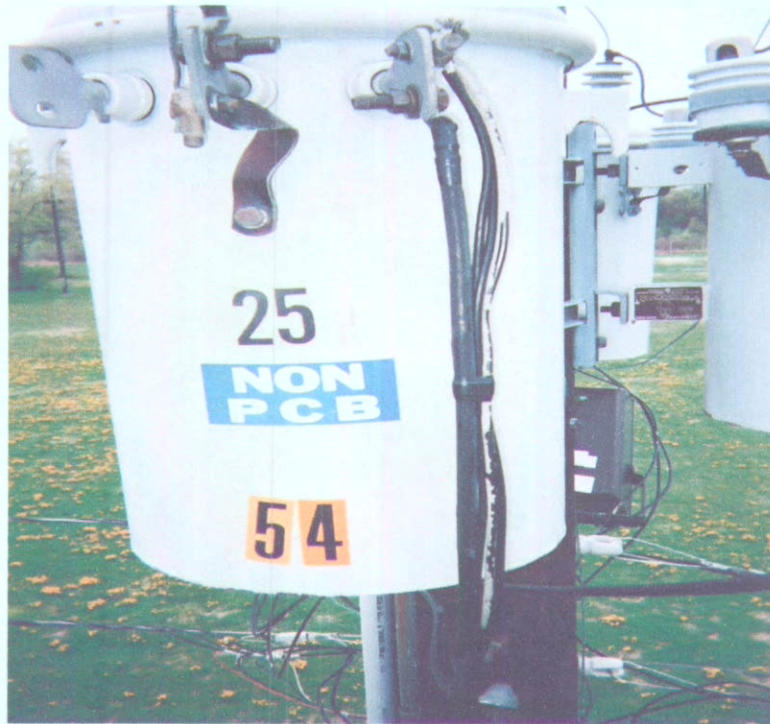
Transformer # 54, Building 404 South
