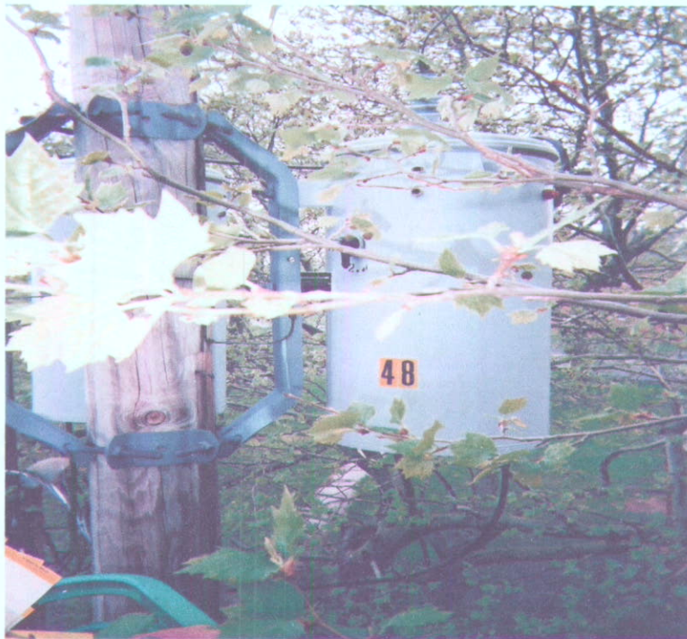
Transformer # 48, Building 285 West
