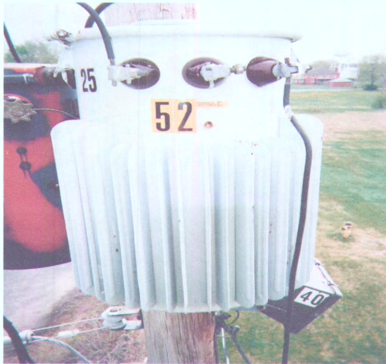
Transformer #52, Building 434 Southeast
