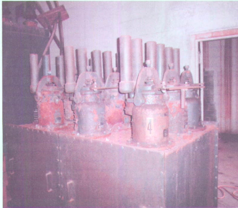
Switch Box #4, Building 422
