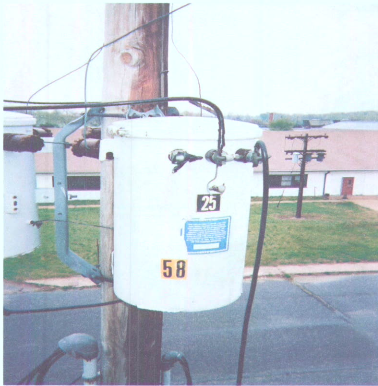
Transformer #58, Building 273 Southwest
