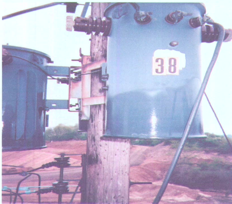
Transformer #38, Building 269 Southeast
