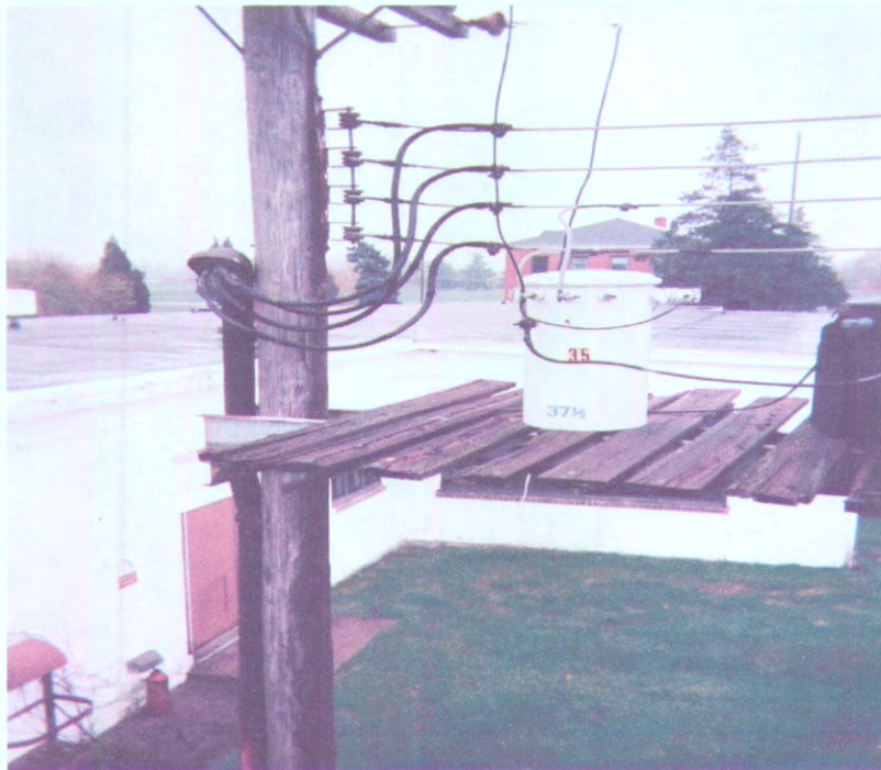
Transformer # 35, Building 173 North
