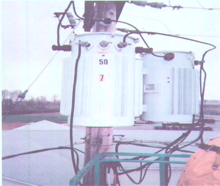
Transformer #7, Building 506 South
