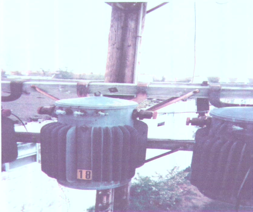
Transformer #18, Building 351 South
