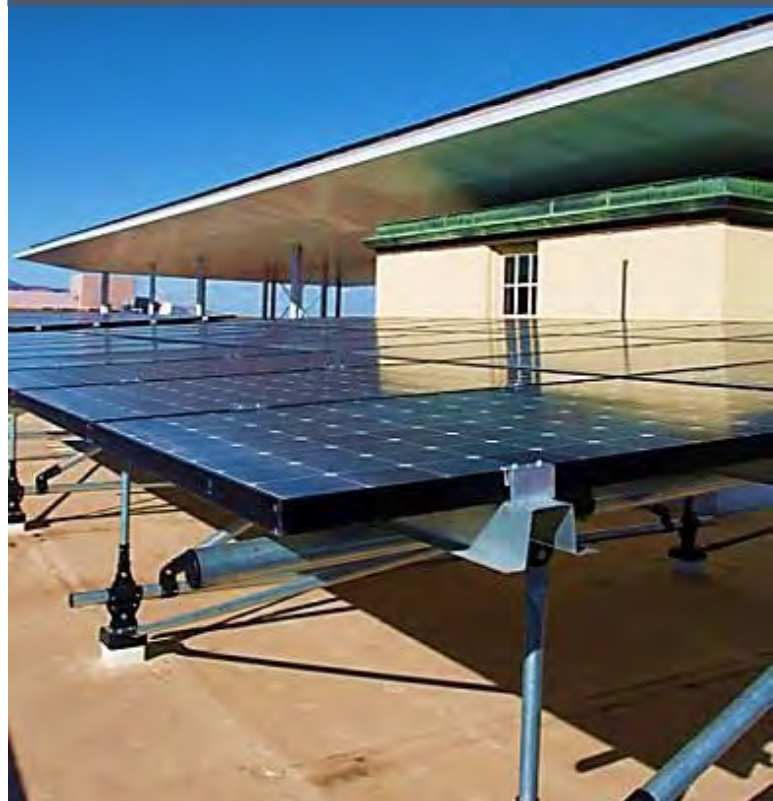
Figure 17: Wayne Aspinall Federal Building and U.S. Courthouse Solar System, Grand Junction, CO
