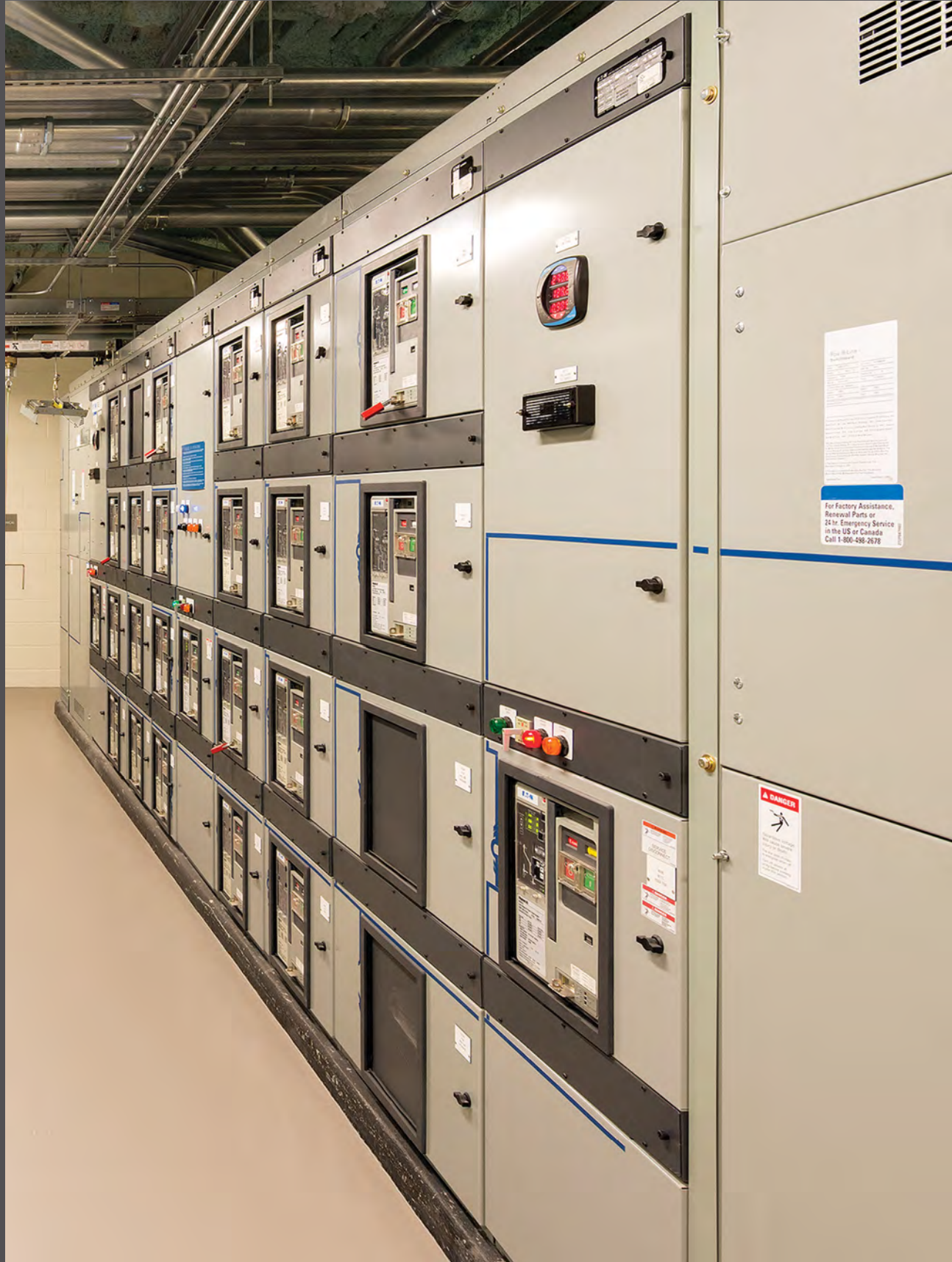
Figure 12: Bishop Henry Whipple Federal Building Electrical Switchgear Fort Snelling, MN
