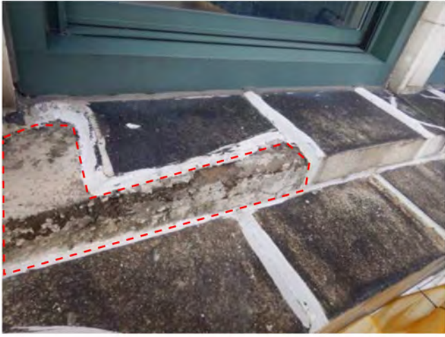
Photo 57: R/S cracks, failed sealant, remove loose + seal
