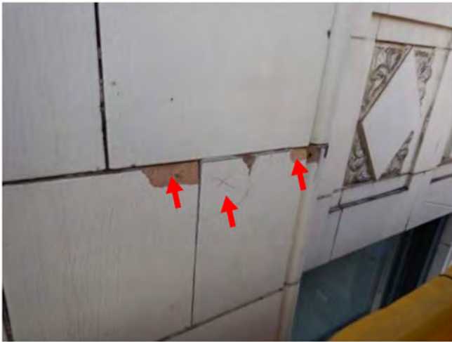
Photo 41: Remove loose + seal
