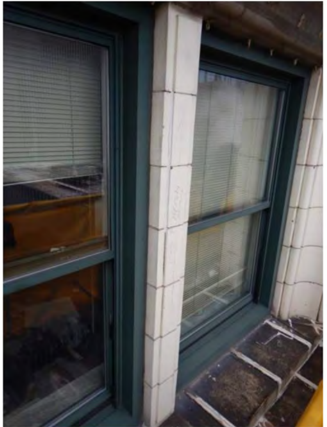
Photo 8: R/S cracks + mesh
