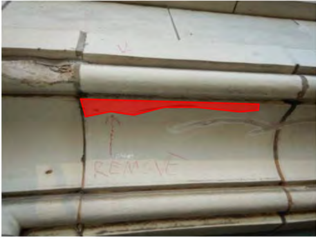
Photo 5: Remove loose & seal
