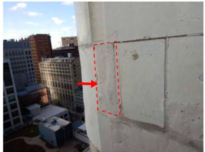
Photo 68: Remove loose + seal
