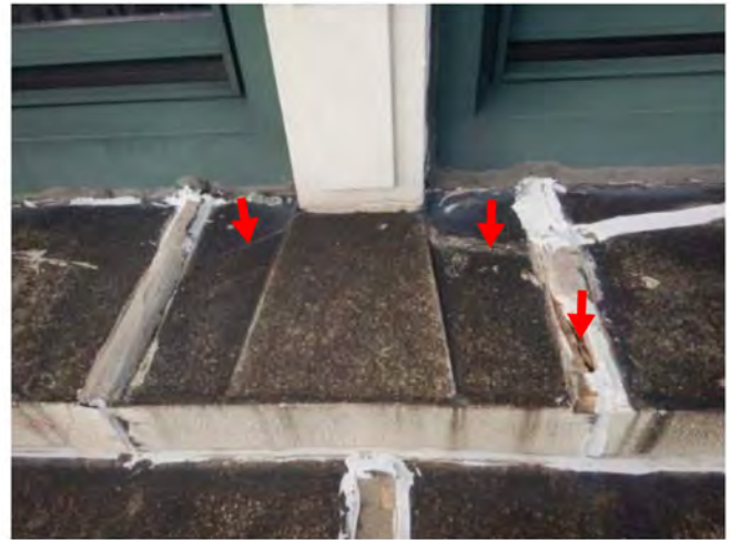
Photo 20: R/S cracks, failed sealant, remove loose + seal
