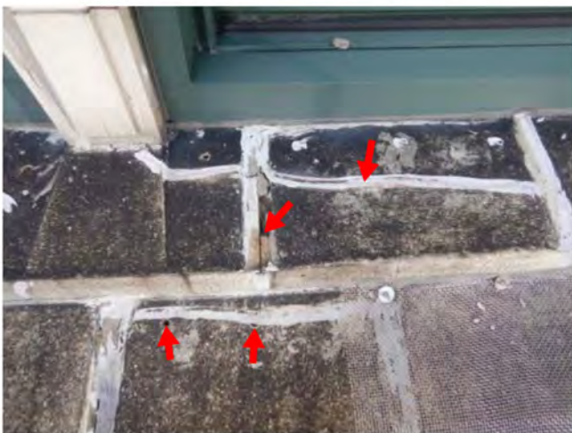
Photo 55: R/S cracks, failed sealant, remove loose + seal
