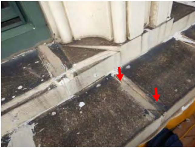
Photo 17: R/S cracks, failed sealant, remove loose + seal
