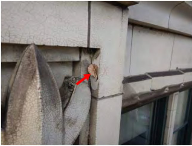
Photo 11: Remove loose + seal
