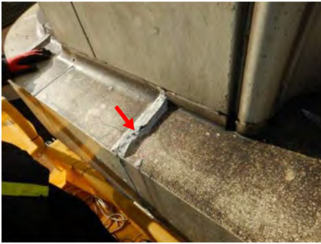
Photo 171: R/S cracks, failed sealant, remove loose + seal
