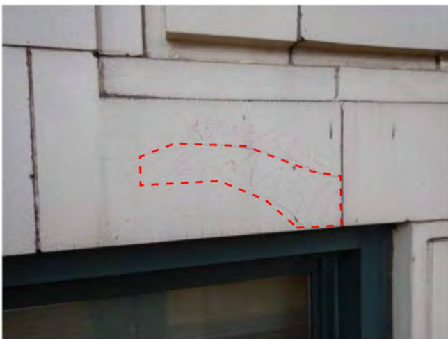
Photo 43: Remove loose + seal
