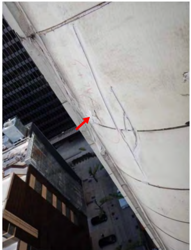
Photo 102: Remove loose + seal
