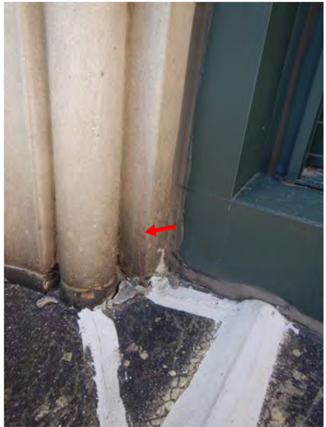
Photo 180: R/S cracks, failed sealant, remove loose + seal
