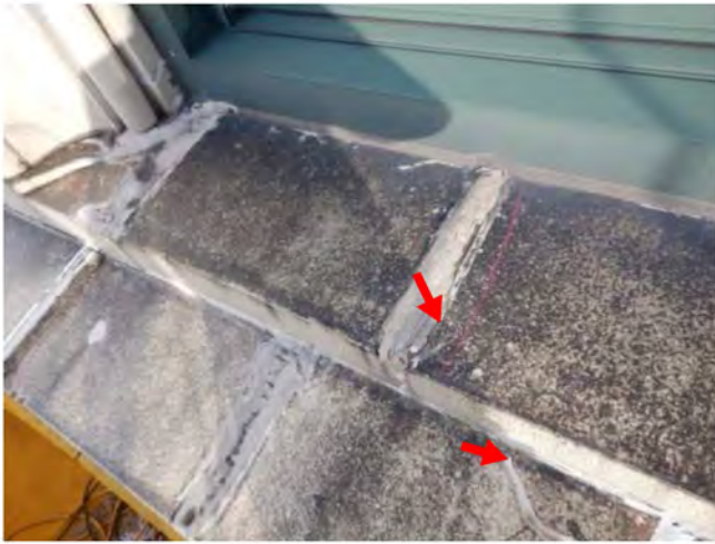
Photo 47: R/S cracks, failed sealant, remove loose + seal
