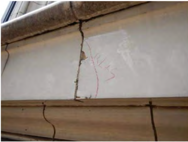
Photo 47: Remove loose & seal
