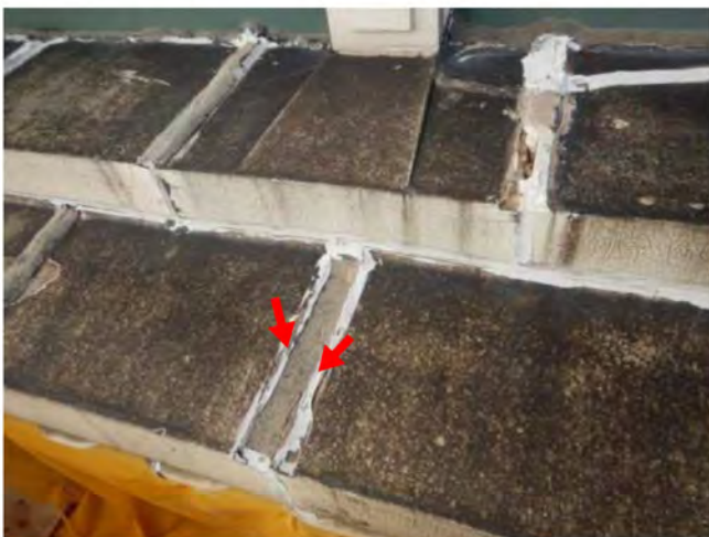
Photo 21: R/S cracks, failed sealant, remove loose + seal
