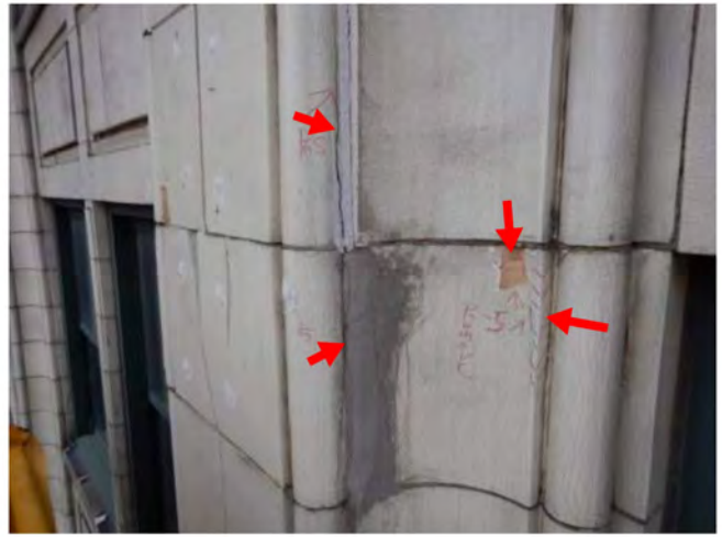
Photo 92: Remove loose + seal
