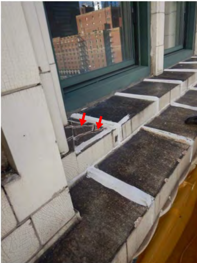
Photo 25: R/S cracks, failed sealant, remove loose + seal
