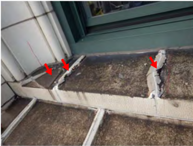
Photo 13: R/S cracks, failed sealant, remove loose + seal
