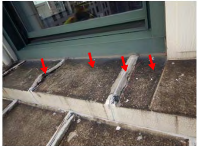
Photo 14: R/S cracks, failed sealant, remove loose + seal
