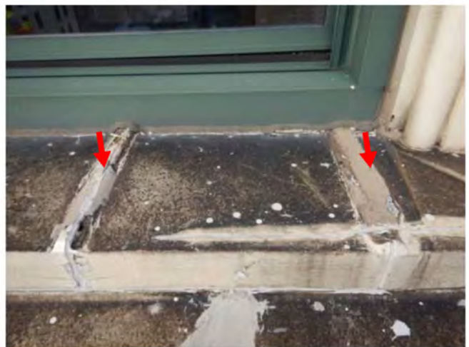
Photo 16: R/S cracks, failed sealant, remove loose + seal
