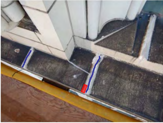
Photo 9: Remove loose & R/S
