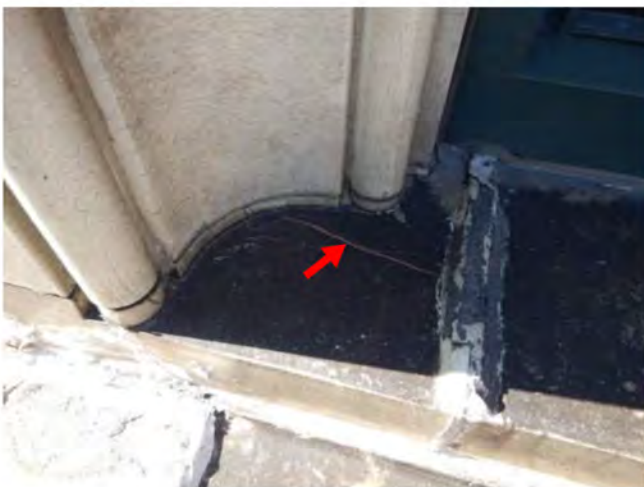
Photo 189: R/S cracks, failed sealant, remove loose + seal
