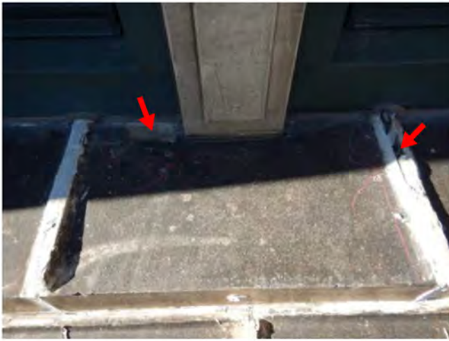
Photo 191: R/S cracks, failed sealant, remove loose + seal
