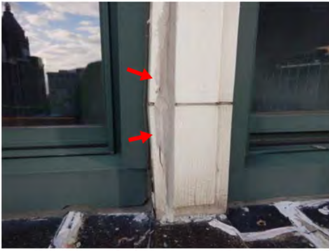
Photo 45: Remove loose + seal
