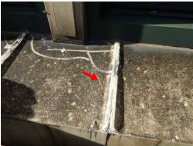
Photo 175: R/S cracks, failed sealant, remove loose + seal
