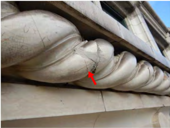
Photo 29: Remove loose + seal
