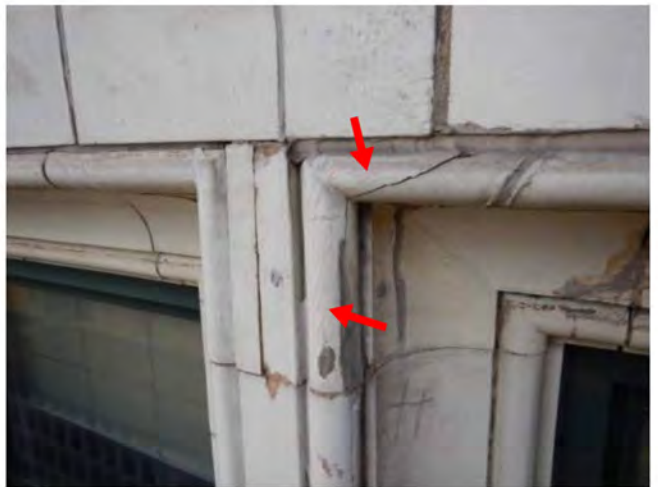
Photo 62: Remove loose + seal
