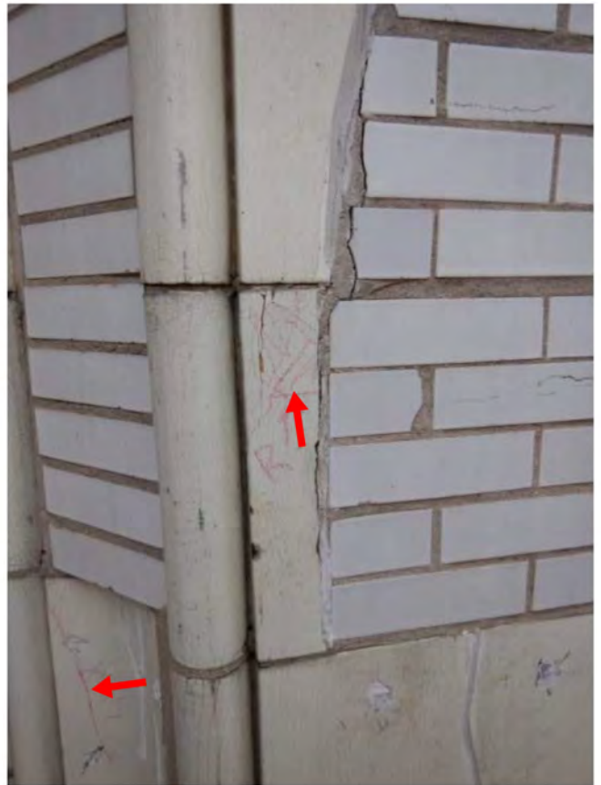
Photo 104: Remove loose + seal
