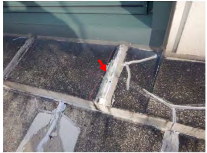
Photo 48: R/S cracks, failed sealant, remove loose + seal
