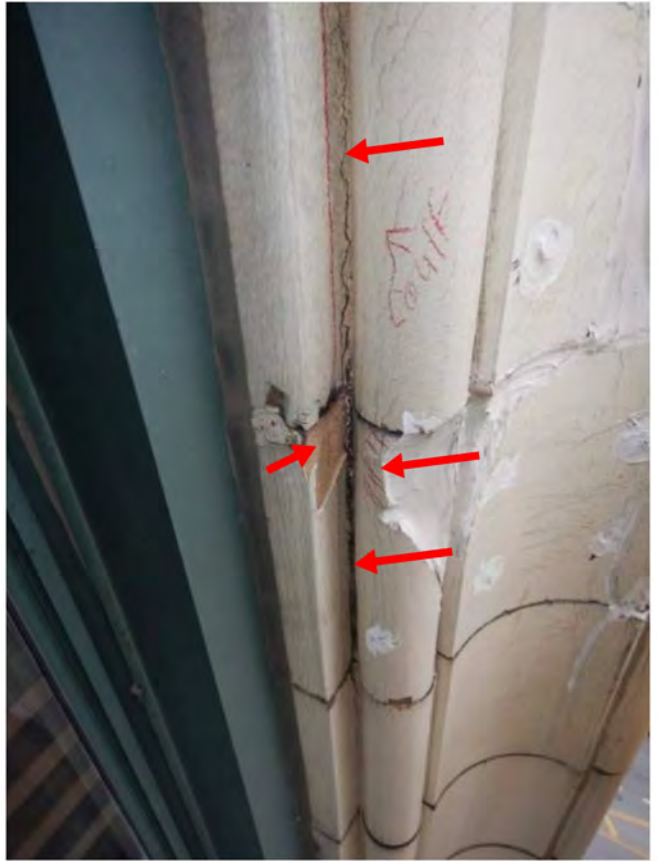
Photo 84: Remove loose + seal
