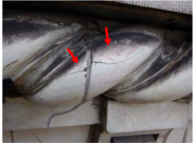
Photo 22: Remove loose + seal
