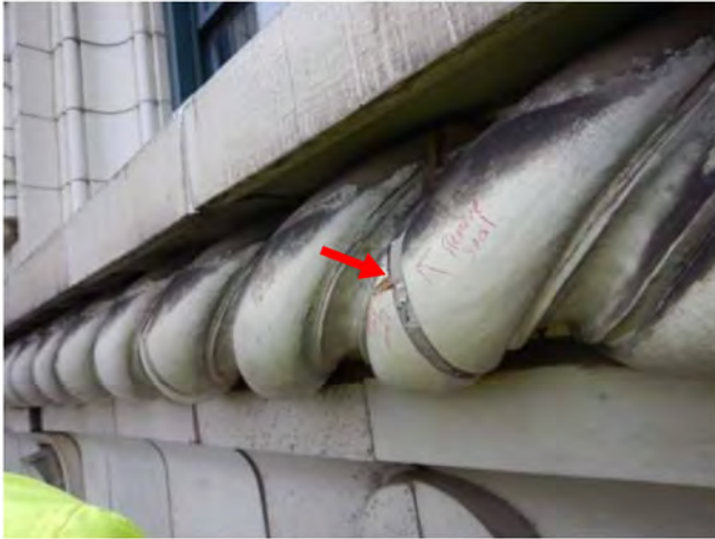
Photo 21: Remove loose + seal
