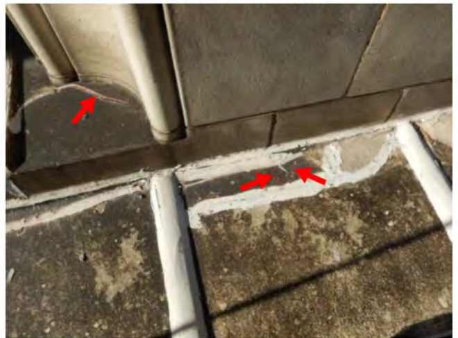
Photo 196: R/S cracks, failed sealant, remove loose + seal
