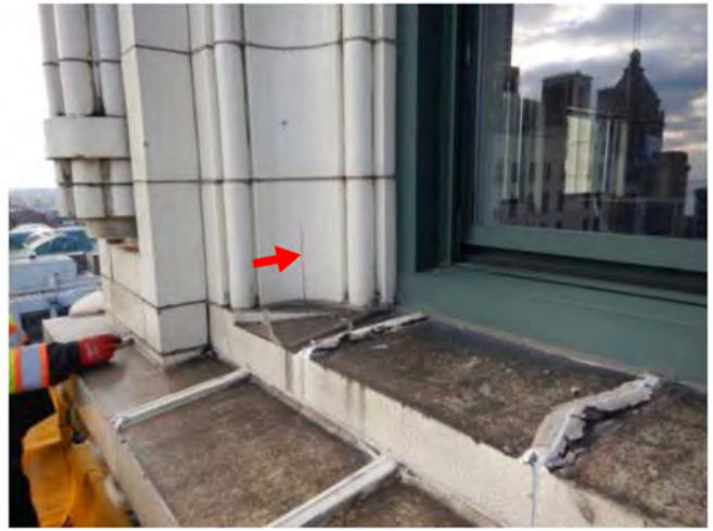
Photo 12: R/S cracks, failed sealant, remove loose + seal
