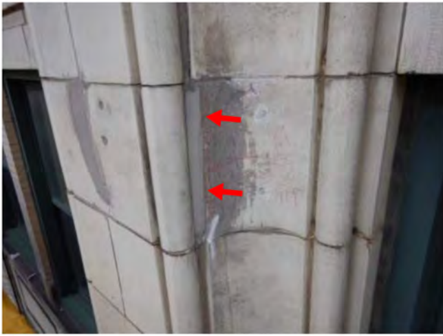
Photo 115: Remove loose + seal
