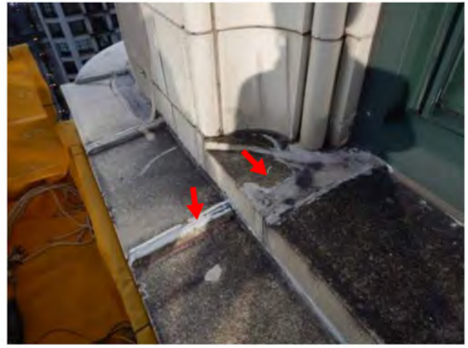
Photo 46: R/S cracks, failed sealant, remove loose + seal
