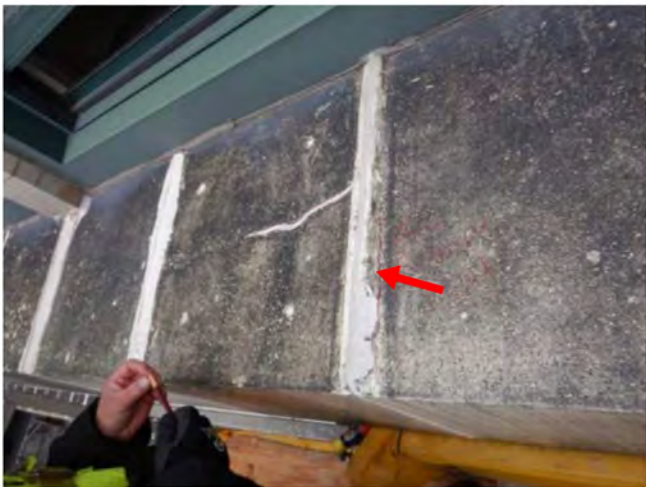
Photo 139: Remove loose + seal
