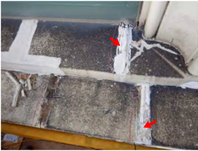
Photo 51: R/S cracks, failed sealant, remove loose + seal
