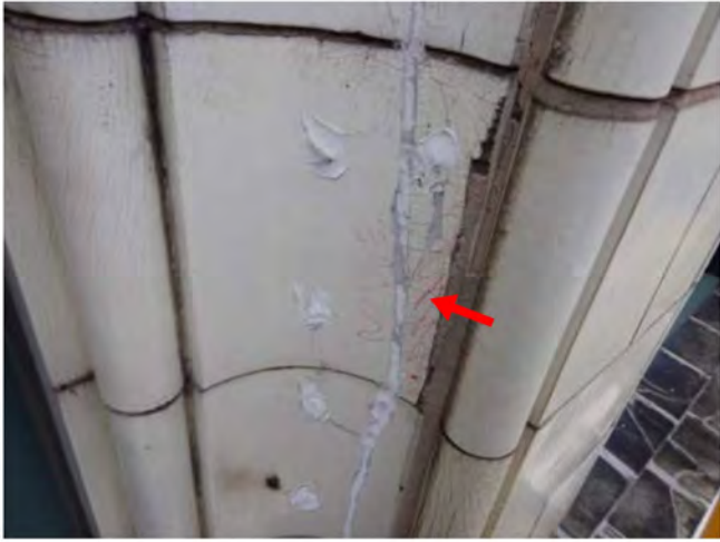
Photo 33: Remove loose + seal
