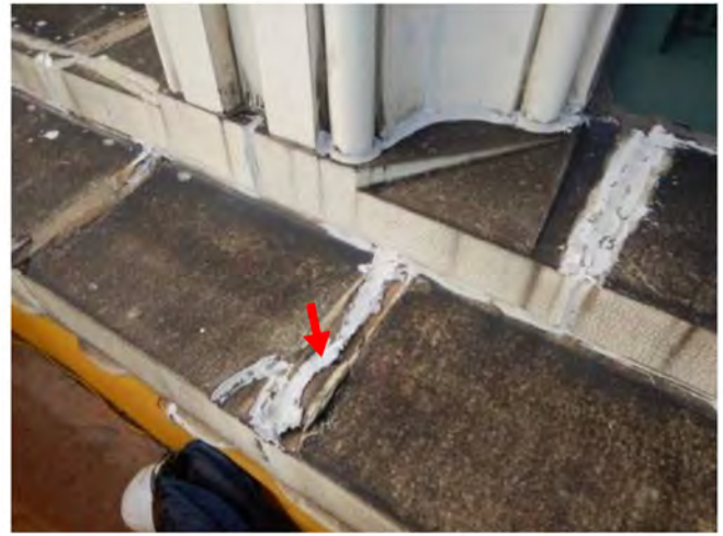
Photo 18: R/S cracks, failed sealant, remove loose + seal
