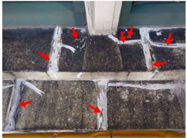
Photo 54: R/S cracks, failed sealant, remove loose + seal
