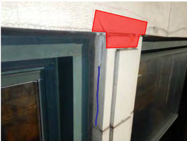
Photo 49: Remove loose & seal + R/S
