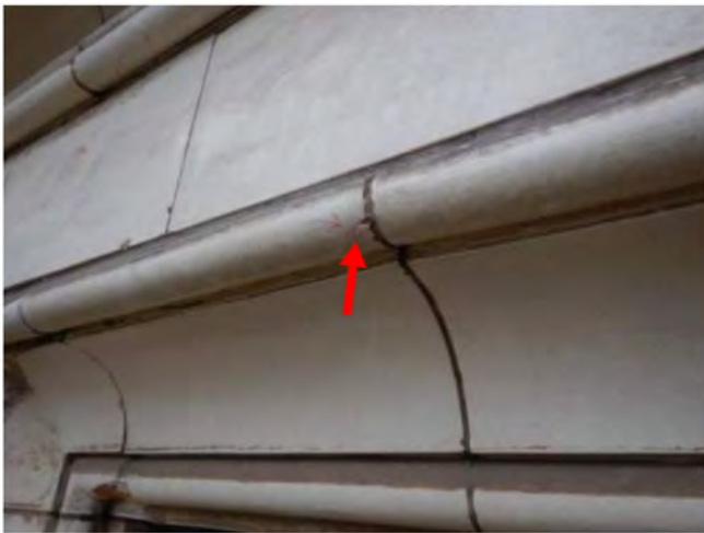
Photo 59: Remove loose + seal
