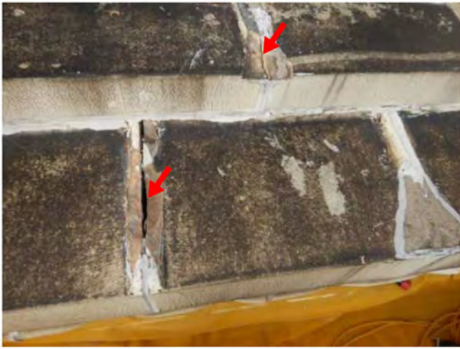
Photo 23: R/S cracks, failed sealant, remove loose + seal
