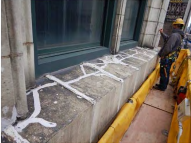
Photo 39: R/S cracks, failed sealant, remove loose material & seal
