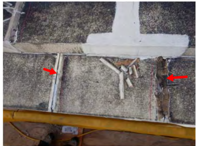
Photo 50: R/S cracks, failed sealant, remove loose + seal
