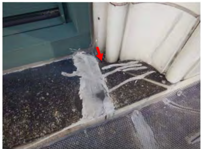
Photo 56: R/S cracks, failed sealant, remove loose + seal
