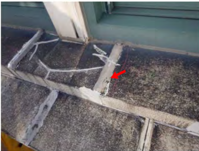
Photo 49: R/S cracks, failed sealant, remove loose + seal
