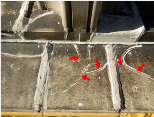
Photo 193: R/S cracks, failed sealant, remove loose + seal
