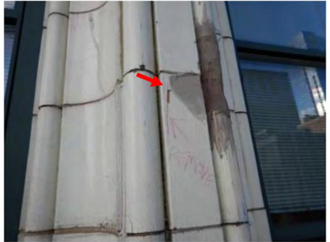
Photo 80: Remove loose + seal
