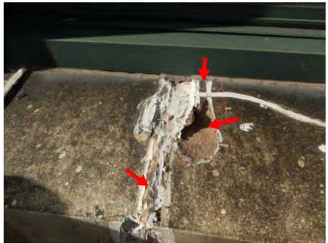
Photo 176: R/S cracks, failed sealant, remove loose + seal
