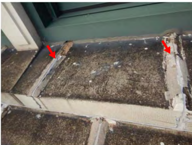
Photo 15: R/S cracks, failed sealant, remove loose + seal
