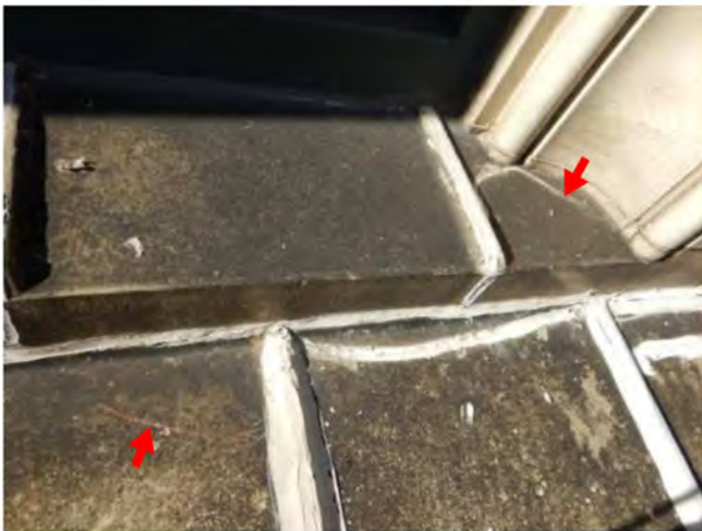
Photo 195: R/S cracks, failed sealant, remove loose + seal
