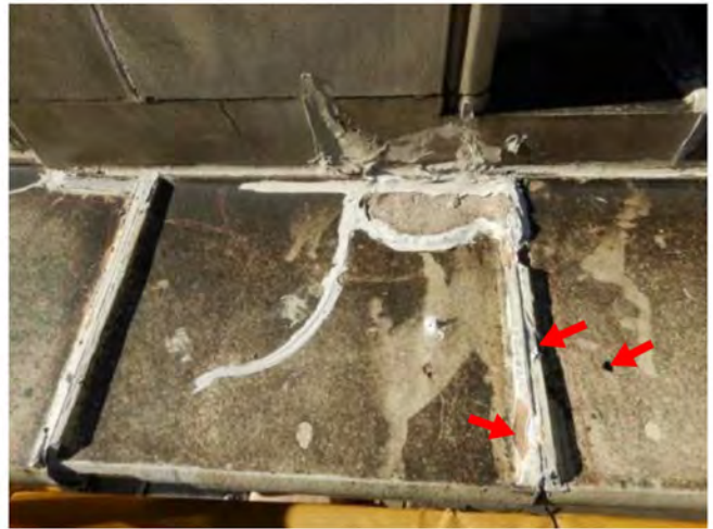
Photo 188: R/S cracks, failed sealant, remove loose + seal
