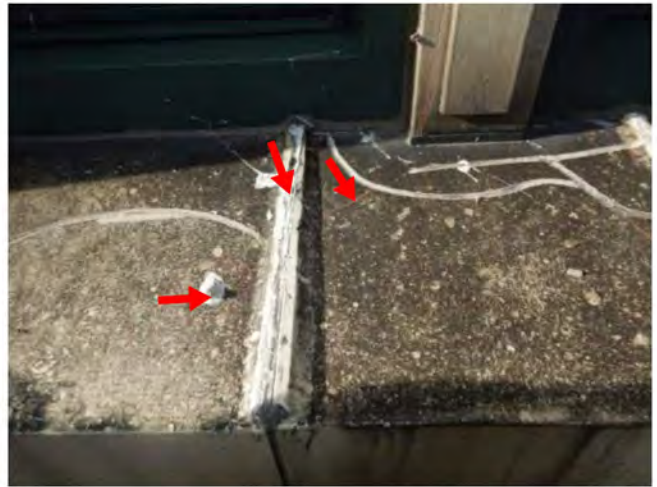
Photo 174: R/S cracks, failed sealant, remove loose + seal
