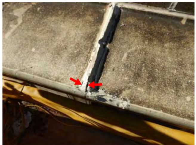
Photo 190: R/S cracks, failed sealant, remove loose + seal
