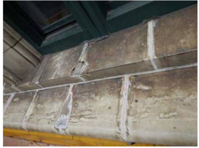
Photo 46: R/S cracks, failed sealant, remove loose material & seal
