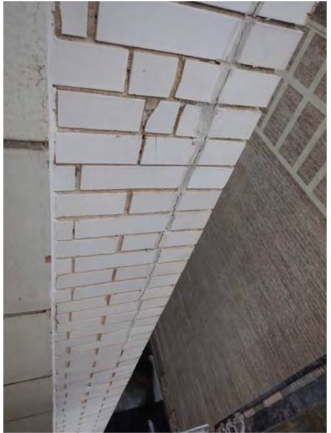
Photo 12: Seal cracked brick & mesh
