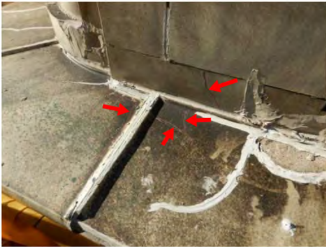
Photo 187: R/S cracks, failed sealant, remove loose + seal
