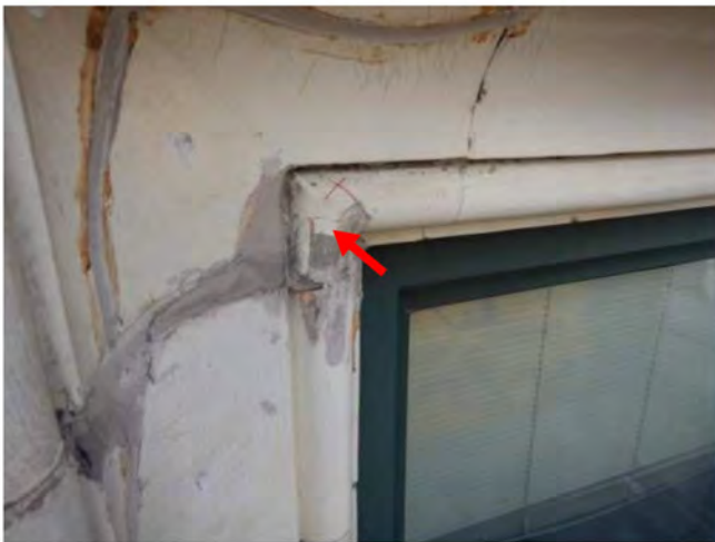
Photo 67: Remove loose + seal
