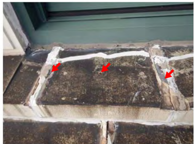
Photo 22: R/S cracks, failed sealant, remove loose + seal
