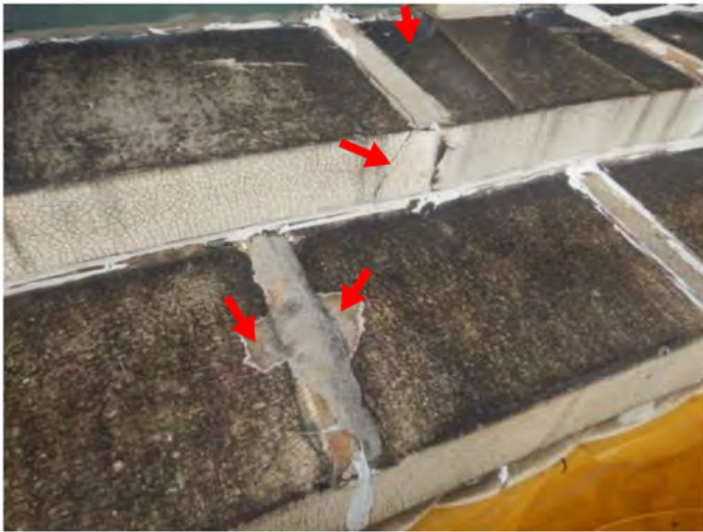
Photo 19: R/S cracks, failed sealant, remove loose + seal
