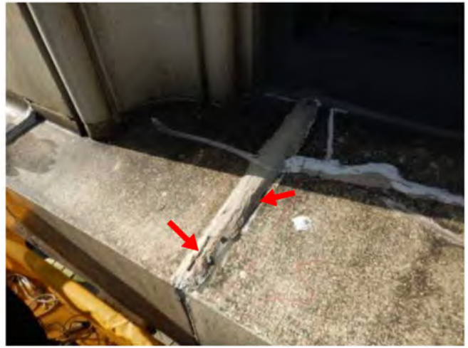
Photo 172: R/S cracks, failed sealant, remove loose + seal
