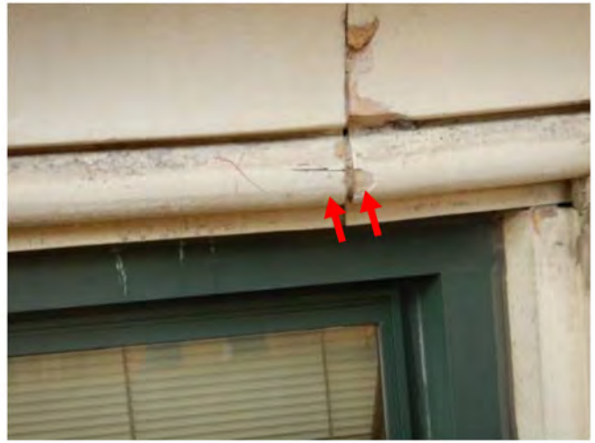
Photo 28: Remove loose + seal
