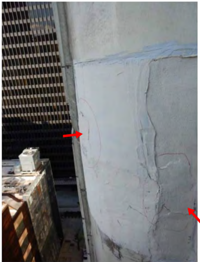
Photo 88: Remove loose + seal
