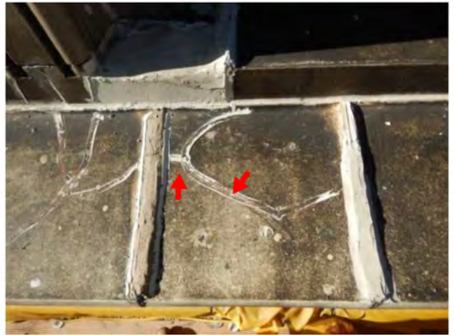
Photo 194: R/S cracks, failed sealant, remove loose + seal
