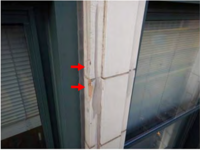
Photo 74: Remove loose + seal
