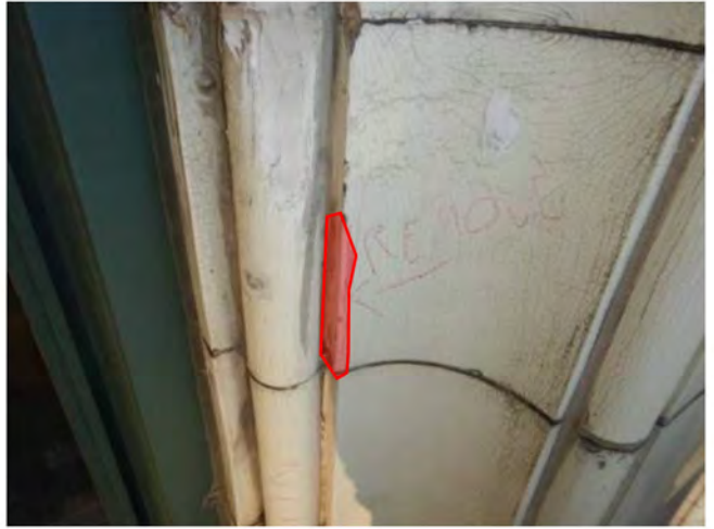
Photo 46: Remove loose & seal
