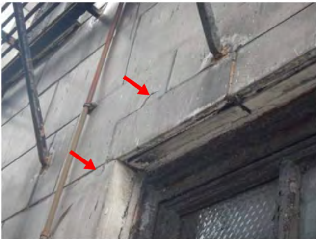
Photo 37: Remove loose + seal
