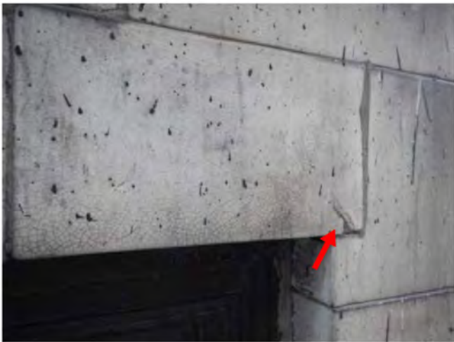
Photo 17: Remove loose + seal
