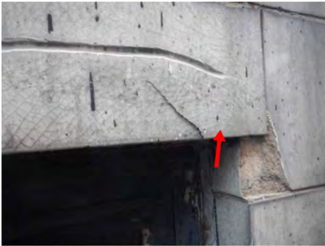
Photo 35: Remove loose + seal
