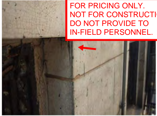
Photo 6: Remove loose + seal
