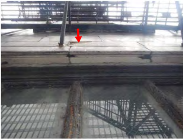
Photo 23: Remove loose + seal
