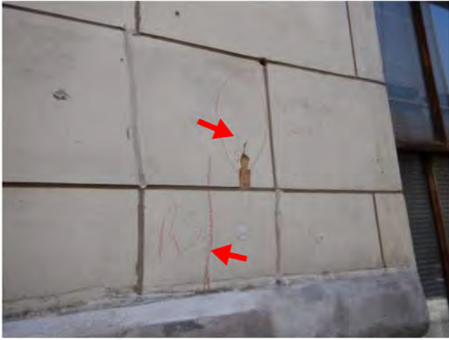
Photo 157: Remove loose & seal
