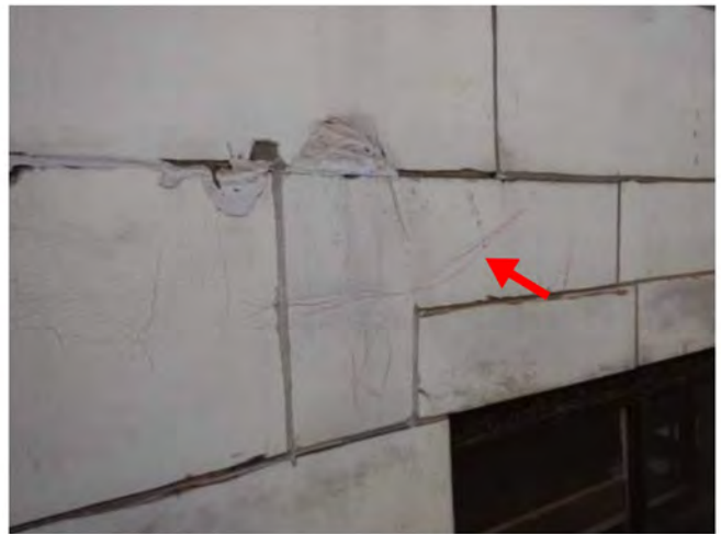
Photo 128: R/S or possible remove loose & seal
