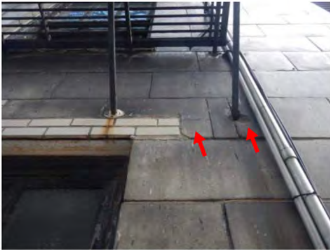
Photo 25: Remove loose + seal
