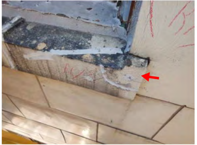
Photo 104: Remove loose & seal
