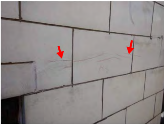
Photo 127: R/S or possible remove loose & seal
