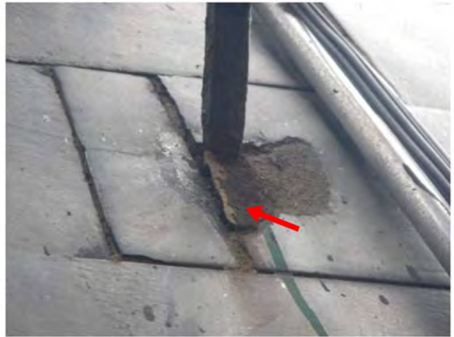
Photo 36: Remove loose + seal
