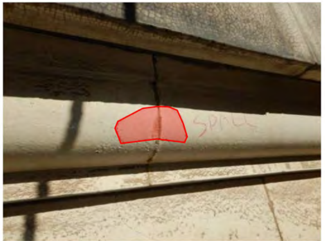
Photo 88: Remove loose & seal
