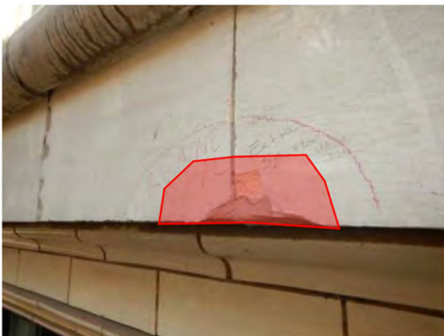
Photo 99: Remove loose & seal
