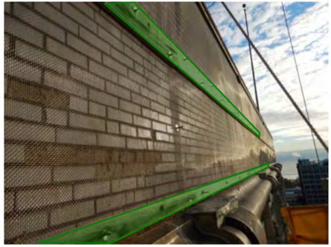
Photo 2: Replace 2x4 studs at mesh
