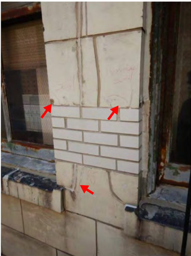
Photo 107: Remove loose & seal
