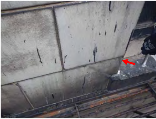
Photo 39: Remove loose + seal
