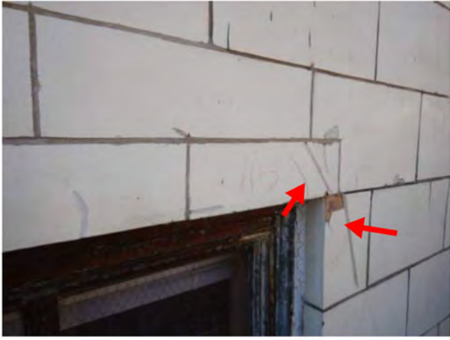
Photo 49: Remove loose + seal
