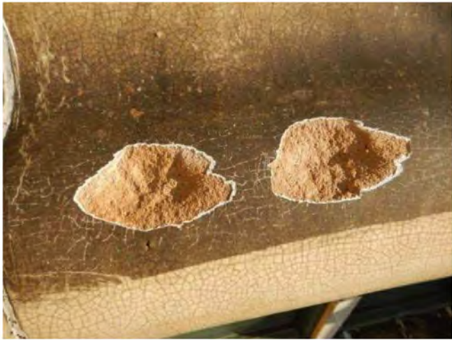
Photo 3: Seal exposed terra-cotta spalls
