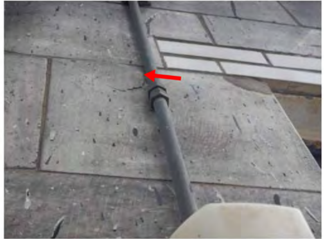
Photo 8: Remove loose + seal
