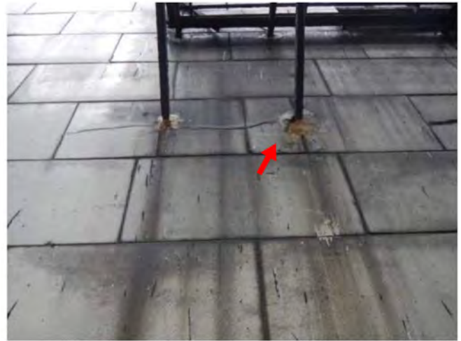
Photo 42: Remove loose + seal
