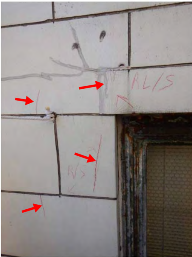
Photo 111: Remove loose & seal
