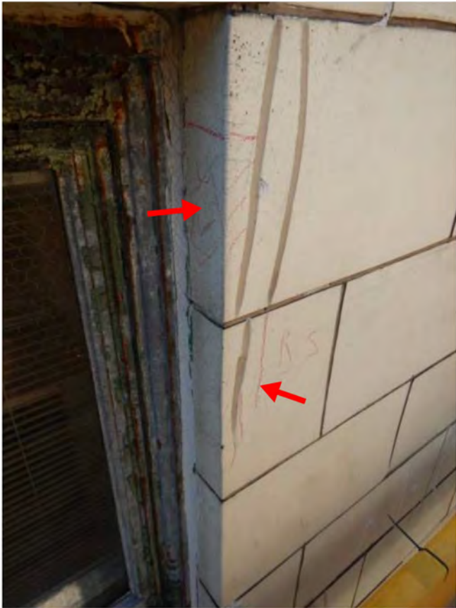
Photo 99: Remove loose & seal
