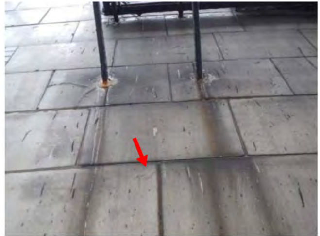
Photo 26: Remove loose + seal
