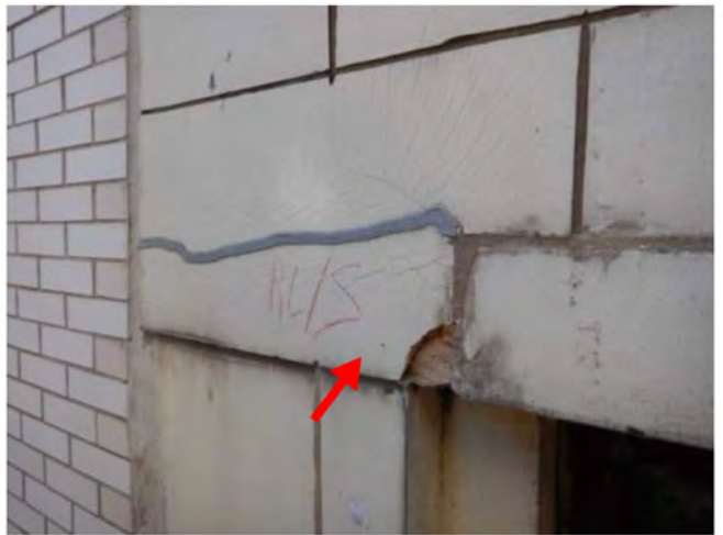
Photo 152: Remove loose & seal
