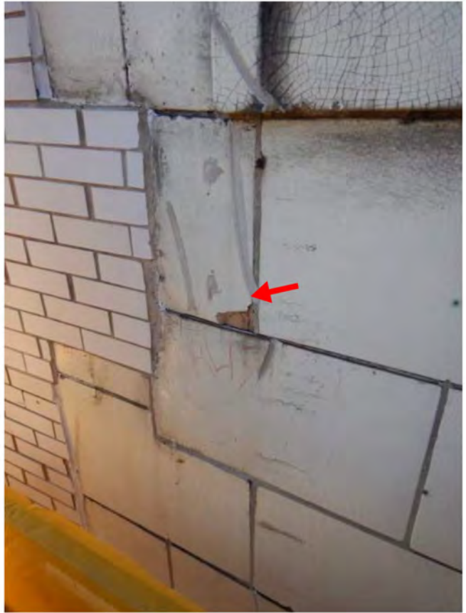
Photo 14: Remove loose + seal
