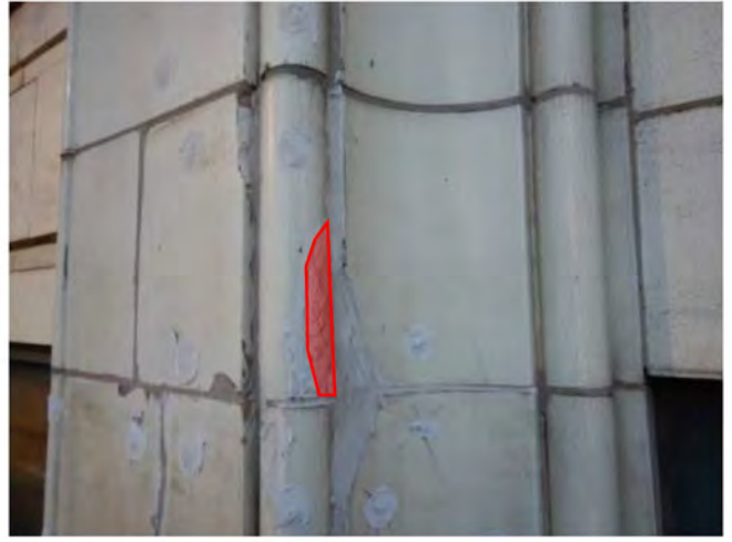
Photo 50: Remove loose & seal
