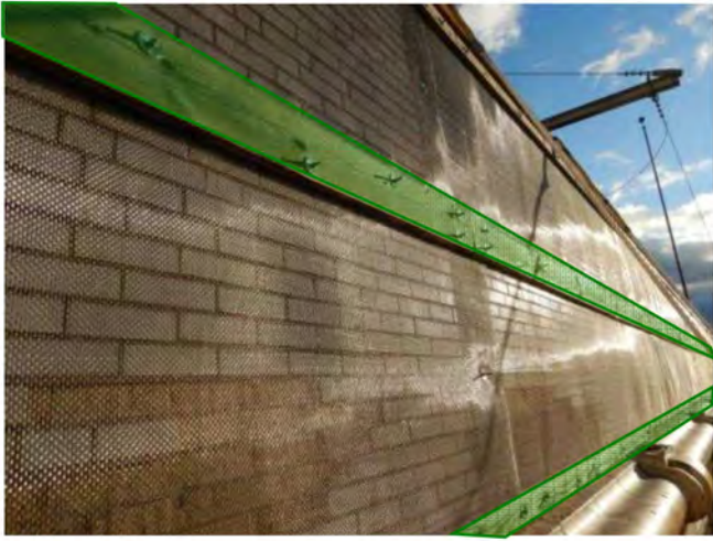
Photo 1: Replace 2x4 studs at mesh
