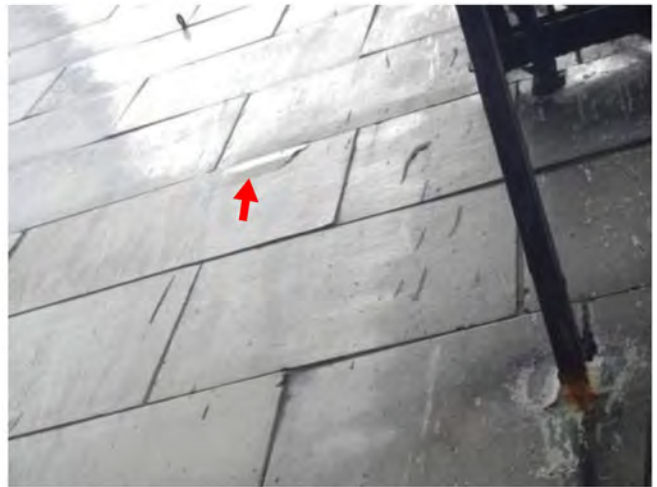
Photo 22: Remove loose + seal
