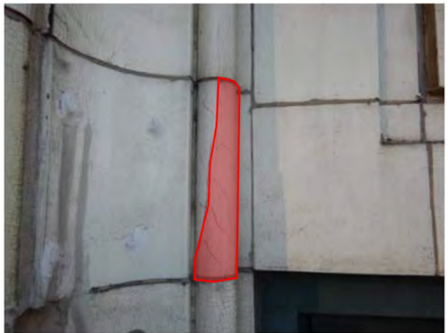
Photo 42: Remove loose & seal
