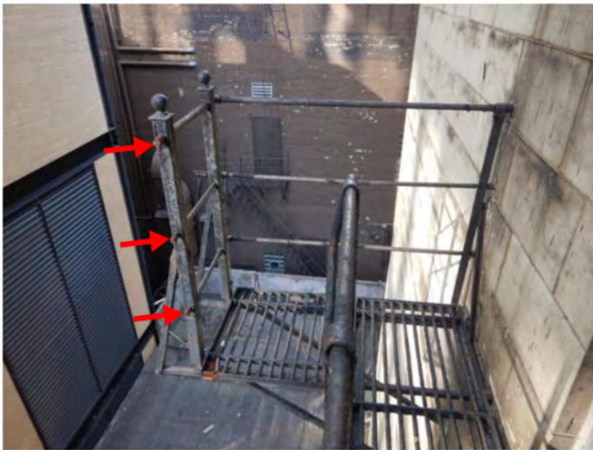
Photo 6: Item #6: Fall hazard at Level 4, install handrails
