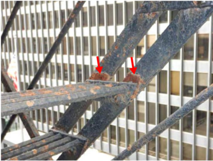
Photo 5: Item #5: Replace tread connection (weld or bolt)
