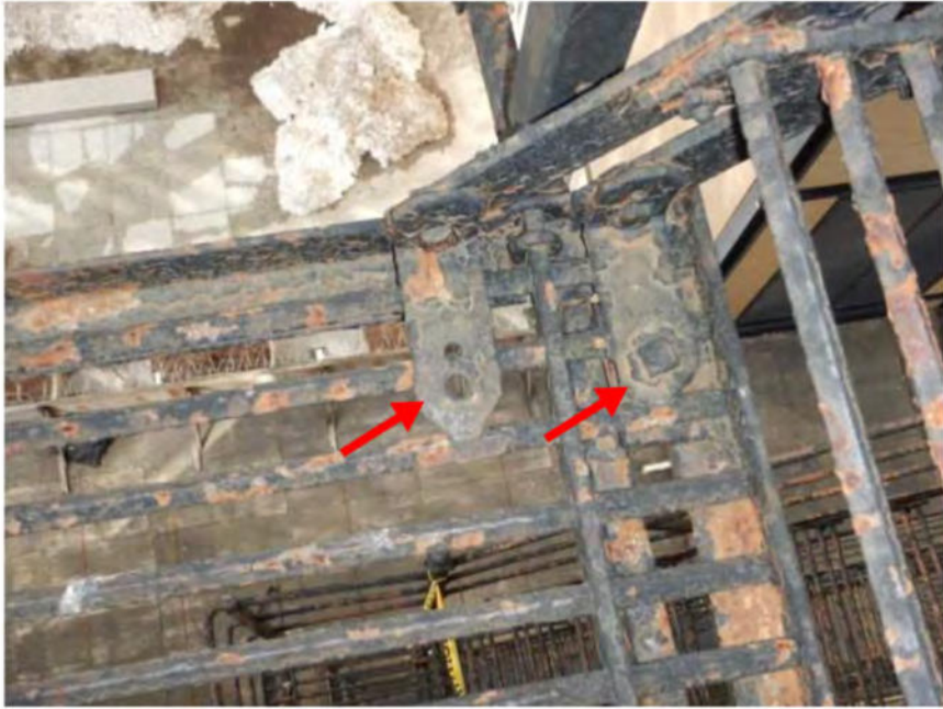
Photo 16: Item #15: Provide plate & bolt at stringer bottom connections (replace deteriorated components as needed)
