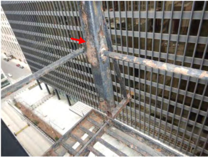
Photo 3: Item #3: Partial-replacement of handrail post (remove deteriorated components and weld new steel)
