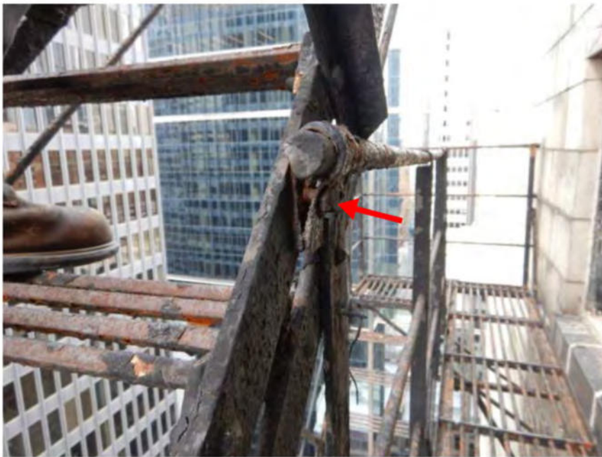
Photo 15: Item #14: Provide new handrail to stringer connection
