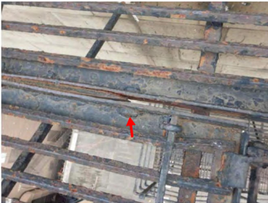
Photo 4: Item #4: Replace missing or deteriorated bolts
