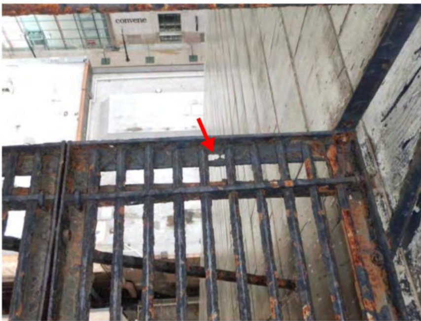
Photo 8: Item #8: Reinforce grating support angles with section loss
