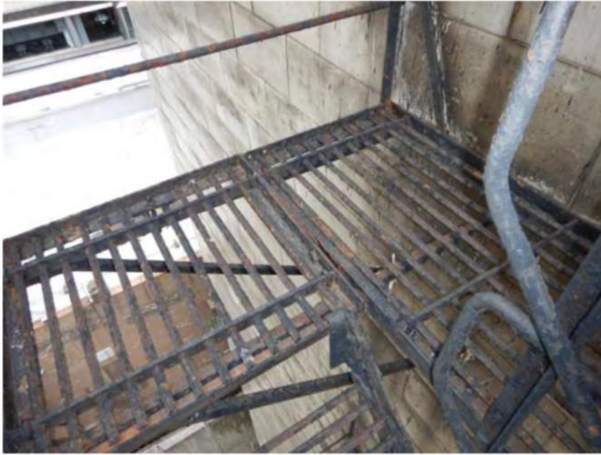
Photo 1: Item #1: Wire brush existing paint & provide new coating
