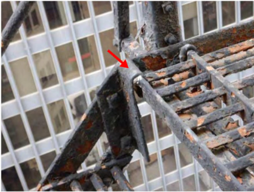
Photo 14: Item #13: Replace deteriorated stringer hook connection
