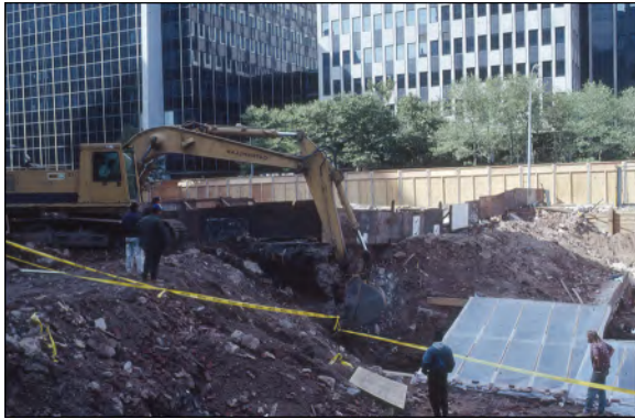
Figure 3. Backhoe clearing adjacent to temporary archaeological excavation shelter early in the fieldwork. (photograph by Dennis Seckler) (from Volume 2, Part 1 [Howson, Bianchi, and Perry 2009:Figure 3]).
