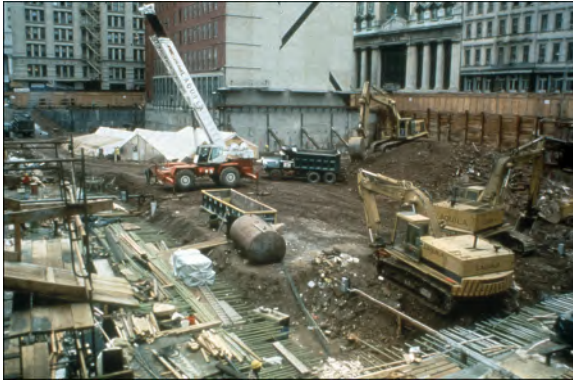
Figure 4. Construction of the 290 Broadway Federal building proceeded during the archaeological fieldwork. The archaeological excavation shelter is visible at the rear. The view is toward the southeast (photograph by Dennis Seckler) (from Volume 2, Part 1 [Howson, Bianchi, and Perry 2009:Figure 6]).
