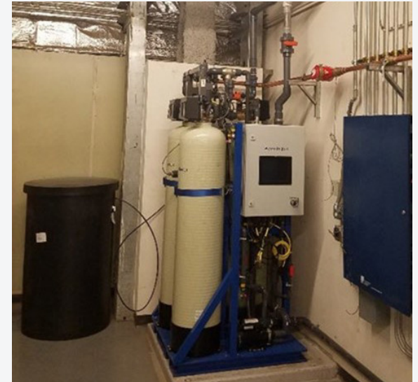
AWT system setup at Lloyd D. George Courthouse. Photo credit Gregg Tomberlin, NREL
