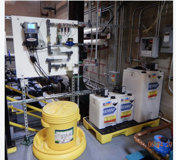
Chemical containers and side stream filtration system used by the chemical scale inhibition system. Photo credit Doug Baughman, GSA
