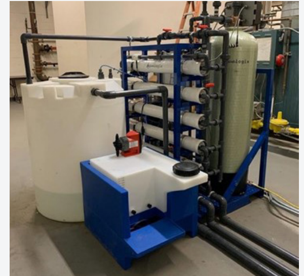
The skid-mounted blowdown recovery system is located in the chiller room at the Lloyd D. George U.S. Courthouse. Photo credit Aqualogix
