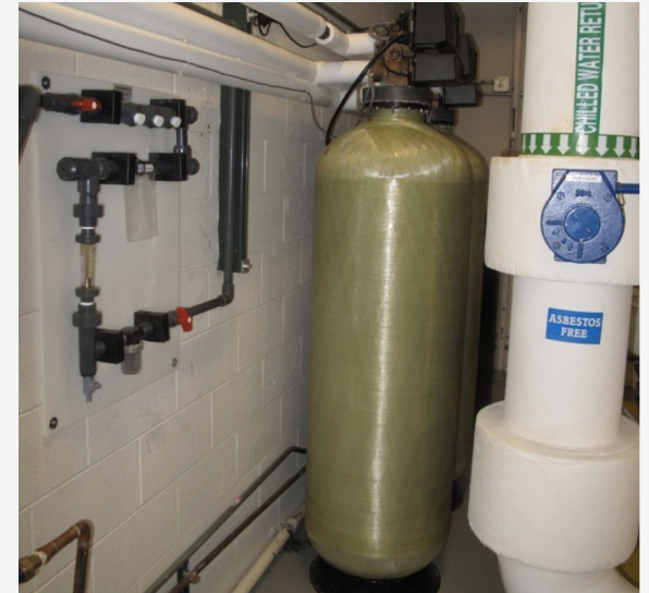
Tanks for treating the make-up water entering the AWT system at Denver Federal Center Building 25, in Denver, CO. Photo credit Dylan Cutler, NREL
