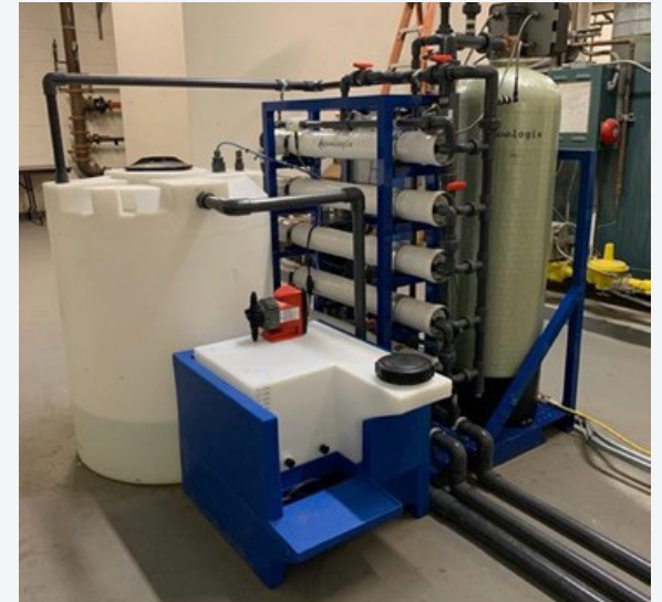
The skid-mounted blowdown recovery system is located in the chiller room at the Lloyd D. George U.S. Courthouse. Photo credit Aqualogix
