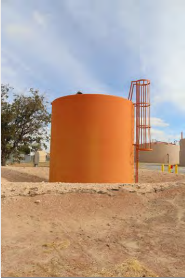
Figure 249. Diesel Tank, 20,000-gallon capacity, looking southeast.
