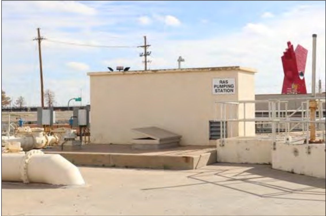
Figure 264. RAS Pumping Station, looking south.
