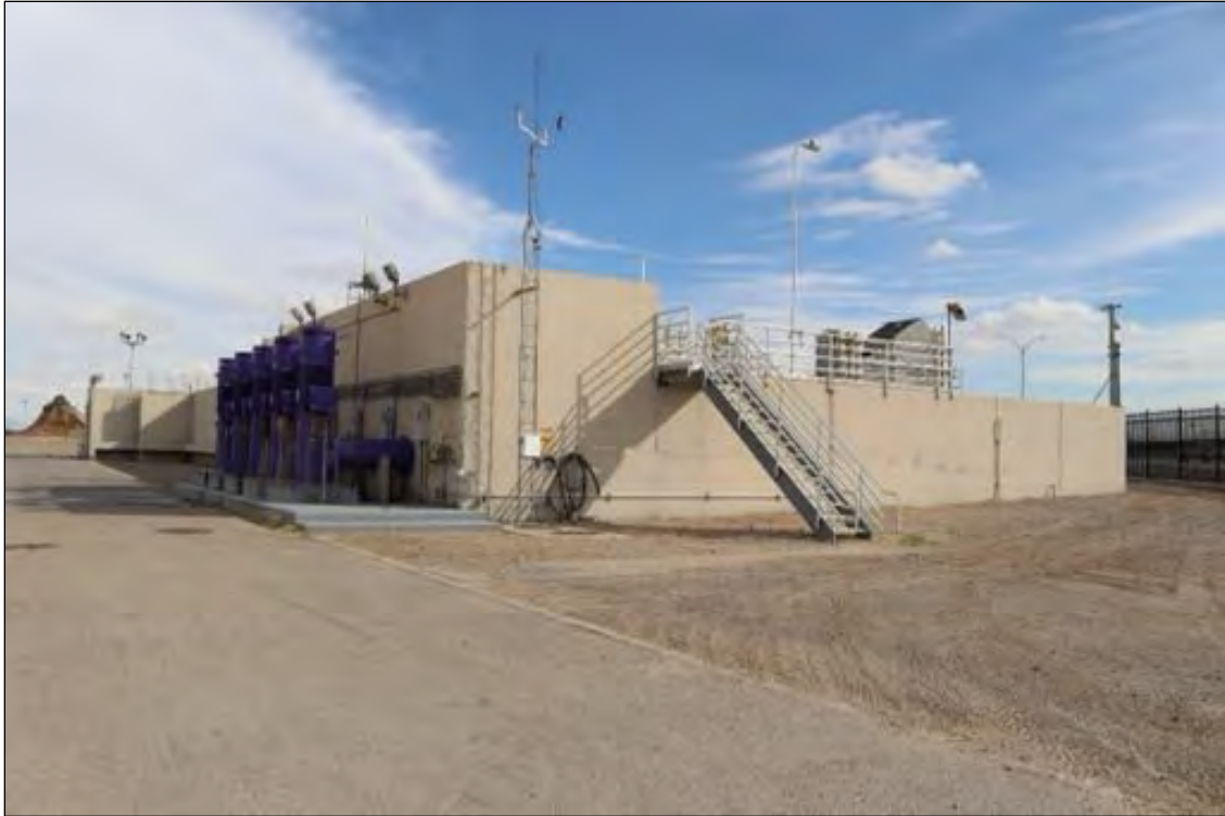
Figure 266. Effluent Pump Station and Filters, looking southeast.
