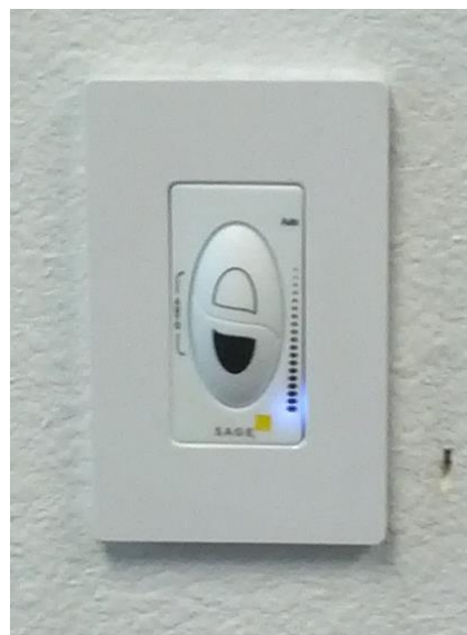
Figure IV-6. The window tint within a zone can be controlled with wall switches such as this one. The blue light indicates the tint that the zone is manually set to (or automatic control).
