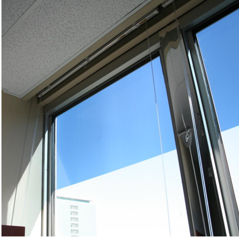
Figure IV-9. Aluminum cover plates were installed to conceal the wires coming out of the window frames.
