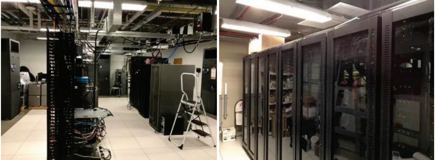
Figure 4: Showing second-floor (left) and fourth-floor (right) server rooms. Source: Dylan Cutler, NREL
