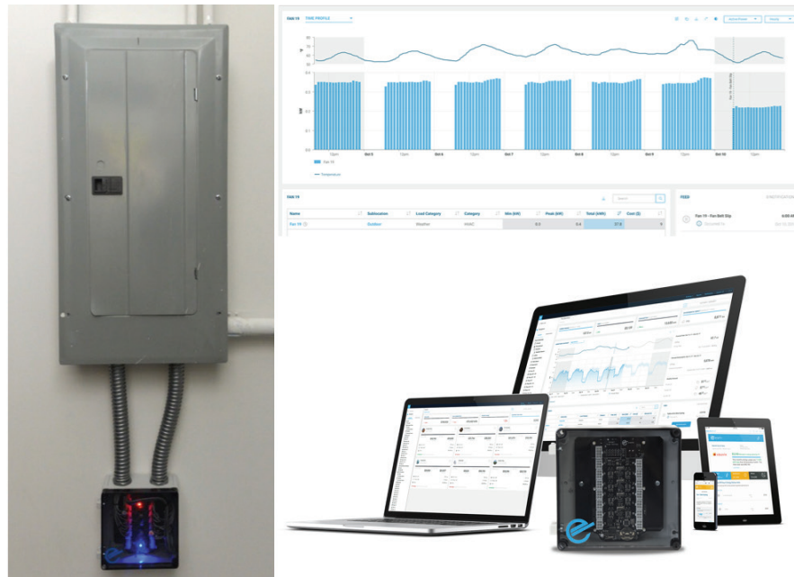
Figure 1: Sample CLASP installation configuration (left; source: Enertiv). Cloud analytics and front web (right; source: Enertiv).
