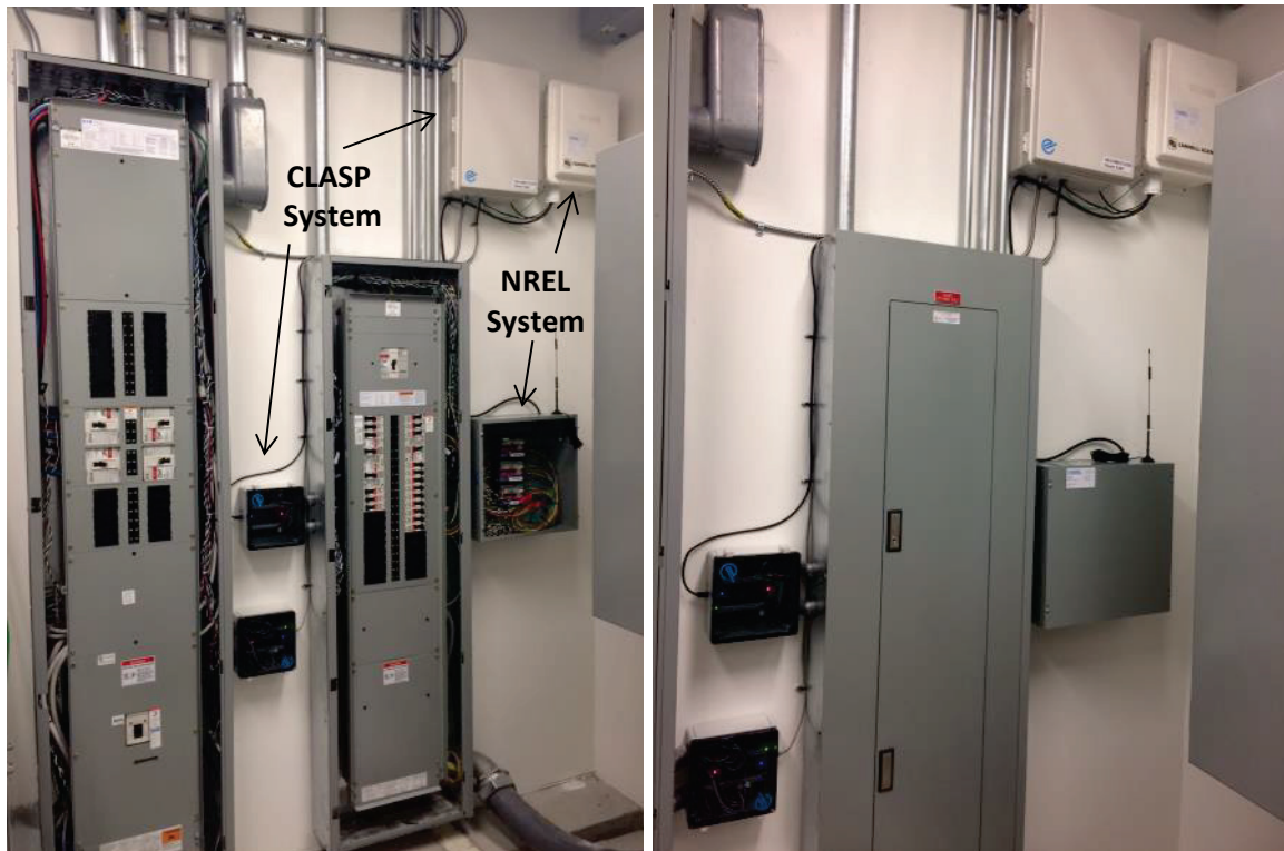
Figure 7: Installation in the second-floor electrical room. Panel H20E1 is shown in the center of each image (in progress on the left; completed install on the right). Source: Dylan Cutler, NREL
