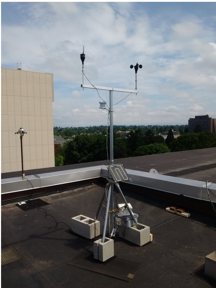
Figure C.6. Weather instruments. To the left, the global and diffuse horizontal irradiance sensor is mounted on a pre-existing metal platform, atop a pole. Wind, temperature and relative humidity sensors are mounted on a tripod-base structure, shown at the center of the image. The structure also holds a solar panel for powering the data acquisition system (white box under tripod).
