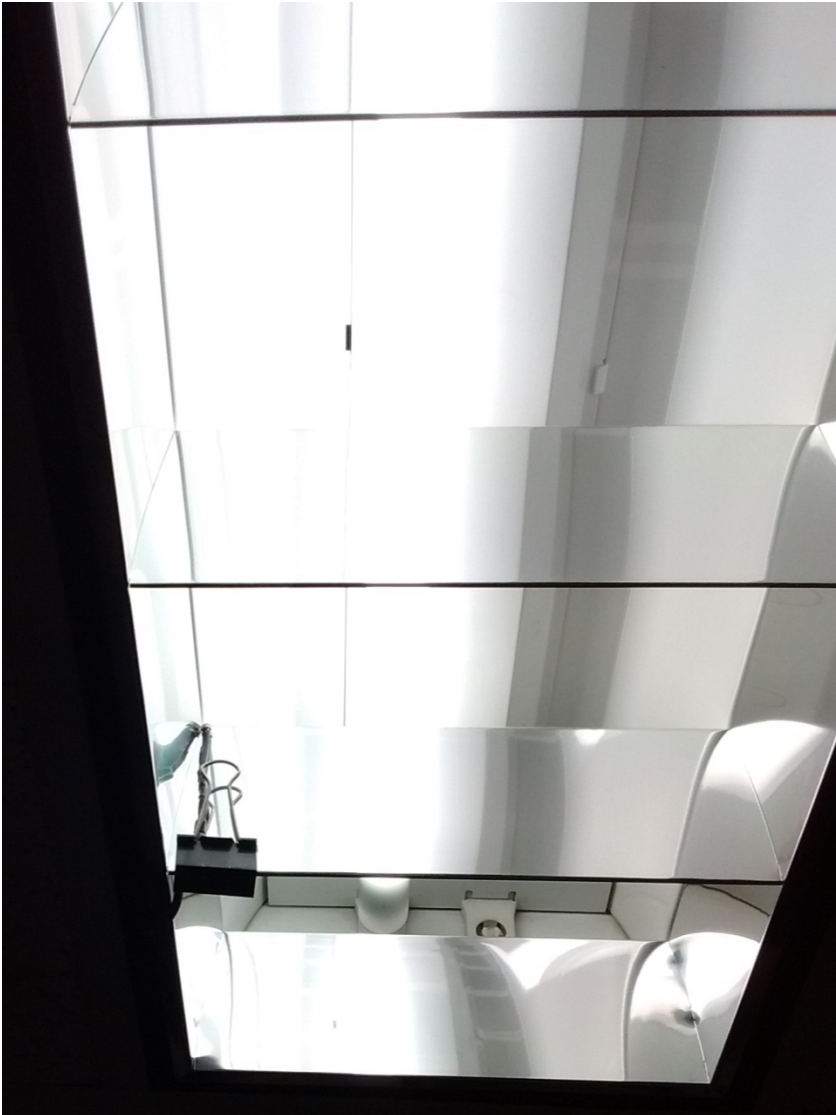
Figure C.2. Luminaire photoresistor sensor.
