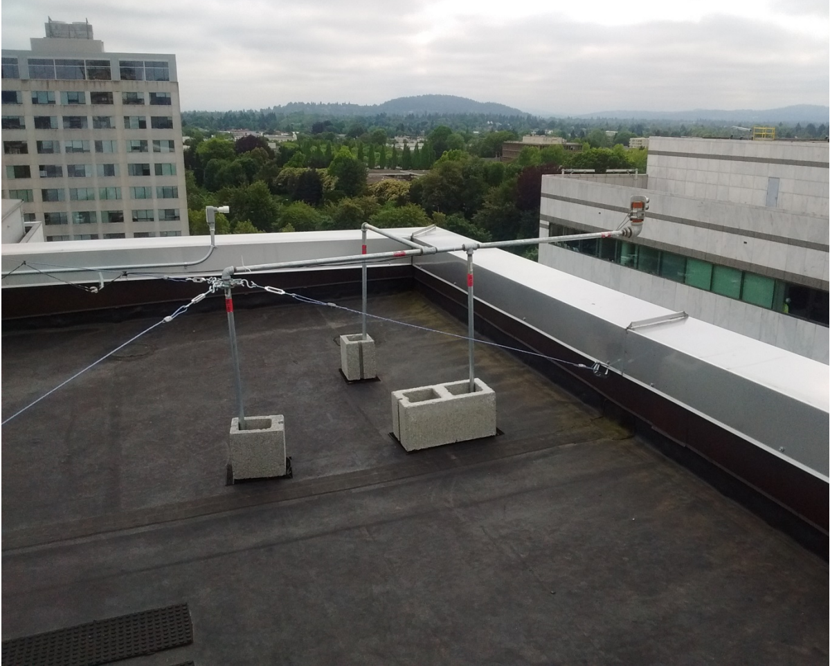
Figure C.5. Exterior vertical irradiance and illuminance sensors. These sensors face due south, and are mounted over the edge of the south façade of the building's service core. They are mounted on a steel tube structure, secured with steel cables and weighted down by cinder blocks. The image was taken facing approximately ESE. South is to the right of the picture, approximately.
