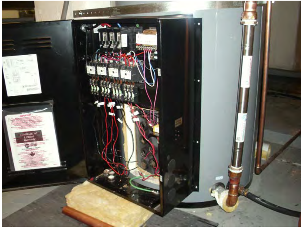
Figure 6. Final Configuration for the Nonchemical Water Treatment System (silver section of pipe on the cold water inlet to the water heater tank).
