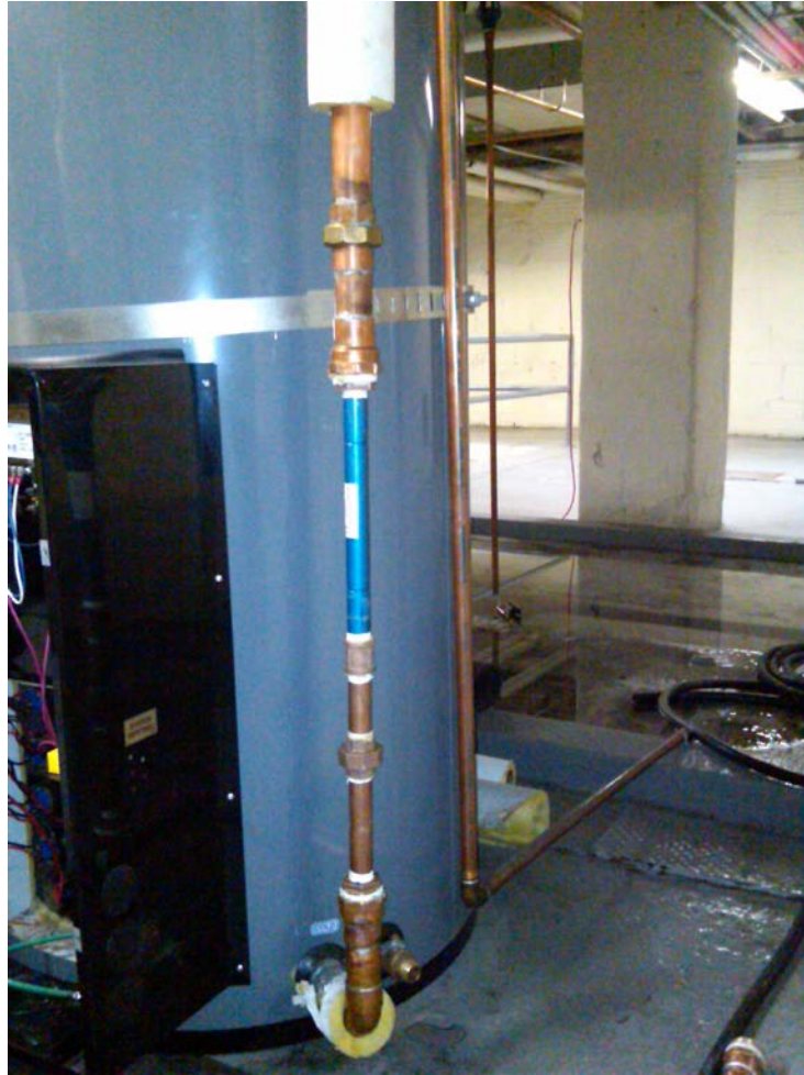
Figure 9. Electric Water Heater Showing the 0.75 in. Device (blue) Installed on the Cold Water Inlet Pipe.
