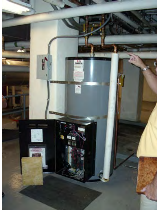
Figure 2. Electric Water Heater Where Test Was Conducted.
