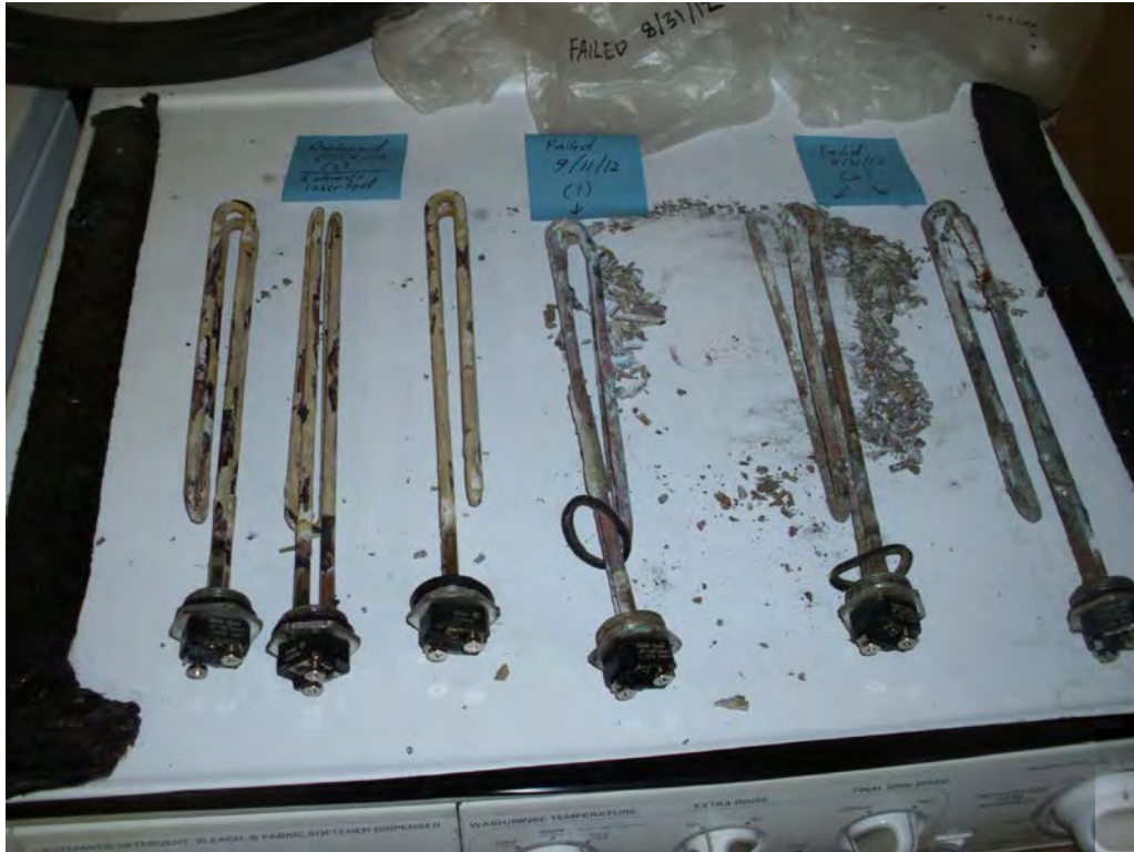
Figure 5. All Six Heating Elements Removed from the Electric Water Heater During a Repair Session.
