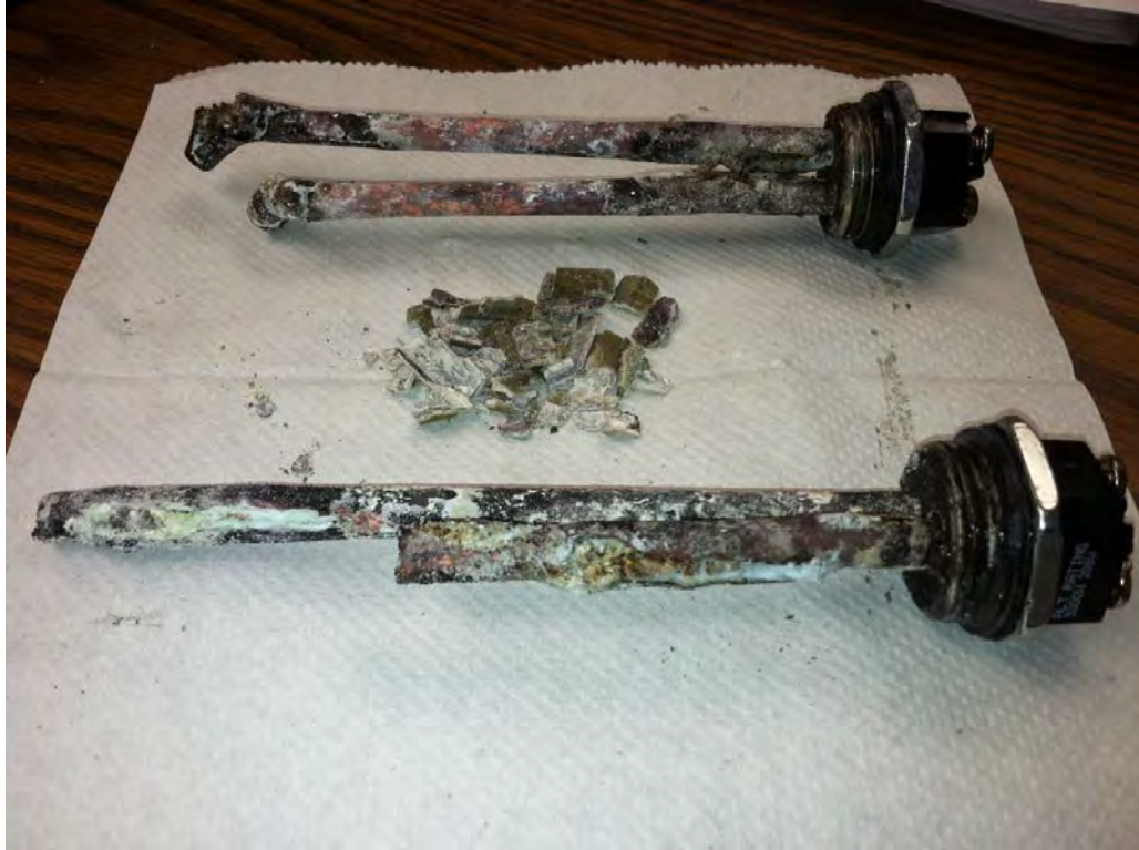
Figure 7. Two of the Three Failed Heating Elements from December 2012.
