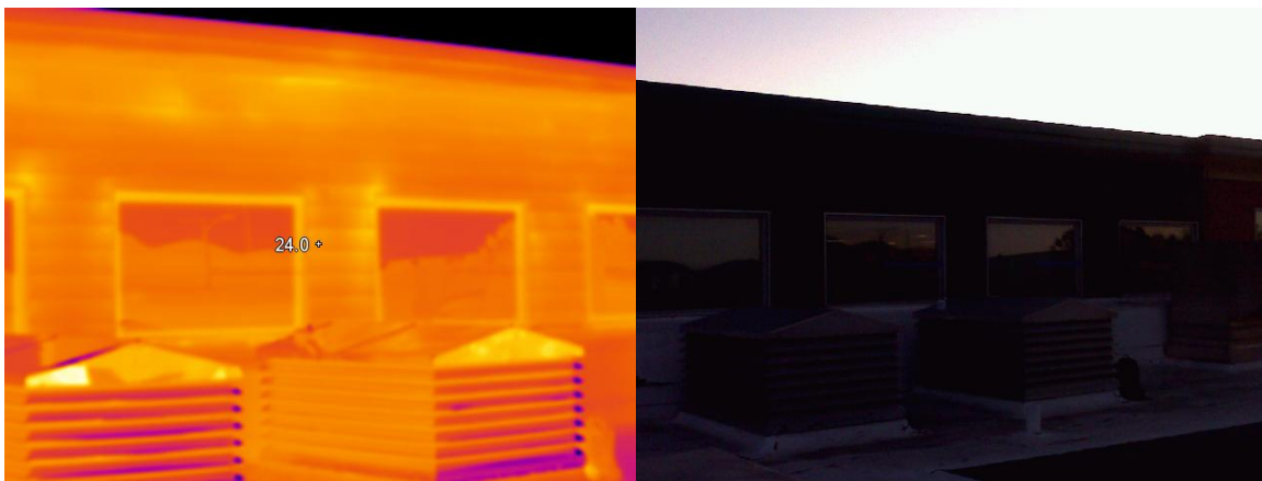
Figure 22: IR image (left) of the two windows outside and the visual photo (right) of the same location
