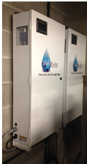
Figure 5: Building 95 Alternative Water Treatment System
