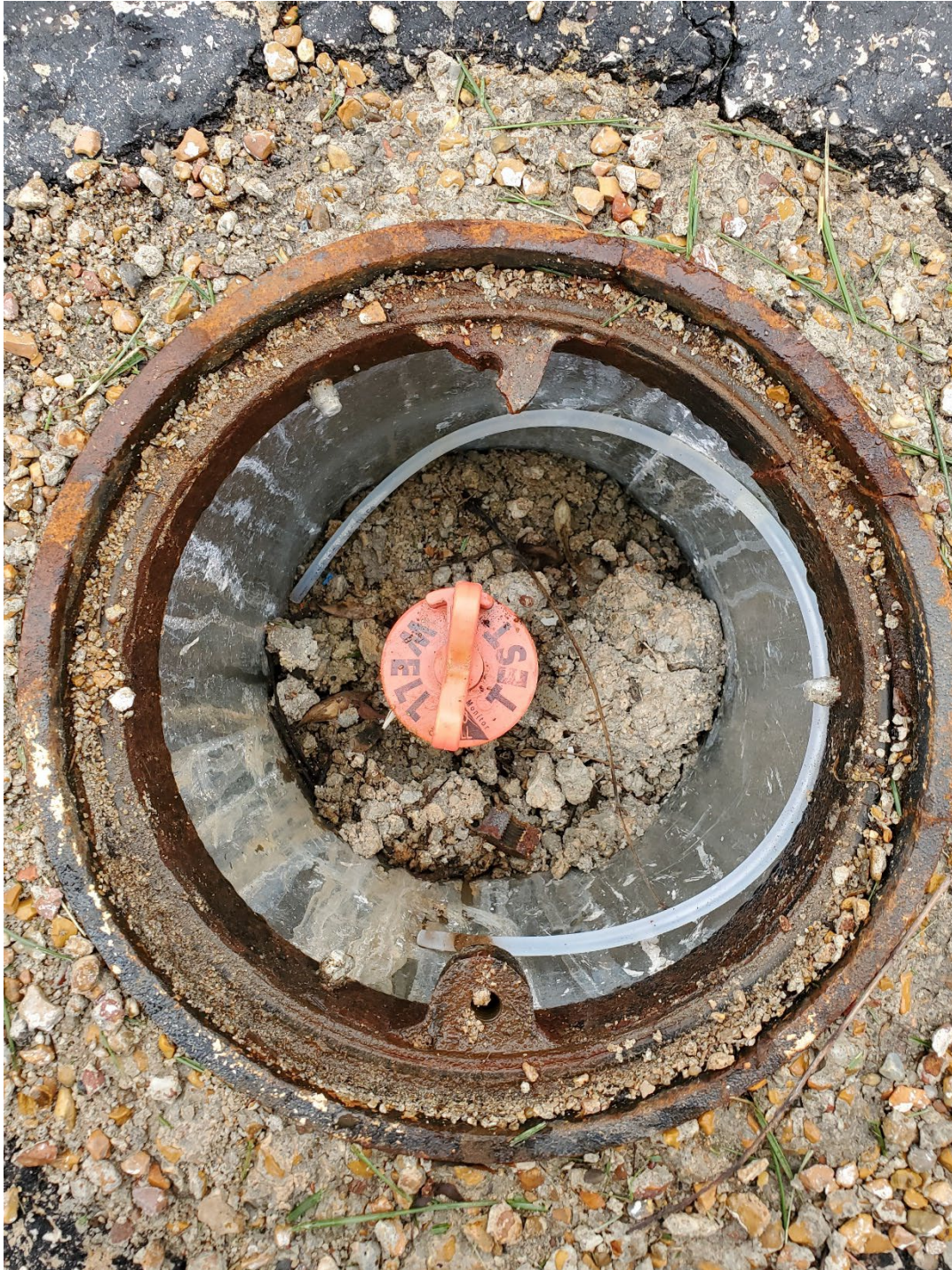
Photo of Monitoring Well MW-15 shows a crack in the well vault and the broken threaded bolt flange.
