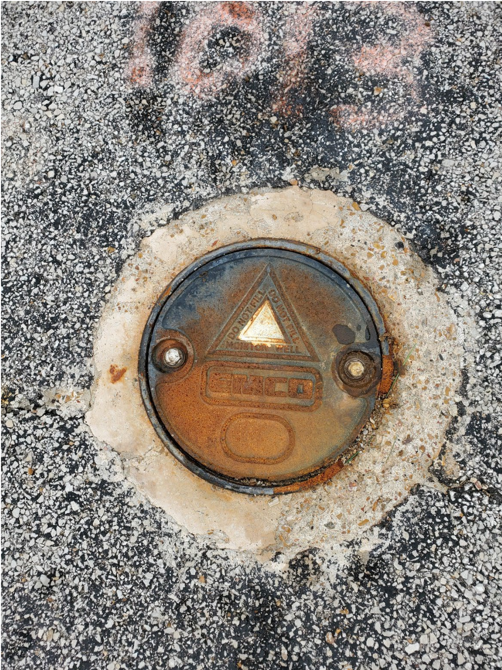
Photo shows the rim of the well vault for Monitoring Well MW-14 to be broken off.
