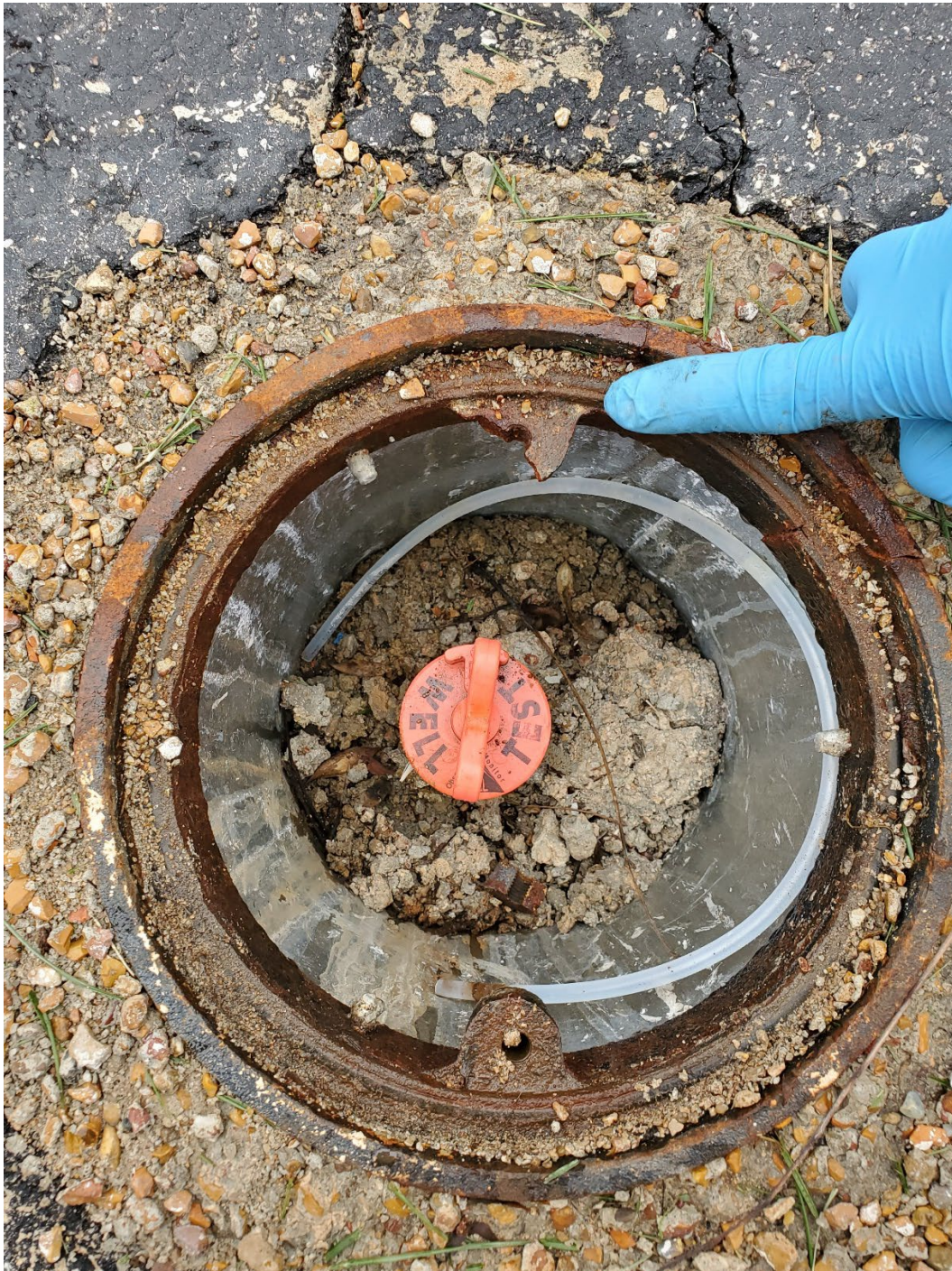
Photo shows a finger pointing out the broken treaded bolt flange for Monitoring Well MW-15.
