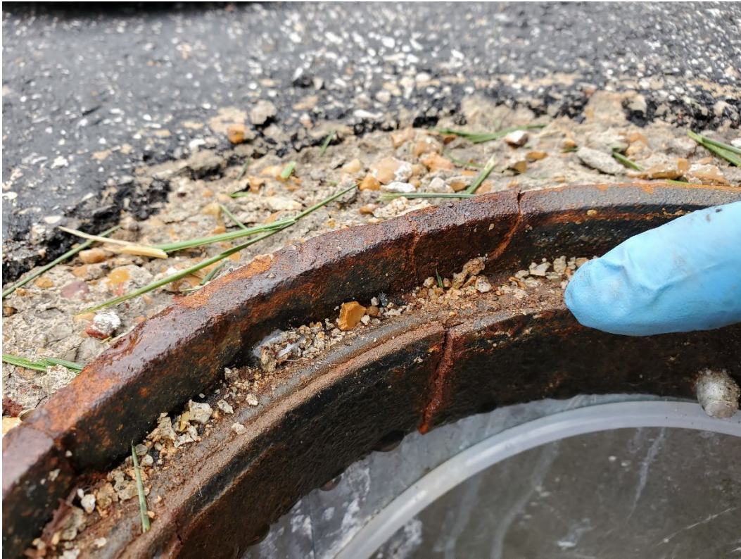
Photo shows a finger pointing toward the cracked well vault for Monitoring Well MW-15.
