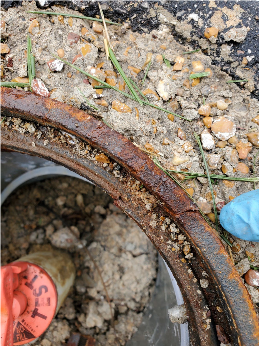
Photo shows a finger pointing toward the cracked well vault for Monitoring Well MW-15.
