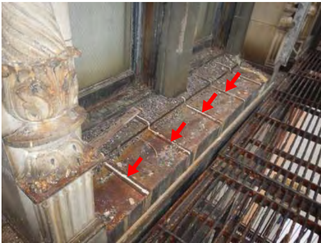
Photo 149: R/S failed joints
