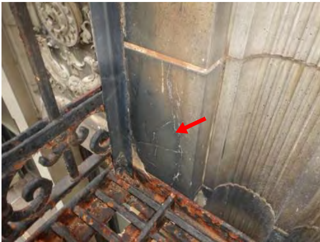
Photo 139: Remove loose + seal
