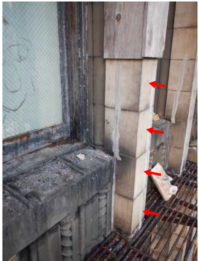
Photo 74: R/S cracks + install wood
