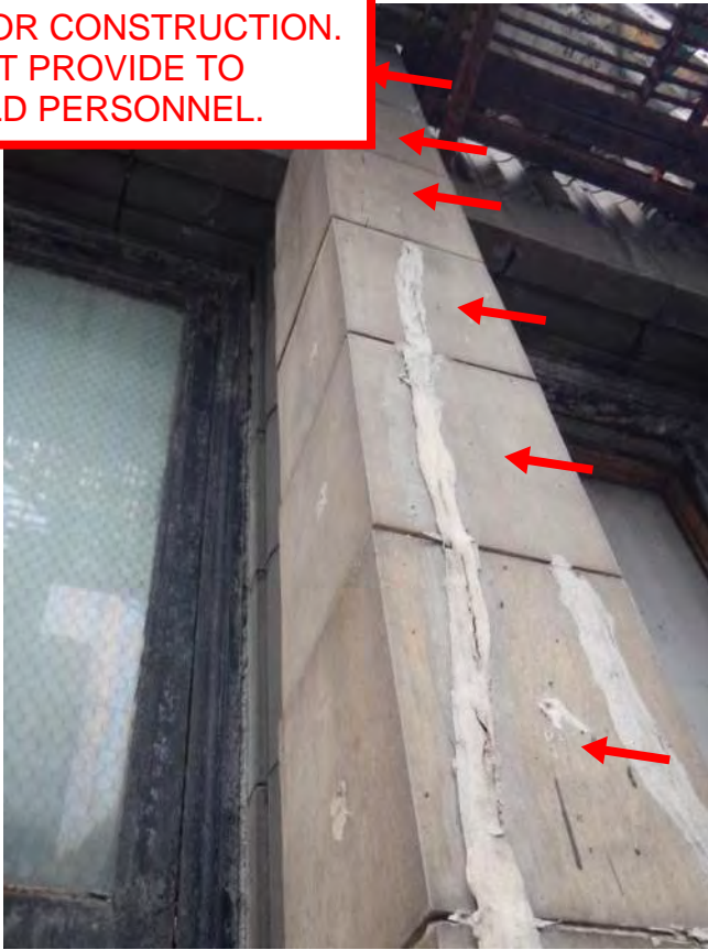
Photo 117: R/S cracks + install mesh or strap
