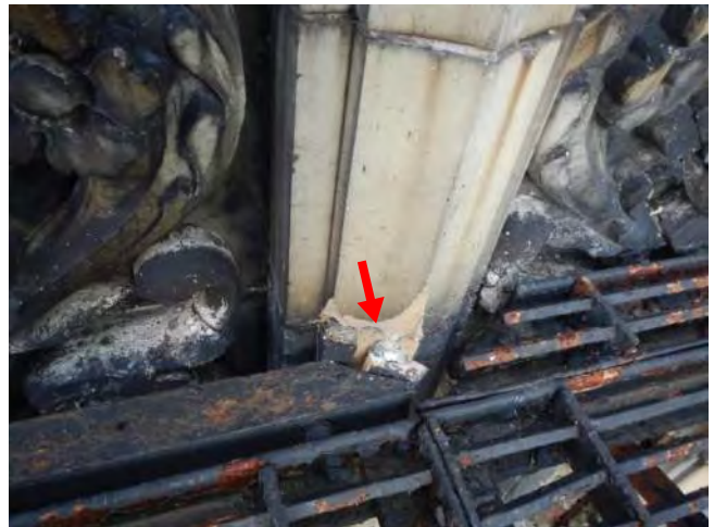
Photo 38: Remove loose + seal
