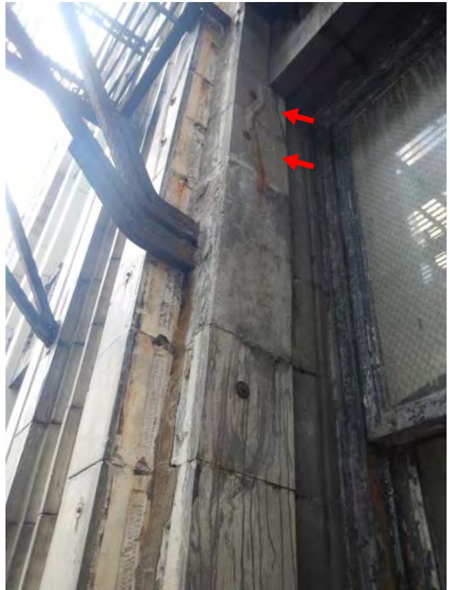
Photo 98: R/S cracks + install mesh or straps
