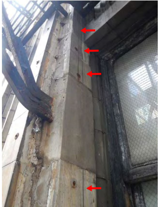
Photo 82: R/S cracks+ install mesh or straps
