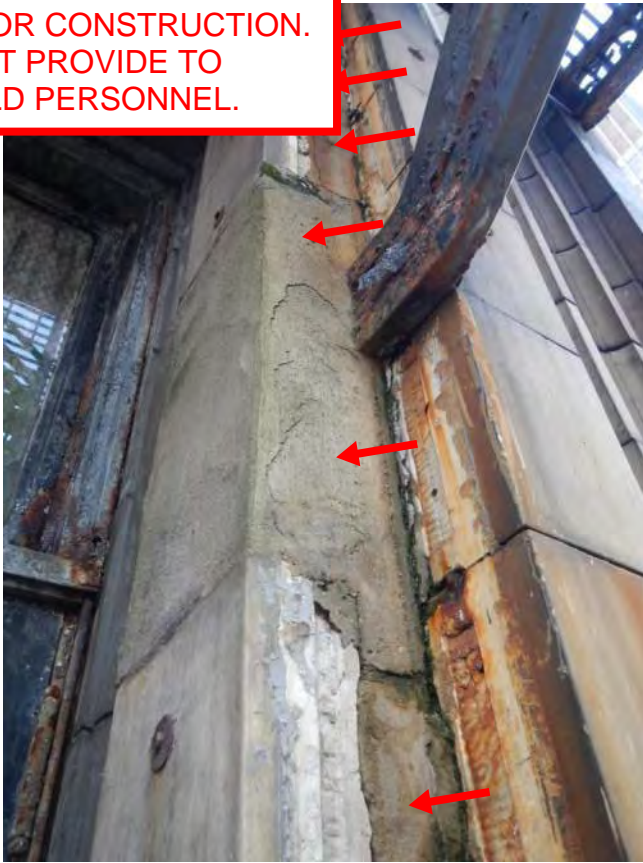
Photo 71: Remove loose + seal
