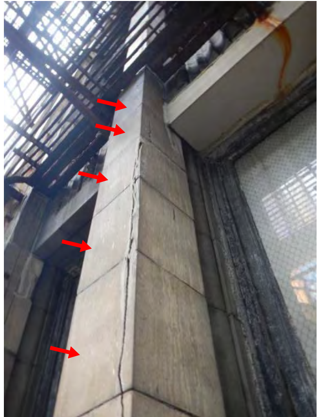
Photo 78: R/S cracks + install mesh or straps
