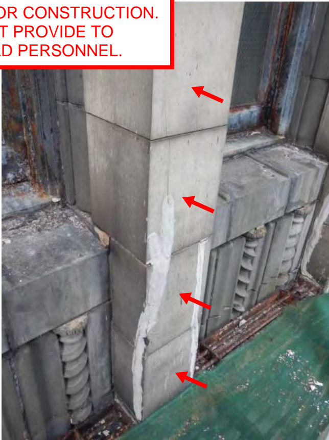
Photo 105: R/S cracks + install mesh or straps
