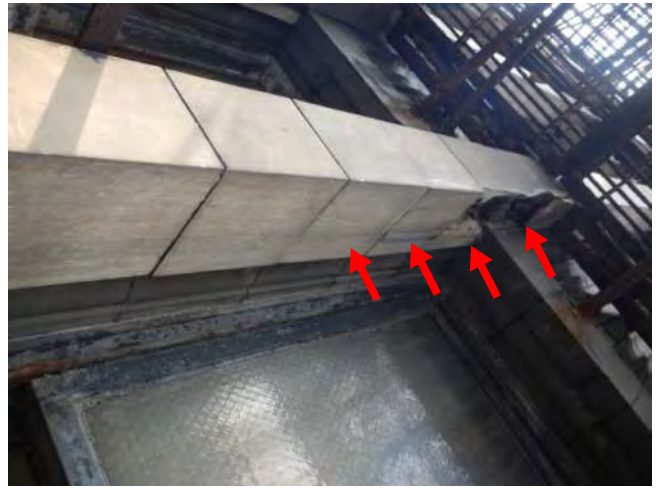
Photo 88: R/S cracks+ install wood
