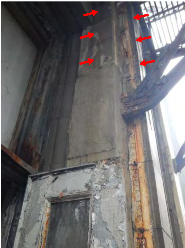
Photo 115: R/S cracks + install mesh or strap
