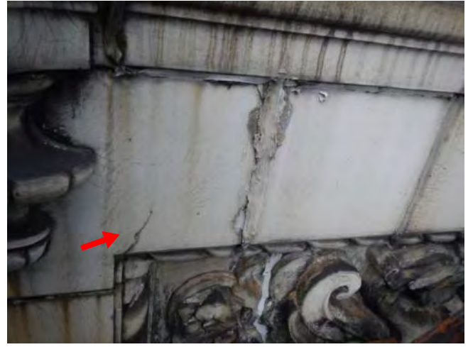
Photo 10: Remove loose + seal
