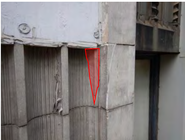
Photo 47: Remove loose & seal
