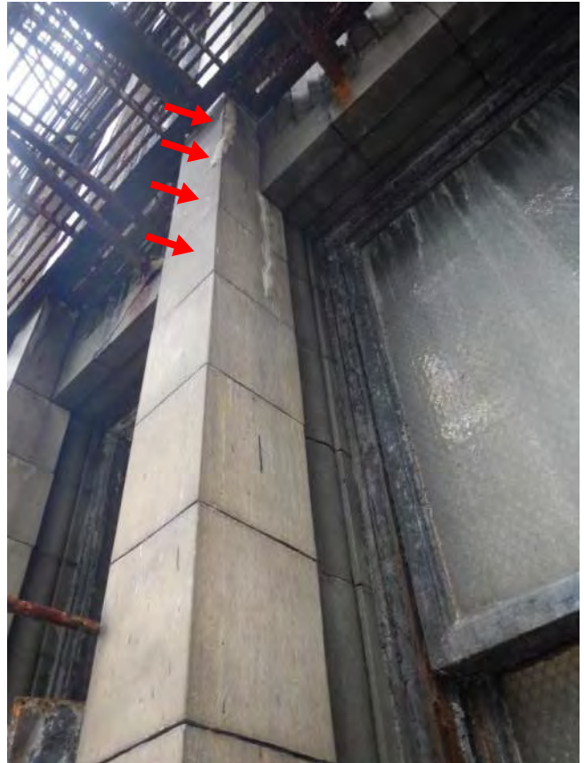
Photo 104: R/S cracks + install mesh or straps
