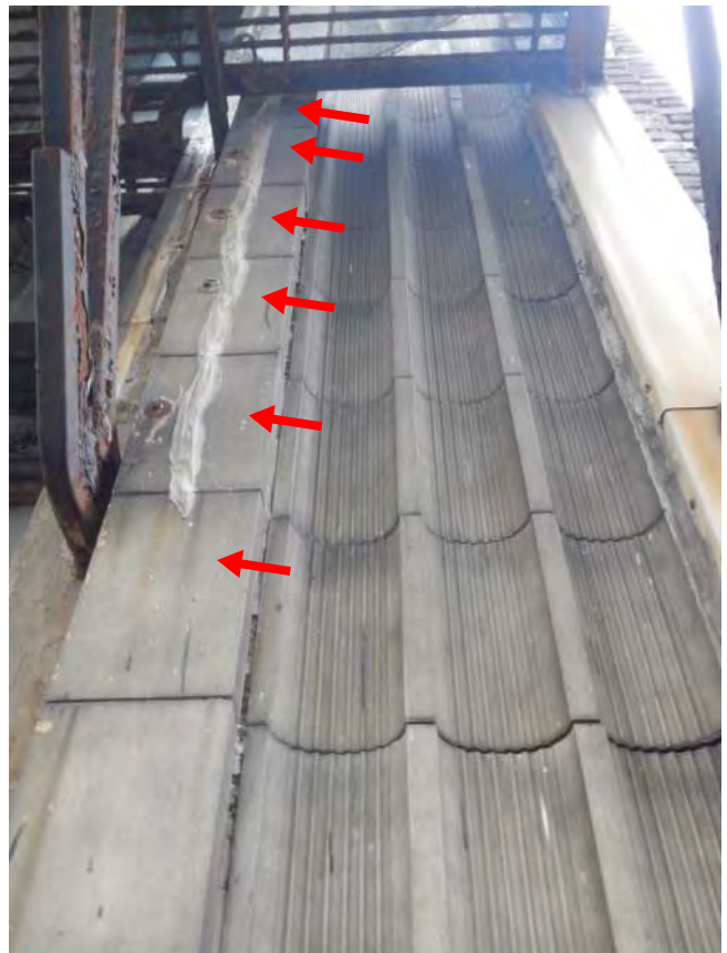
Photo 116: R/S cracks + install mesh or strap
