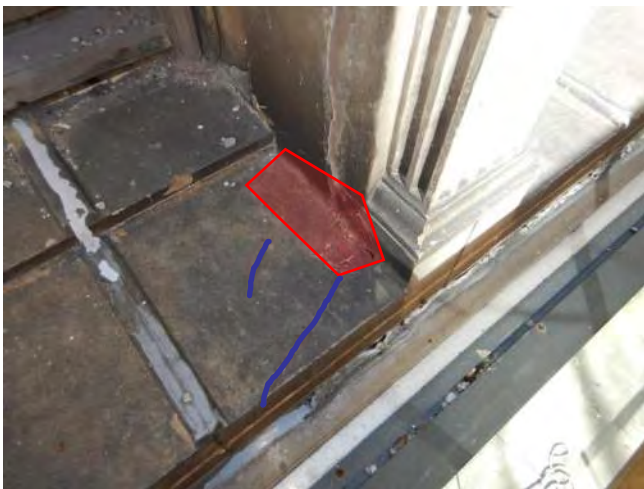
Photo 153: Remove loose + seal
