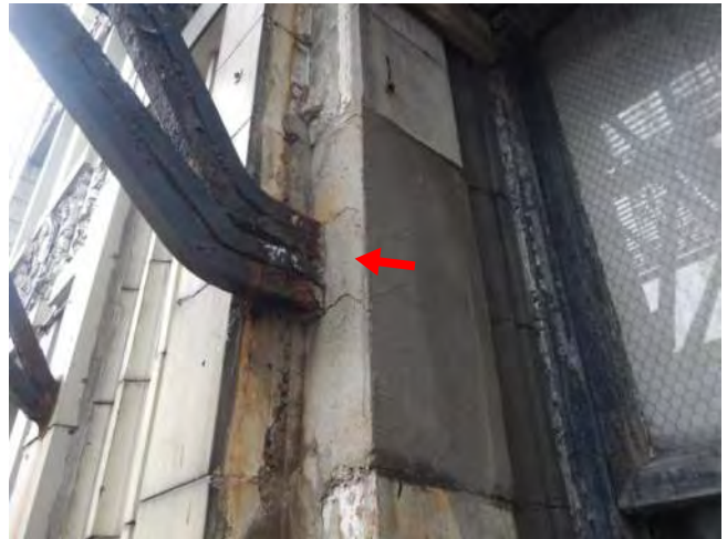
Photo 54: Remove loose + seal
