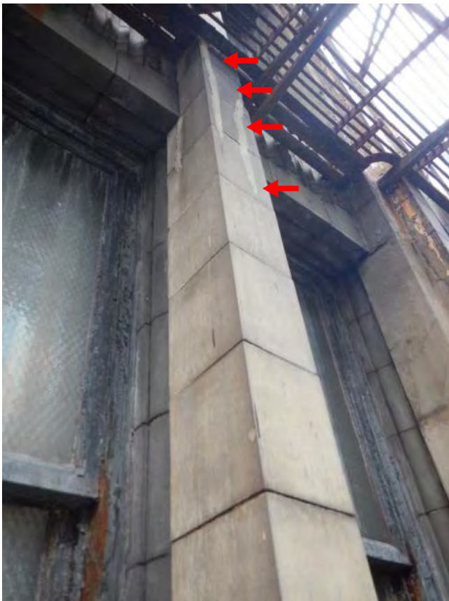
Photo 99: R/S cracks + install mesh or straps
