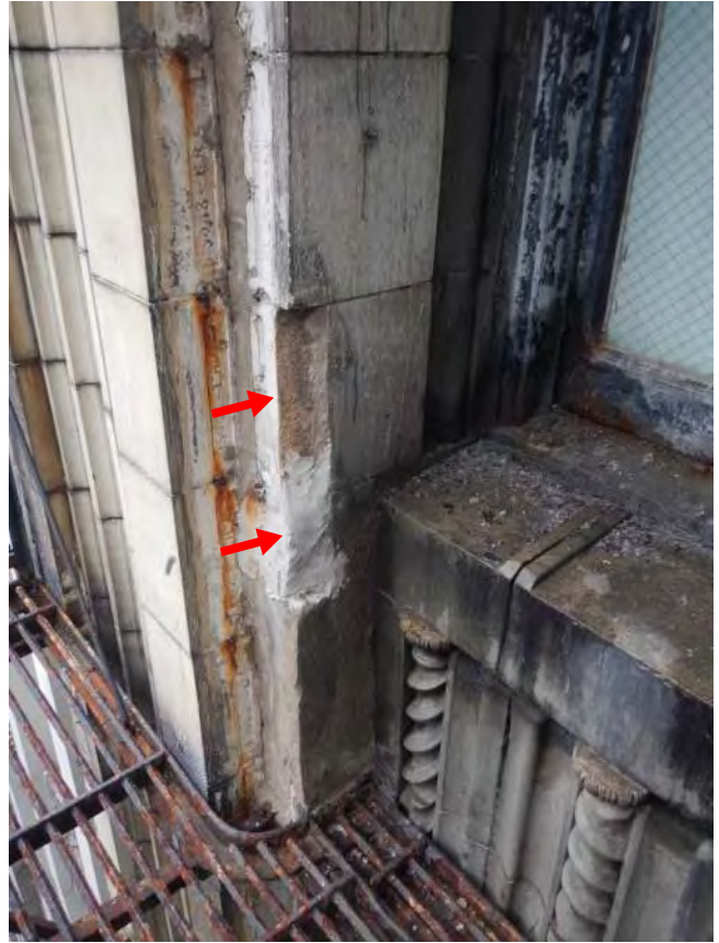
Photo 68: Remove loose + seal
