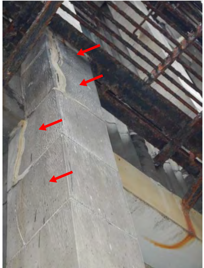
Photo 136: R/S crack + install mesh or strap
