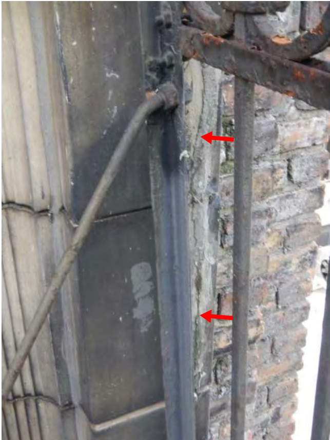
Photo 85: R/S cracks+ install mesh or straps
