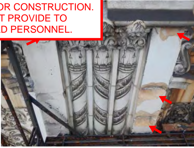
Photo 9: Remove loose + seal
