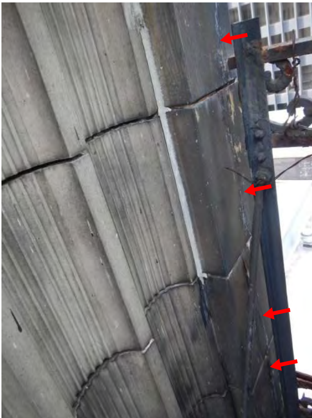
Photo 107: R/S cracks + install mesh or straps
