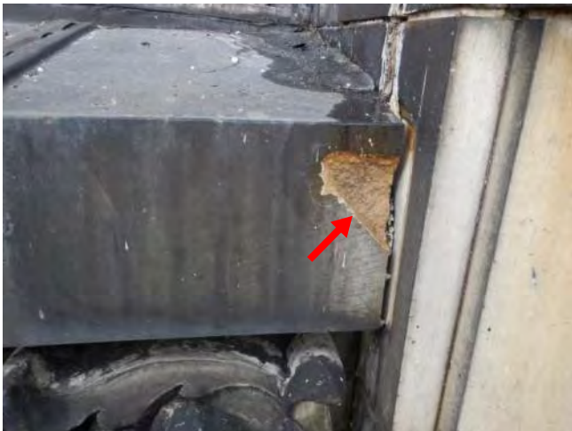
Photo 37: Remove loose + seal
