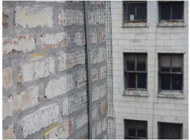
Photo 4: Replace missing anchors at existing mesh, TYP
