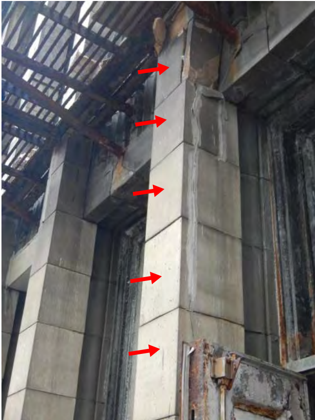
Photo 77: R/S cracks + install wood
