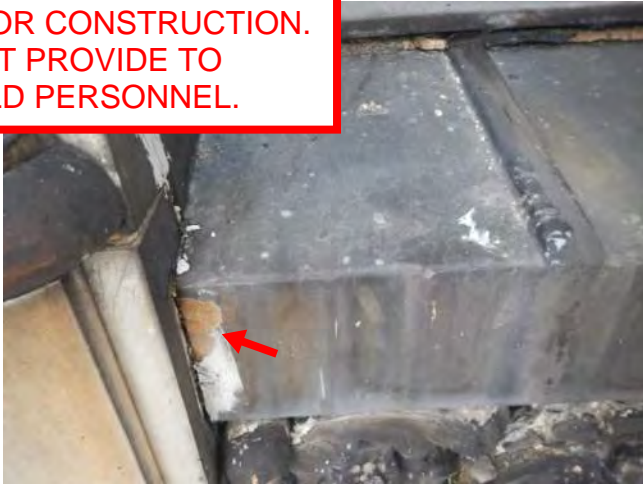
Photo 39: Remove loose + seal
