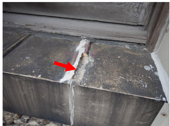
Photo 18. Typical spall on spandrel window sill terra cotta unit.
