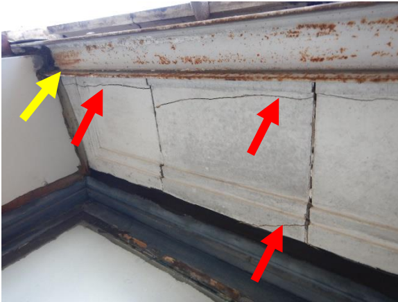
Photo 13. New underside cracks (red arrows) at terra cotta window head units (metal channel noted by yellow arrow).
