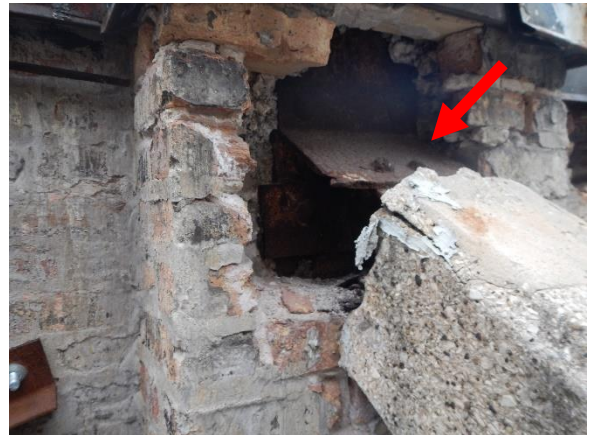
Photo 34. Exposed steel column at north elevation parapet. Exposure has led to extensive section loss due to corrosion.
