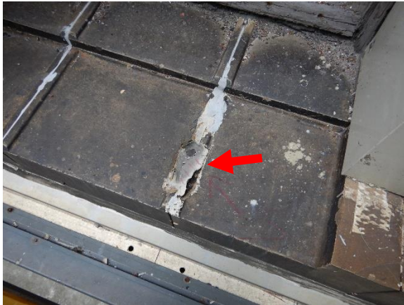
Photo 27. Failed sealant at skyward facing joint.
