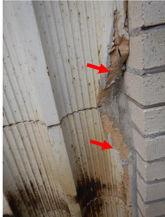
Photo 24. Spalled terra cotta units at column.
