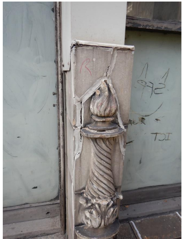
Photo 22. Mullion units at 3rd floor in extremely poor condition, marked for removal.
