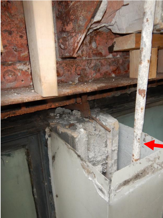
Photo 41. Section loss due to corrosion noted on steel hanger rod (red arrow).
