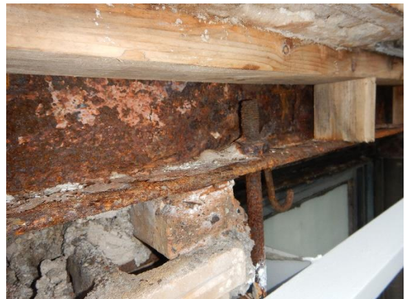
Photo 50. Extensive surface corrosion and rust jacking observed on existing steel elements.
