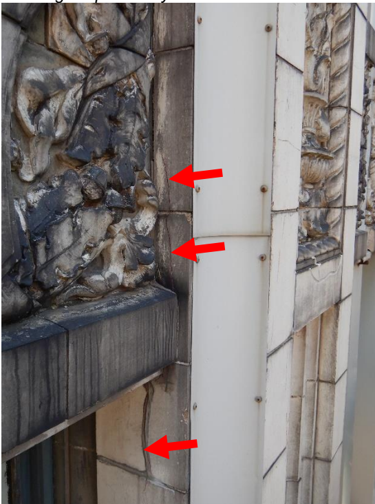
Photo 25. Cracked terra cotta units at jamb return.
