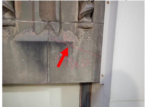
Photo 16. Typical diagonal crack observed on most terra cotta window head units (red arrow).
