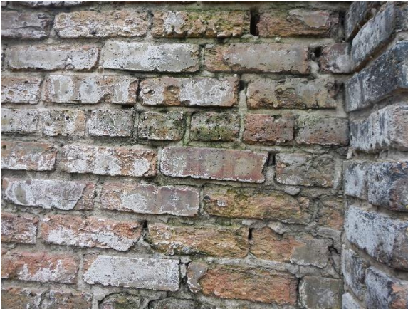
Photo 31. Typical brick deterioration at the west elevation included: cracked brick, spalled brick, organic growth, and efflorescence staining.
