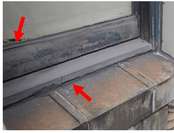
Photo 36. Failed sealant around window frame elements.
