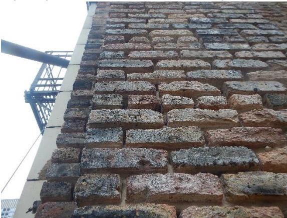
Photo 33. Severely eroded mortar joints observed at the west elevation.
