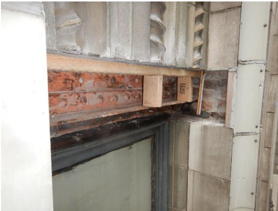
Photo 43. Exploratory opening #2 at 5th floor spandrel, north elevation. Moderate surface corrosion observed at bottom flange of steel built-up spandrel.
