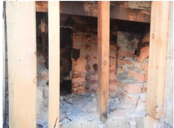
Photo 44. Exploratory opening at 8th floor column, north elevation. Minor surface corrosion and rust staining observed on steel.
