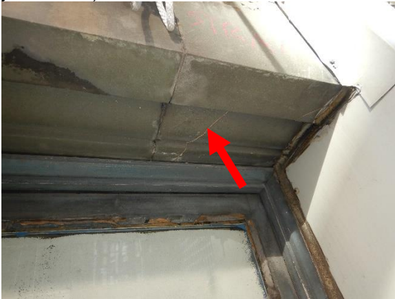
Photo 15. Underside crack at terra cotta window head unit (red arrow).
