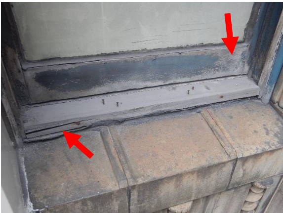
Photo 35. Deteriorated wooden window frame elements.
