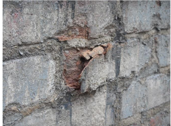
Photo 32. Surface spall observed, indicating excessive moisture within masonry wall.
