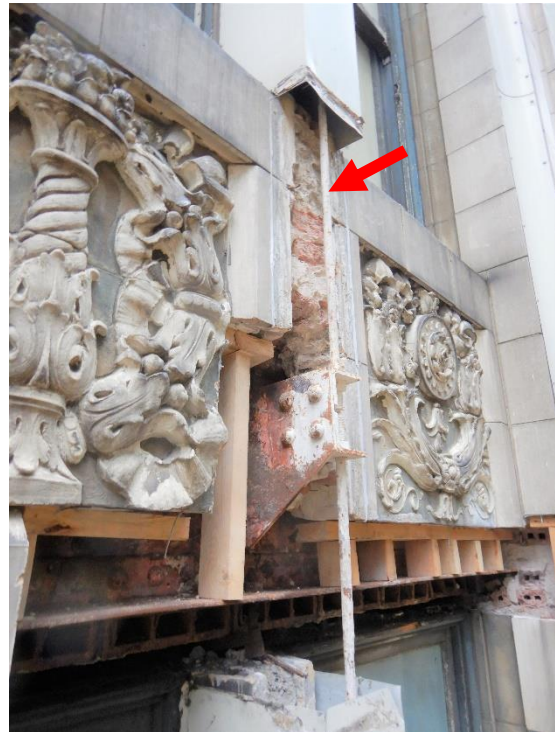
Photo 40. Exploratory opening at 4th floor mullion, north elevation (hanger rod noted in red).
