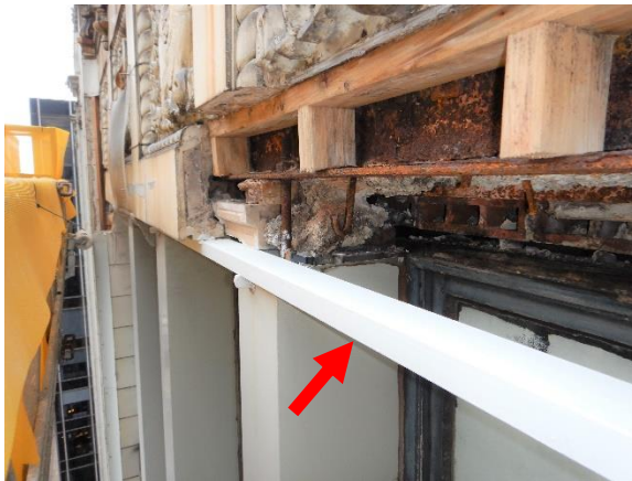
Photo 47. Exploratory opening #1 at attic floor window headers, north elevation (painted metal channel noted by red arrow).
