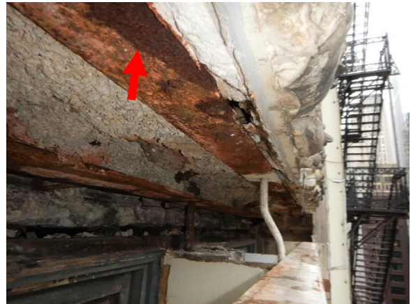
Photo 46. Corroded steel shelf angle with water staining (red arrow), evidence of water infiltration.
