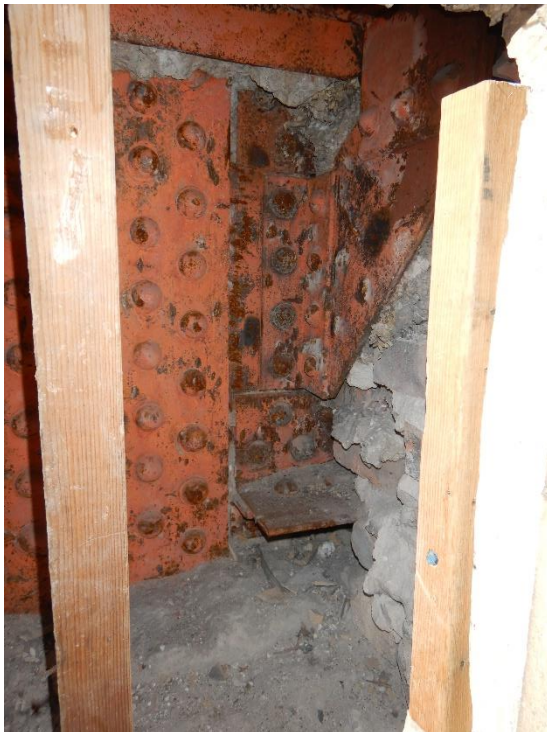
Photo 39. Steel column and connection in good to fair condition with minor surface corrosion.
