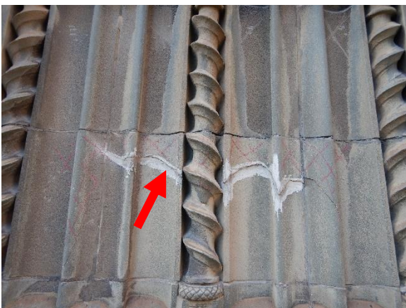
Photo 17. Large spall observed on terra cotta spandrel units.
