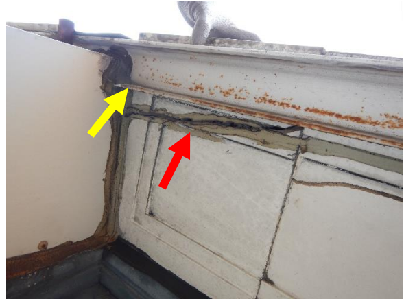
Photo 14. Previous underside crack repair (red arrow) in poor condition at terra cotta window head unit (metal channel noted by yellow arrow).
