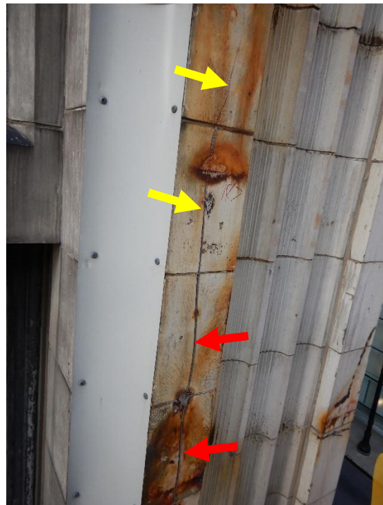
Photo 26. Previous crack repair in poor condition (red arrow) with new crack (yellow arrow).
