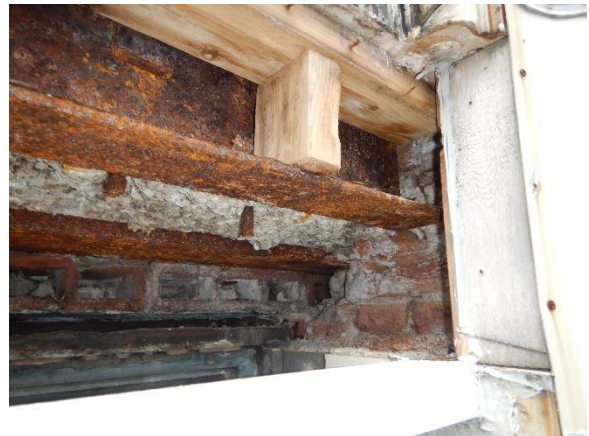
Photo 48. Extensive surface corrosion and rust jacking observed on existing steel elements.
