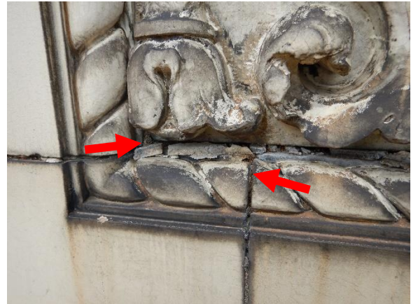
Photo 28. Cracked and deteriorated mortar joint with organic growth (red arrow).
