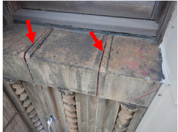
Photo 20. Typical open skyward facing joints observed at most window sill terra cotta units.
