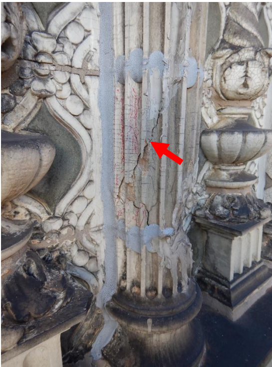
Photo 7. New cracks and loose material observed at terra cotta units.
