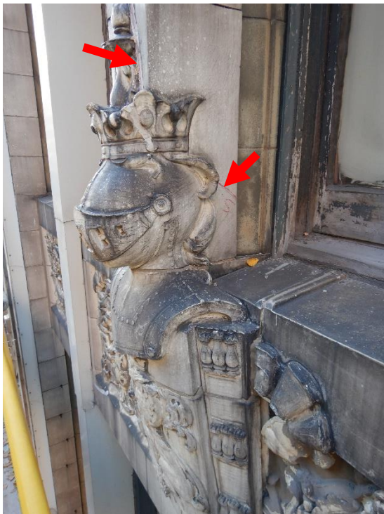
Photo 11. Ornamental spandrel at 4th floor (new cracks noted by red arrows).
