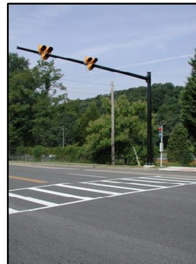
High Intensity Activated Crosswalk Signal in Alexandria, Virginia Source: City of Alexandria (2015)
