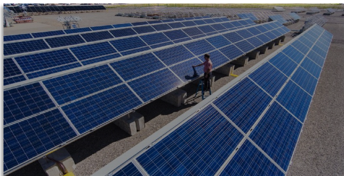
PHOTO 1. EXAMPLE GROUND-MOUNTED SOLAR ARRAY. (Source: www.energy.gov/articles/getting-most-out-solar-panels )
