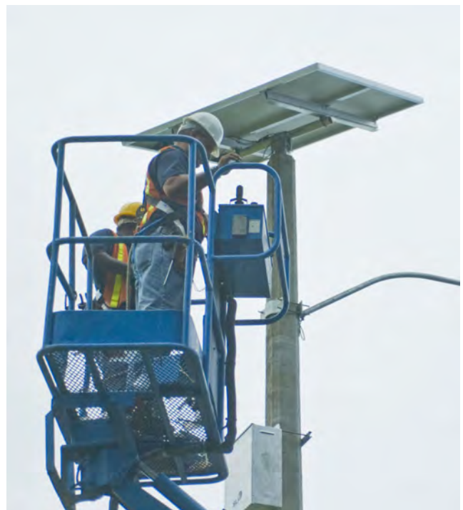
Solar powered street lights Image courtesy of: United States Army
