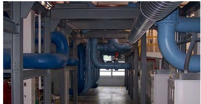
Effluent heat exchange facility at the main base Image courtesy of: Trane U.S., Inc.
