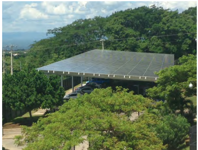
Carport canopy solar PV system
