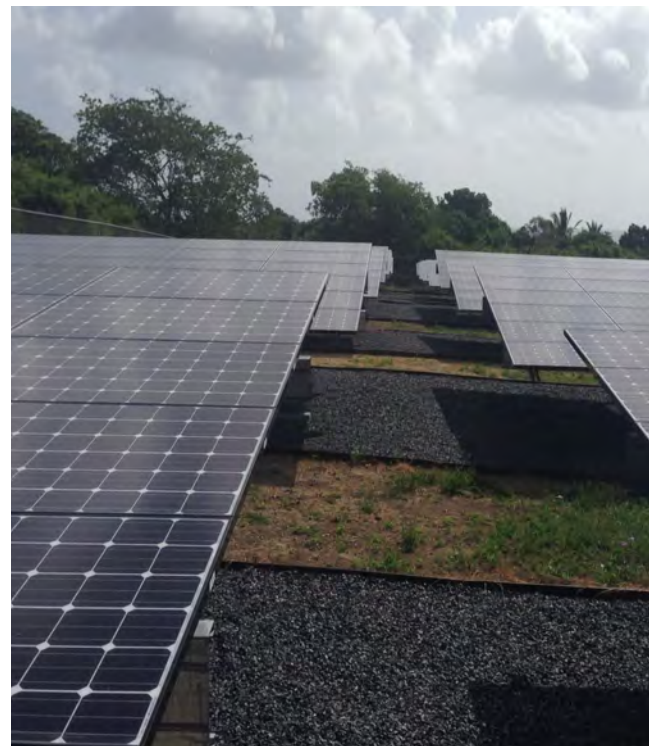
The Almeric L. Christian Federal Building's 462 kW solar array
