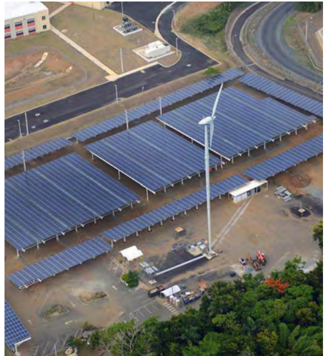
Parking lot PV canopy and neighboring wind turbine Image courtesy of: United States Army
