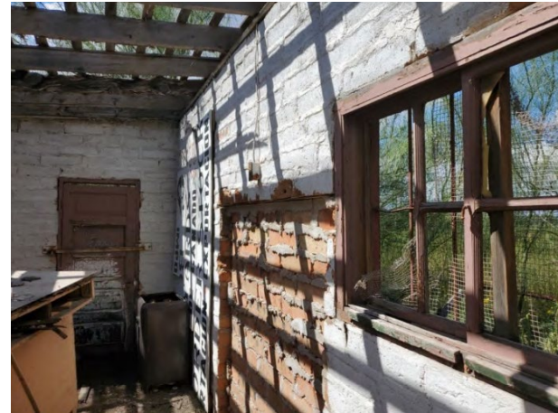
Interior of Cattle Operation Building
