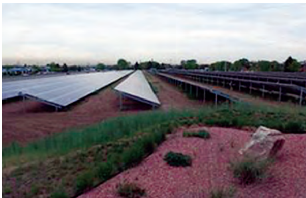
Denver Federal Solar Park Denver, CO
