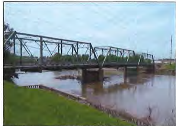
The $2.6 million SW 5 th Street (Jackson) Multi-Use Trail Bridge Rehabilitation project is being made possible with $1,050,000 of private donations and a $500,000 State Grant.
