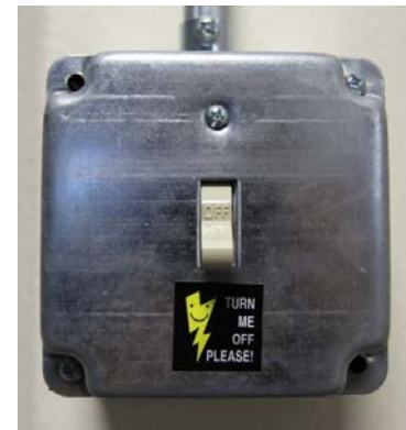
Figure 24 Image of Building 1219, Open Office Manual Switch and Reminder Sticker
