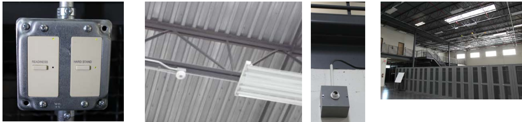
Figure 30 Images of Building 9447, High Bay Module Daylighting and Lighting Control Features
