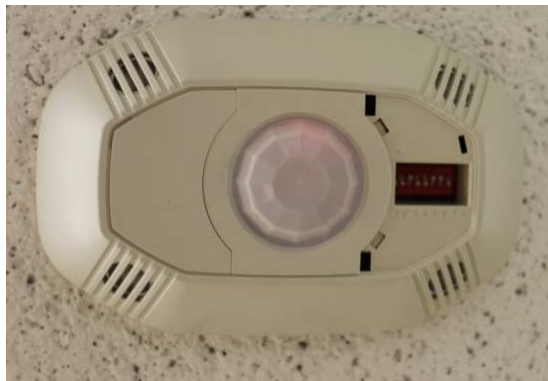
Figure 23 Image of Building 1219, Open Office, Ceiling-Mounted Occupancy Sensor
