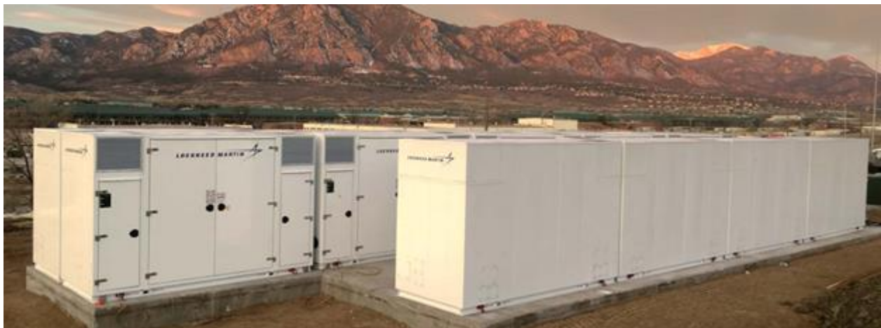
Image: Ft. Carson - Peak Shaving Microgrid
