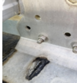
Bolts missing because of transverse slip
