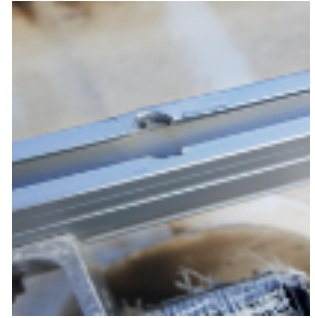
Top-down clamp with T-bolt torn out of rail
