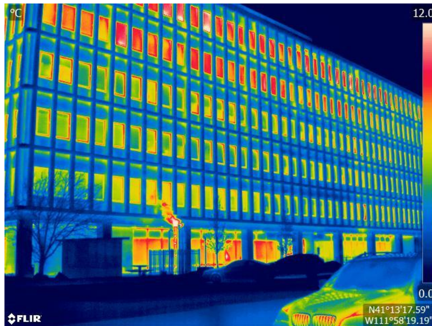
Figure 13. North facing side of the Hansen Building in Ogden, UT. Infrared image at night during the winter. The top two floors have no applied film (warmer surface temperature indicate more heat loss). The lower floors have the low-e applied film installed (less heat loss).
