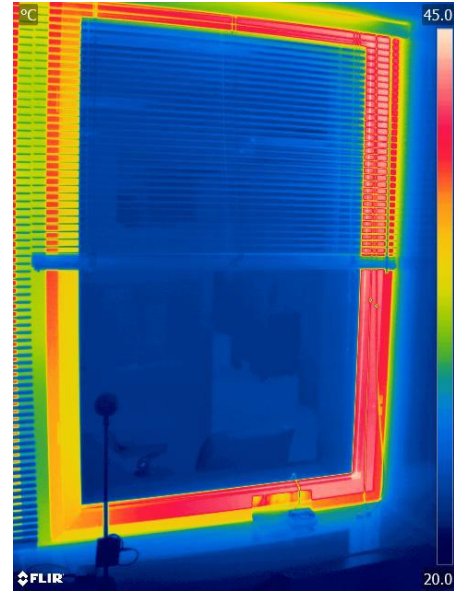
Left NORTH façade in WINTER, Right SOUTH façade in SUMMER both low-e film (different temperature scales)
