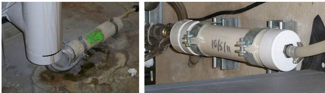
Figure 11. In-line Condensate Neutralizer Kits Installed on Condensing Boilers
