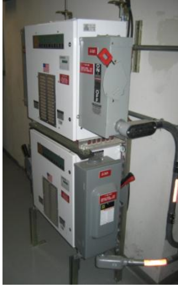
Figure 13. Two inverters and disconnects
