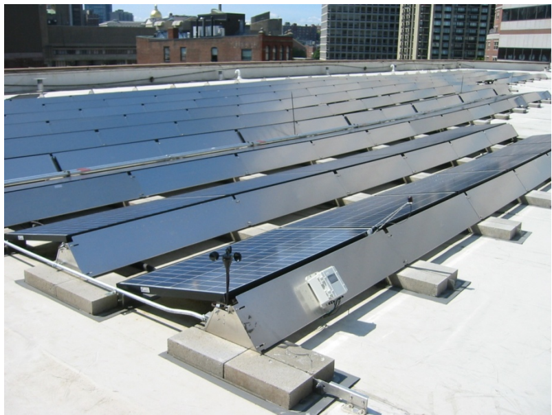
Figure 11. O'Neill Federal Building PV-T system facing approximately south
