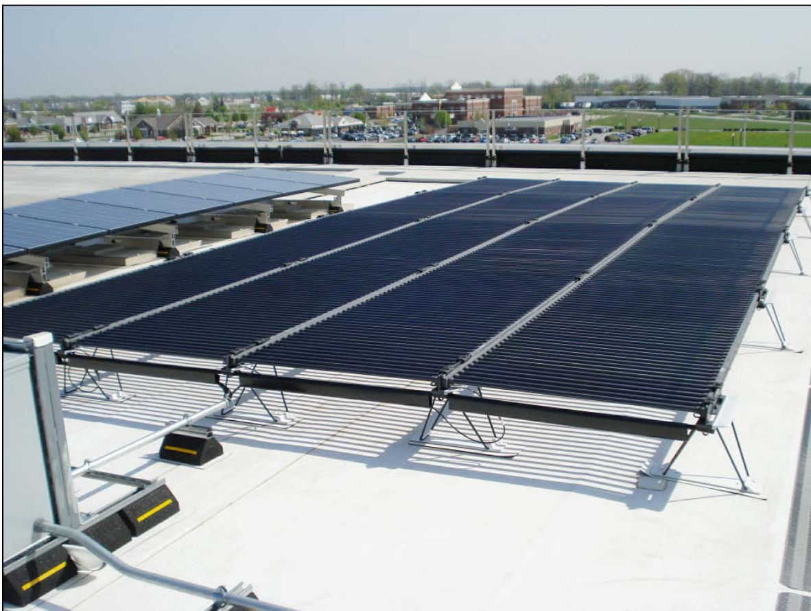
Figure 4: Thin-film CIGS Cylindrical PV Array, Laboratory PV systems, Bean Federal Center
