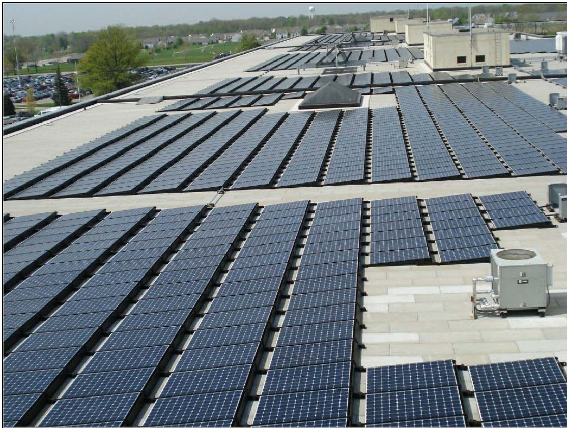
Figure 1: Section of the High Efficiency Crystalline (Main) PV system at the Bean Federal Center
