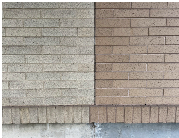
Expansion joint between original construction and 1981 addition showing difference in brick color, 2021.
