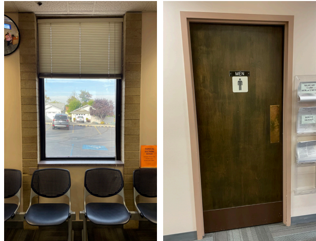
Typical interior window treatment with exposed masonry flanking window (left); typical original wood door (right), 2021.
