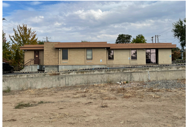
West elevation with parking lot in the foreground, elevator addition does not have the metal panel fascia, 2021.
