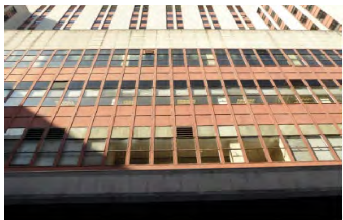
Photo: Appraisers Building example of curtain wall repairs needed.
