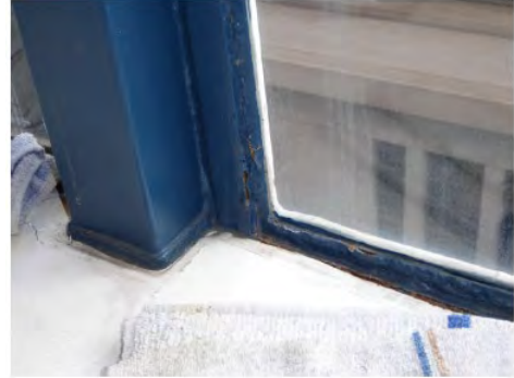
Photo: Appraisers Building example of curtain wall repairs needed.
