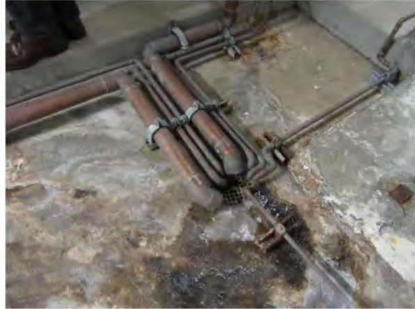
Photo: Appraisers Building sub-basement water intrusion needing repair.
