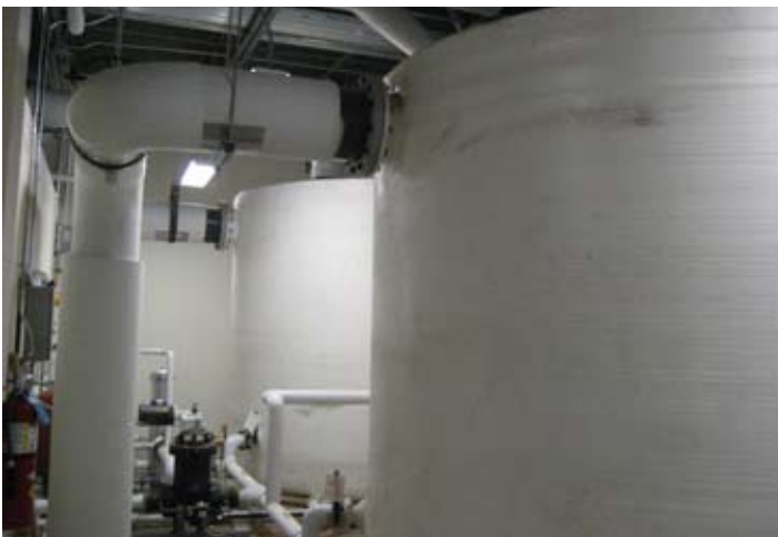
Rainwater is stored and reused for landscape irrigation
