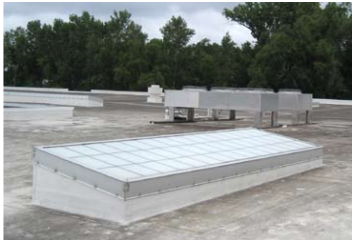
Skylights provide daylight where needed
