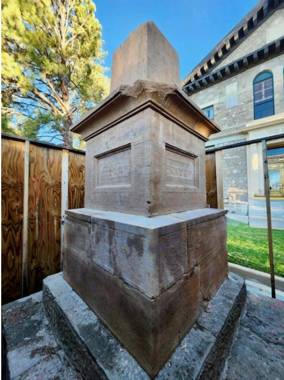
Figure 2, image showing damages and deterioration.
