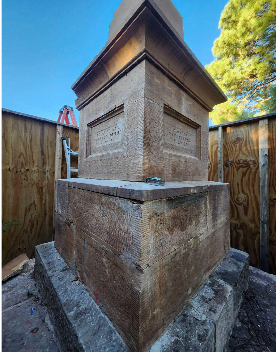
Figure 6, Photograph of two sides of the monument, reflecting its current general appearance. Images of condition issues can be found in Appendix C. Note that not all condition issues are captured in this image. See Appendix C for detailed images of cracks, delaminating, and broken sections of sandstone.
