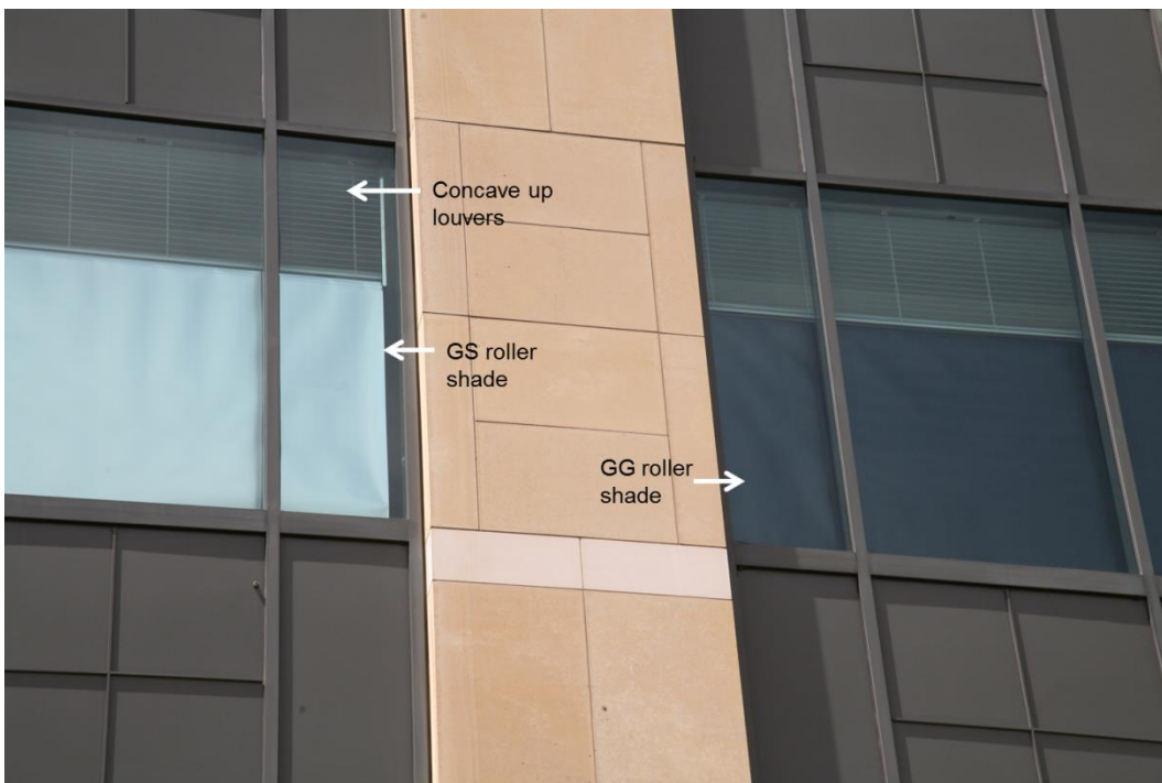
Figure 7. Outdoor view of the Oakland Federal Building with automated upper louvers and lower manually operated GS (bright white) or GG (dark gray) shades on the southeast facade.
