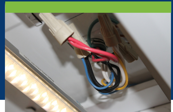
Ballast is disconnected. Sockets are wired directly to the branch circuit and provide line voltage. Photo credit Michael Myer, PNNL
