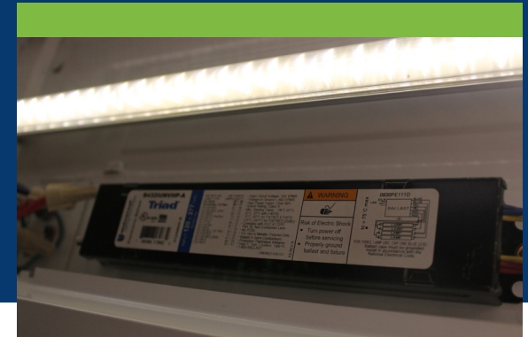
Type A TLED installed in the luminaire using the existing ballast. Photo credit Michael Myer, PNNL
