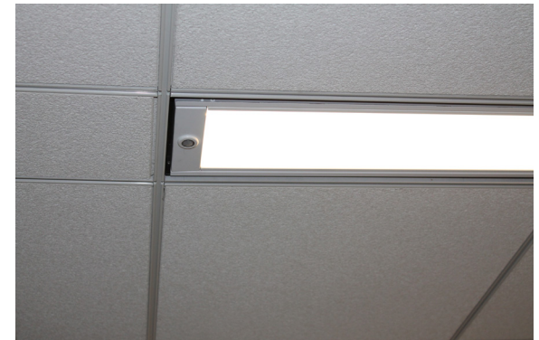
Troffer with embedded occupancy sensor Photo credit Michael Myer, PNNL
