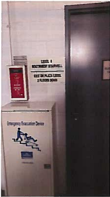
Typical floor sign, evacuation chair and emergency phone
