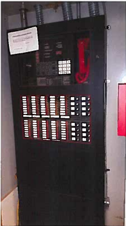
No grounds noted on the Fire Alarm Control Panel
