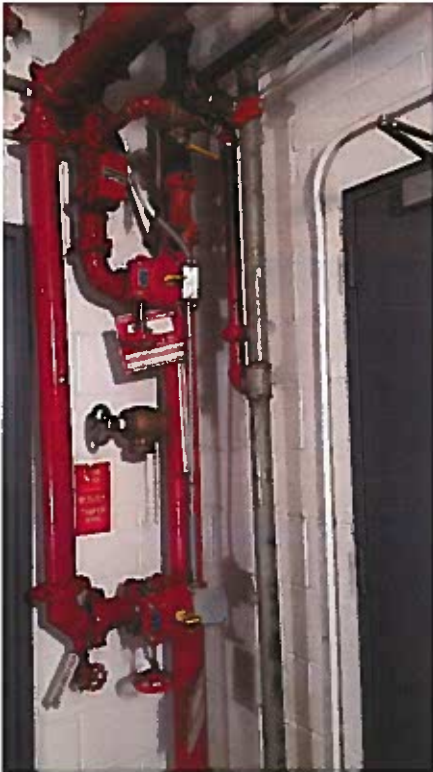
Typical floor control valve for sprinkler system
