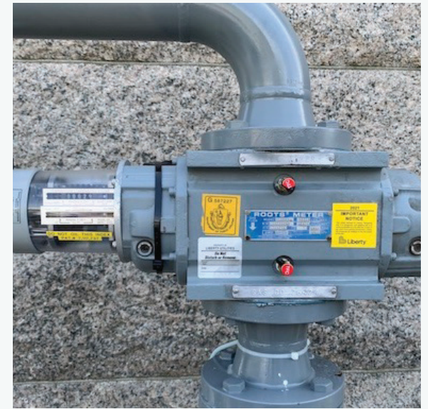
Non-Invasive Gas Submeter Photo credit Vata Verks
