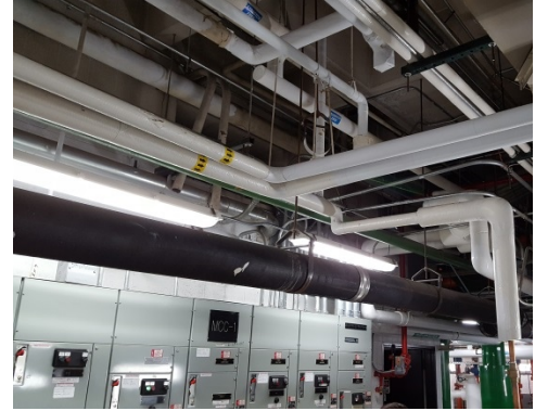
Figure 9 – DHW Supply and Return Lines
