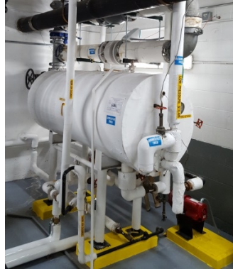
Figure 8 – DHW Storage Tank
