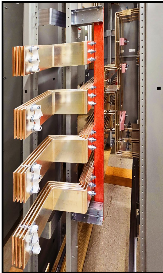
Figure 18: Building 48 Denver Federal Center Electrical Denver, CO
