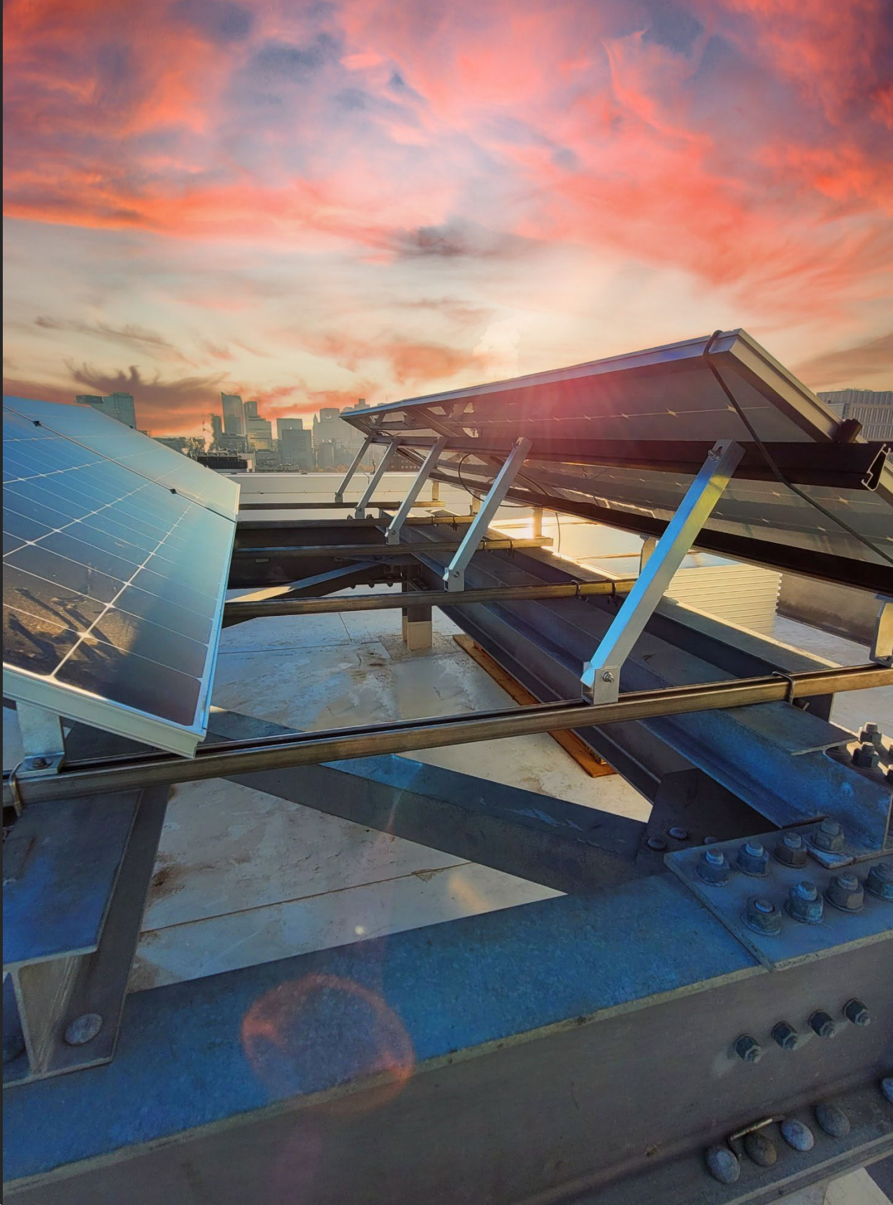
Figure 17: Solar on U.S. Department of Transportation Volpe Center Cambridge, MA
